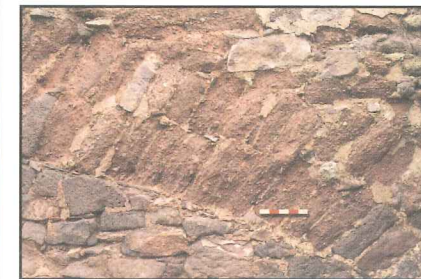
Sloping blocks of red Heavitree stone (mixed with some purple and grey volcanic trap) in the 15th-century relieving arch below the church tower. The photograph shows the signs of heavy weathering typical of this material.
