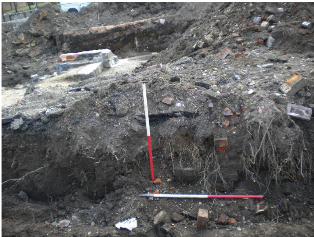
Plate 7. Brick return wall running south from west end of context 5 seen in temporary trench section below tarmac and rubble in-fill deposits. From the north.
