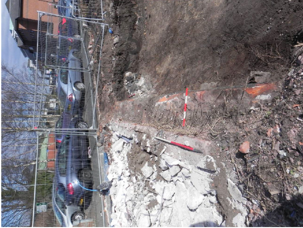
Plate 4. Wall foundations exposed in northern trench section showing demolished 1980s concrete slab to the north with line of modern brick foundations directly in front, context 3, and wall foundations, contexts 4 and 5, running parallel. From the west.
