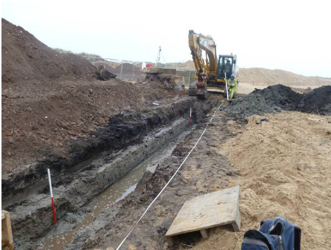
Plate 10. Along east-facing trench profile just prior to section across line of ramp to old sea defences. From the north.
