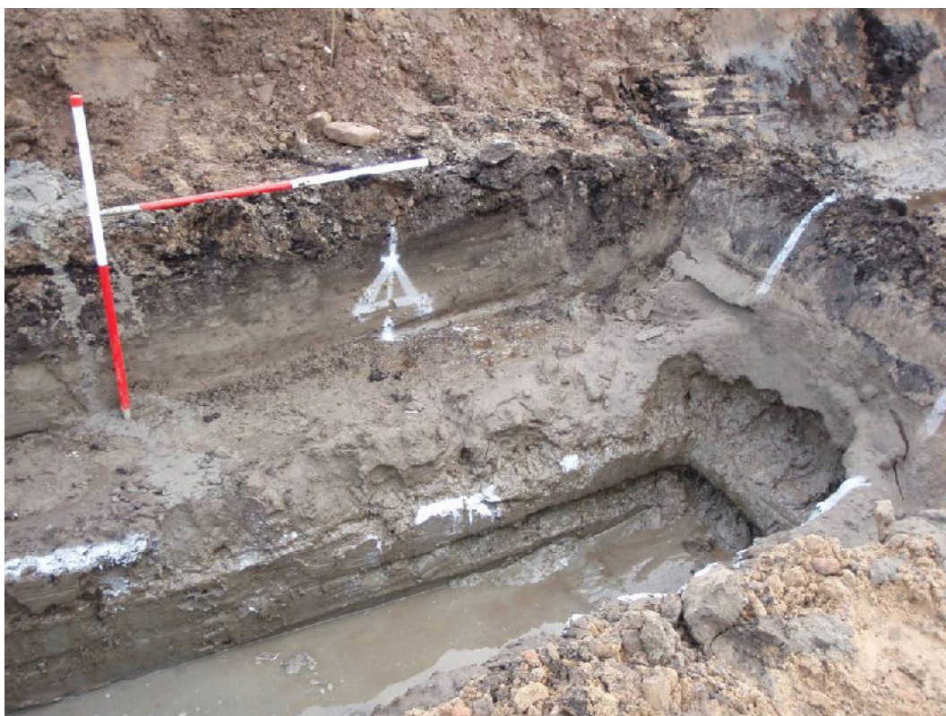
Plate 6. West facing trench profile at c. 36 m showing rising clay and sand layers below thinner layer of peat. Water seepage at base of trench caused by a layer of blue sand below thinning layer of clay. From the west.
