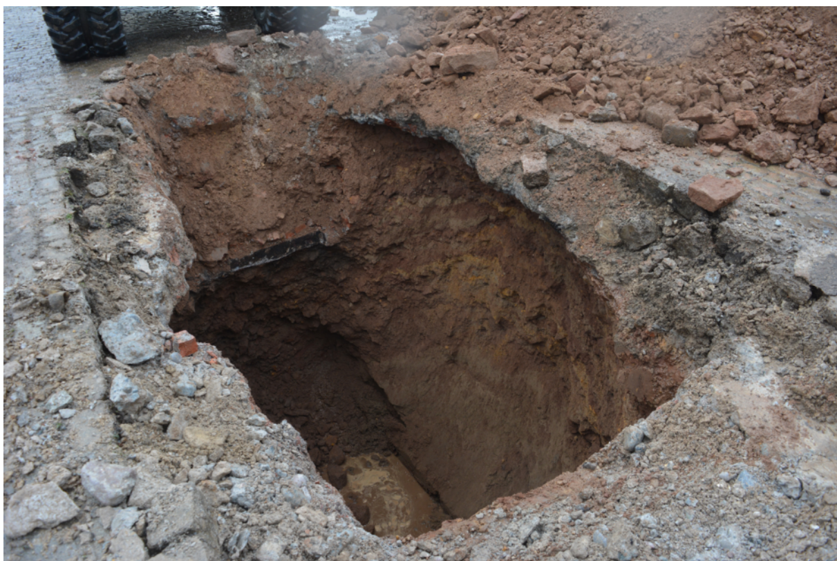
Plate 11. TT306. Brick lined culvert exposed in southern edge of trench. View looking south-west.
