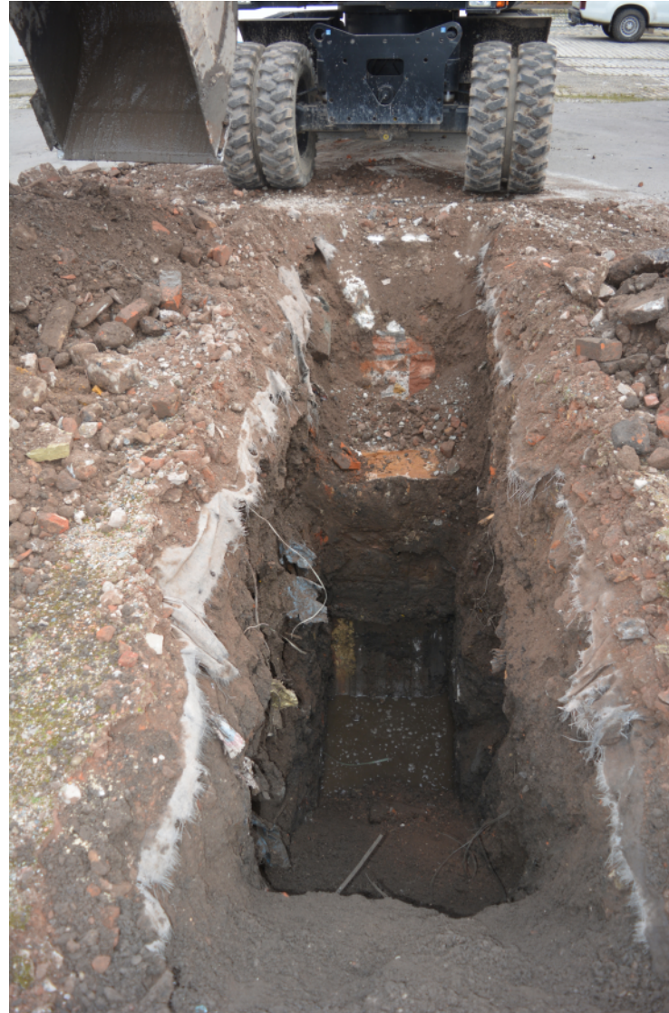
Plate 2. TT301/305. Retaining wall to Princes Dock after further excavation. View looking east. A scale could not be inserted.
