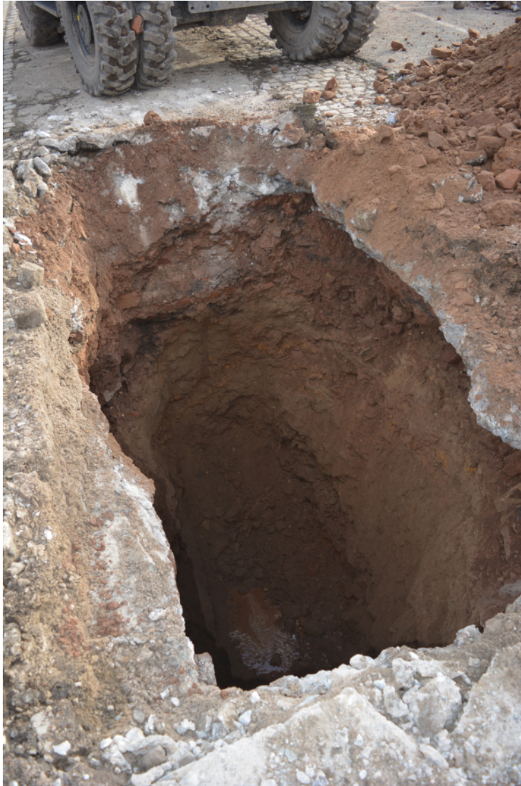
Plate 8. TT304. Brick lined culvert exposed in southern edge of trench. View looking south-west.
