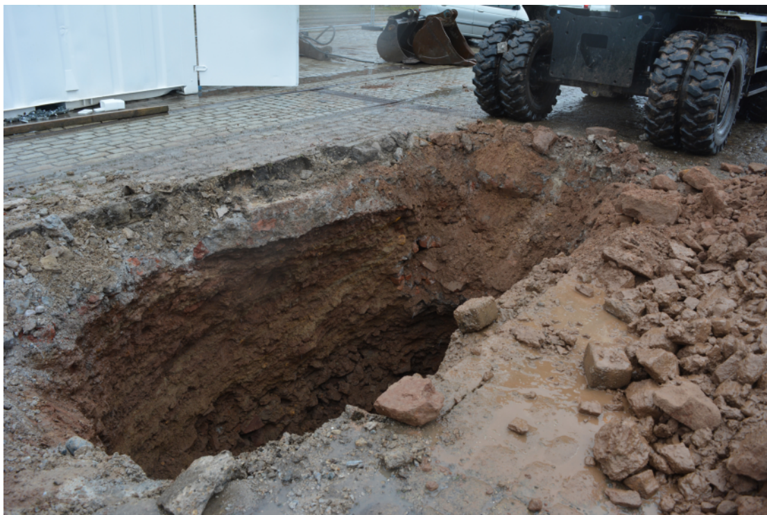
Plate 10. TT306. Brick lined culvert exposed in southern edge of trench. View looking south-east.
