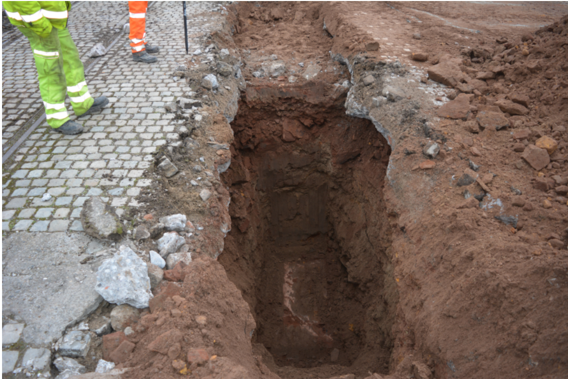
Plate 7. TT304. Large red sandstone block exposed at base of trench. View looking south.
