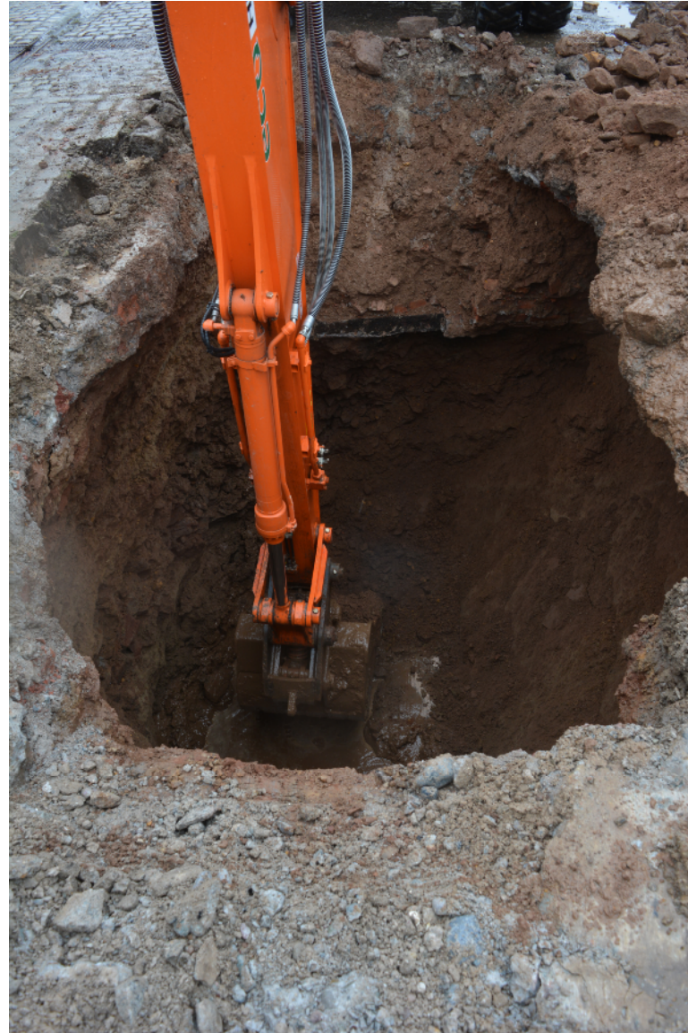
Plate 9. TT306. Red sandstone obstruction in base of trench. The block is set to the immediate right of the excavator bucket. View looking south.
