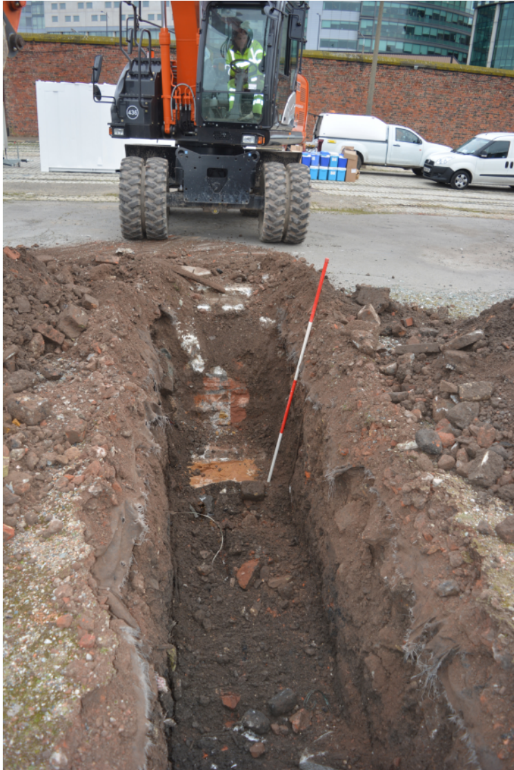
Plate 1. TT301/305. Retaining wall to Princes Dock as first exposed. View looking east. Scale = 2 m.
