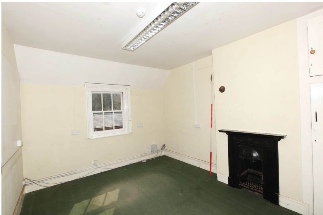
Illus. 10. The interior from the north of the chamber above the main entrance to the courtyard showing its ostensibly original coal grate on the right.
