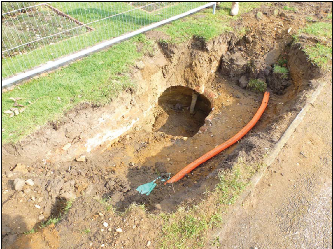
Plate 4. Well shaft and brick dome revealed in service trench, camera facing NE
