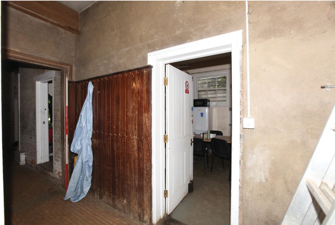
Illus. 11. The corridor of the western range (15) viewed from the north-east and showing the doors of the northern and southern offices (14 and 13 to right and left respectively). The wainscot and imitation ashlar matches that of the stables but these rooms were heated and probably used by the stablemen.
