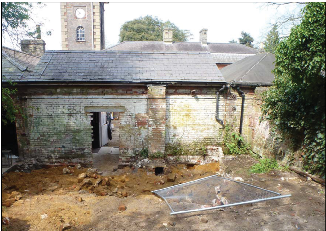
Plate 14. General view of area of boiler house 2, camera facing N. The flue and chimney breast can be seen in the centre of the photograph
