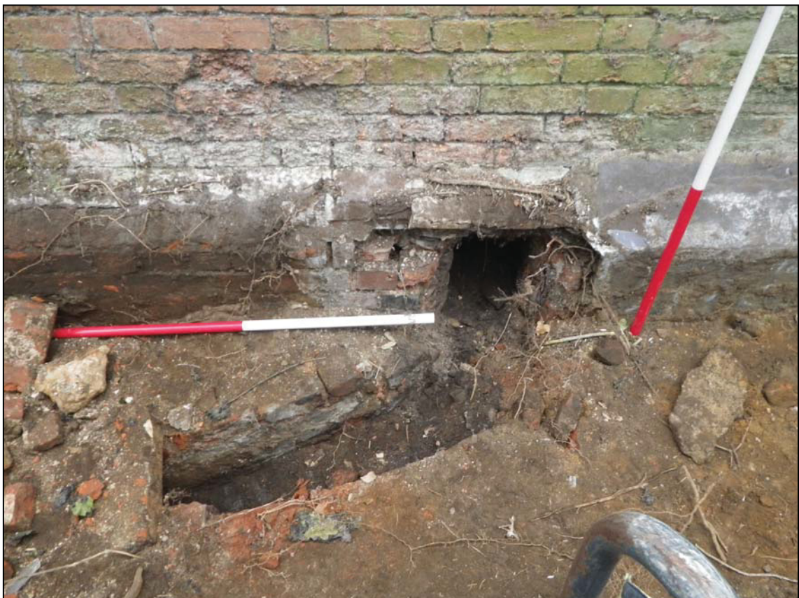
Plate 10. Flue from boiler house to west wall of stable block, camera facing E
