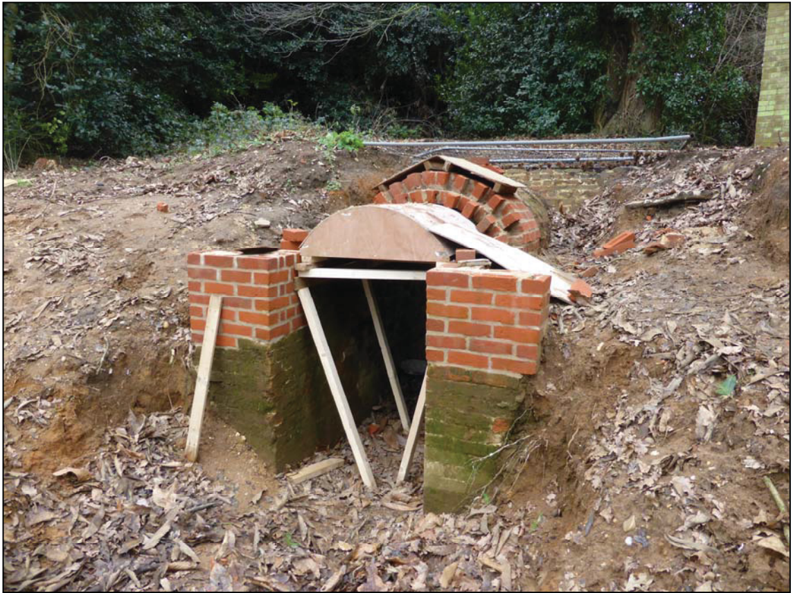
Plate 21. Restored brickwork around the entrance to the icehouse (Jan 15), camera facing SE
