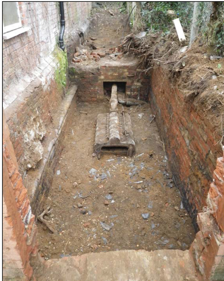
Plate 6. General view of Boiler House 1 through the newly opened access, camera facing S
