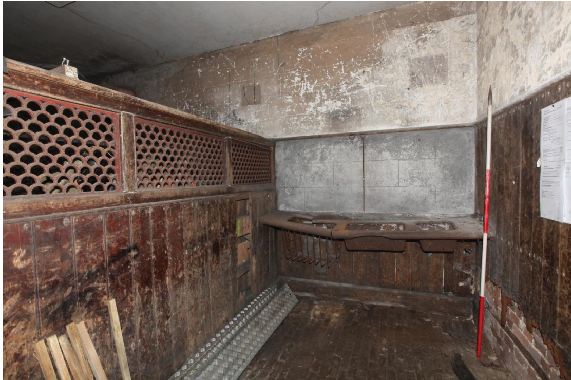
Illus. 5. The intact eastern stall of the triple stable (3) showing what appears to be its original decor and fittings with the north-eastern corner of the stable block to the right. The plaster above the wainscot is lined in imitation of ashlar and the decorative pierced iron grill of the internal stall division on the left is painted red. Note the pressed iron trough incorporating twin compartments with a hay basket on the left.
