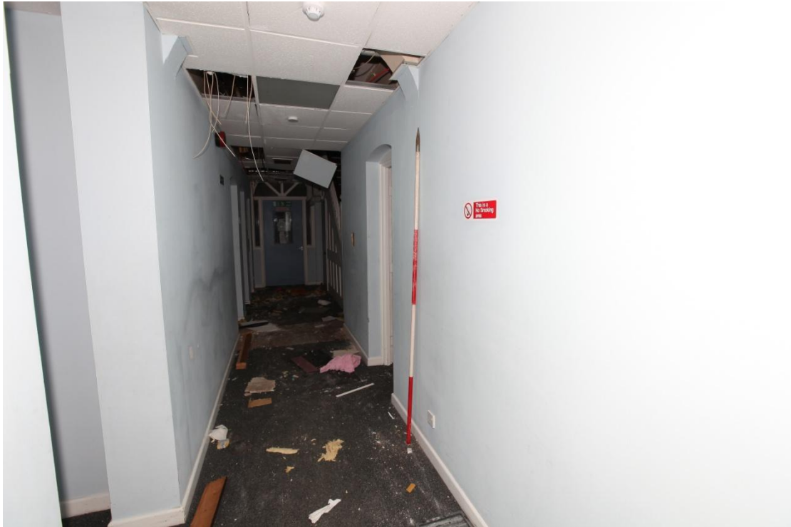
Illus. 9. The southern section of the axial ground-floor corridor in the original structure (A) viewed from the south and showing the late-20 th century cladding which dominates the interior. This corridor links the entrance lobby shown in illus. A2.8 above to the staircase in A2.10 . Note the lower section of a tall original brick arch immediately above the scale rod which indicates the original height of the corridor before the insertion of the present ceiling.
