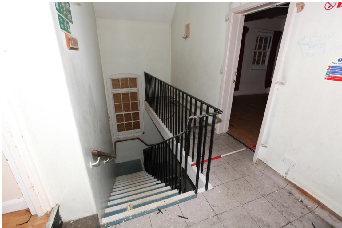
Illus. 16. The first floor landing of the iron staircase at the western end of the early-20th century extension (B) as viewed from the north. This stair was probably added when the building was extended in the mid-20 th century. The internal division between structures B on the left and C1 on the right is heavily disguised.
