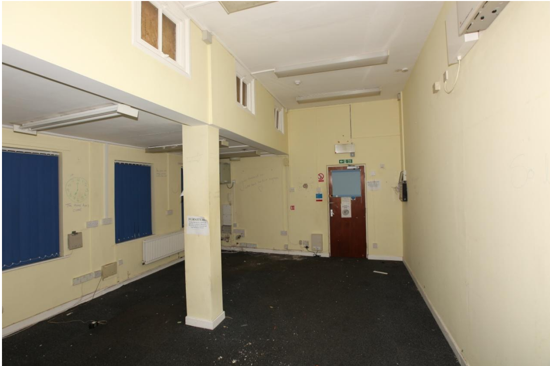
Illus. 13. The high-ceilinged room to the east of the axial corridor in the single-storied section of the original structure (A), viewed from the north and showing the eastern facade on the left and the door to the entrance lobby on the right.
