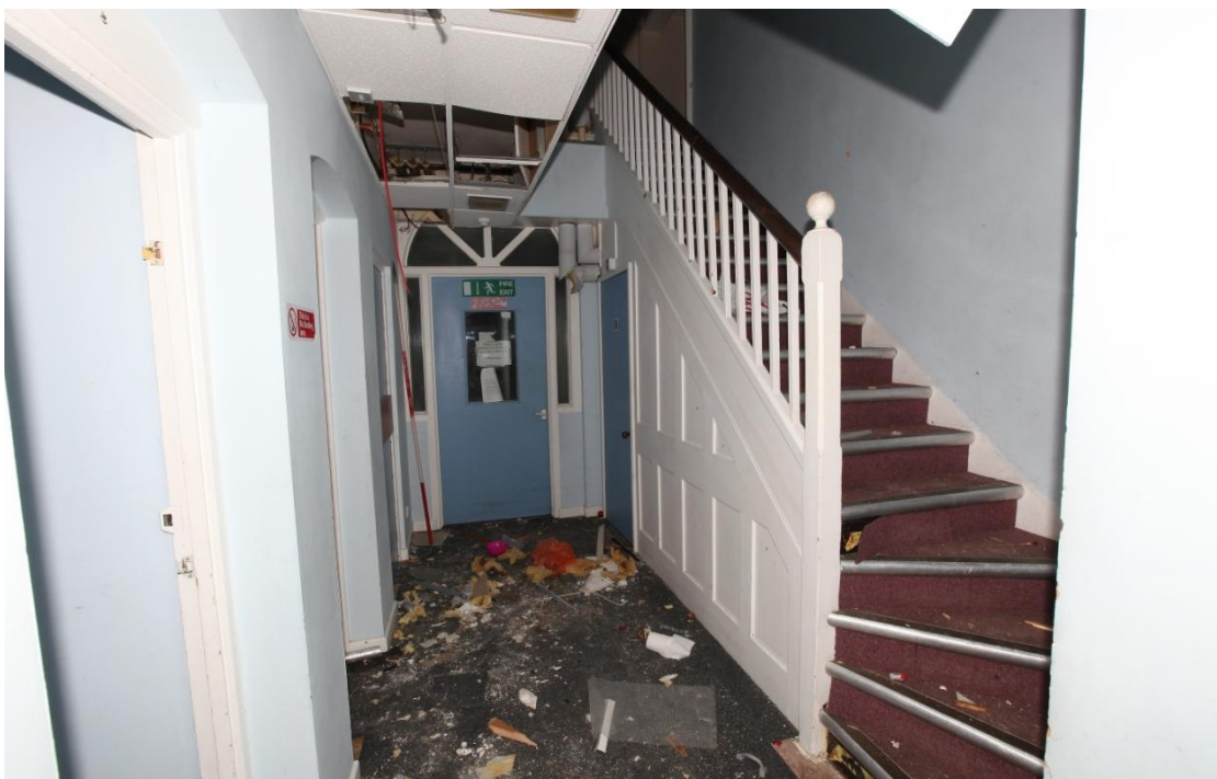
Illus. 10. The possibly original staircase at the northern end of the southern section of corridor in structure A, seen from the south. This rises to the southern end of the two-storied section of the building, and the door beneath its balustrade opens onto the cellar steps. The arched fire door leads to the northern section of the axial corridor.
