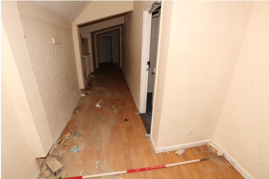
Illus. 17. The rear (northern) first-floor corridor of the early-20th century extension (B) viewed from the landing of the iron staircase to the west. Original painted brickwork is exposed on the left but the partitions of the rooms and kitchens on the right all appear to be later insertions.
