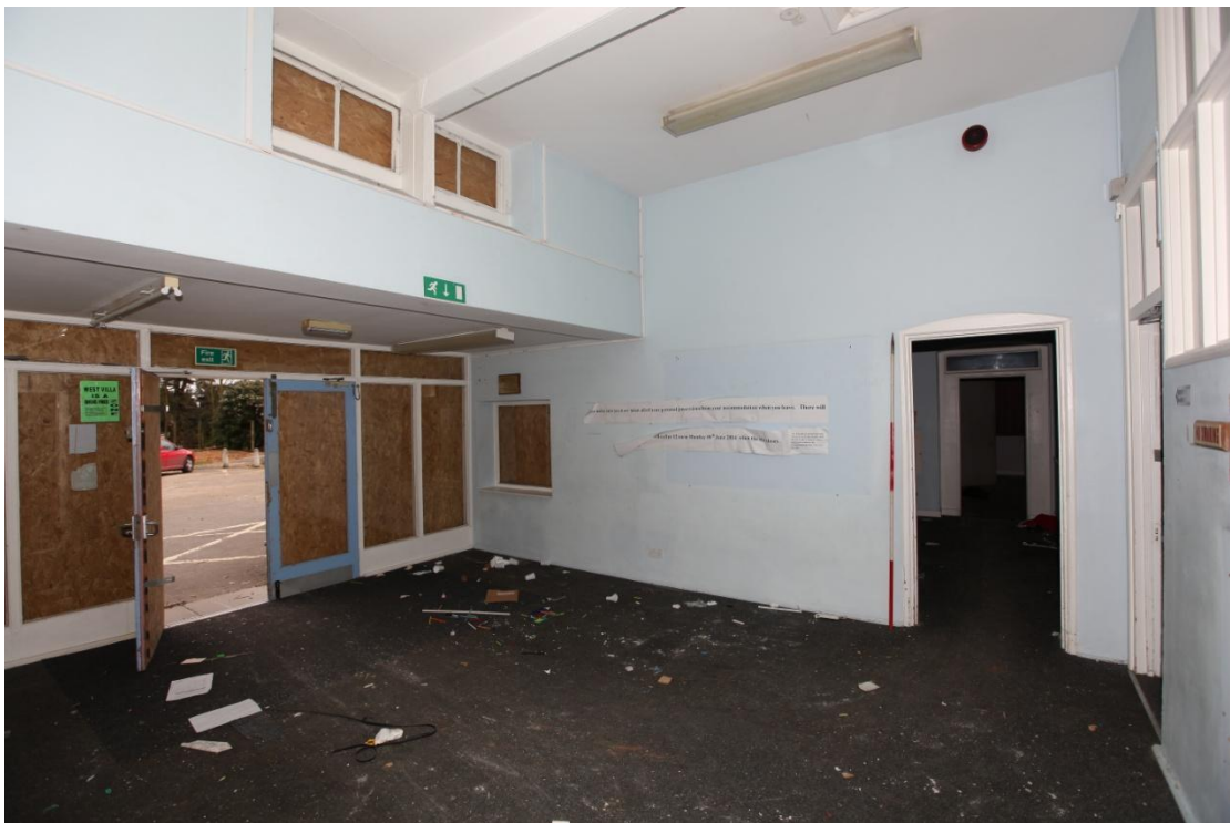
Illus. 8. The interior from the north of the modern entrance lobby at the southern end of the original structure (A). The lower section of its eastern wall to the left has been removed where it adjoins the flat-roofed late-20 th century 'porch', which retains a brass plaque commemorating the 'reopening' of West Villa in 1995 (above the hatch in the centre of this image). The door to the right opens into the early-20th century extension (B) and marks the southern gable of the late-19 th century building.
