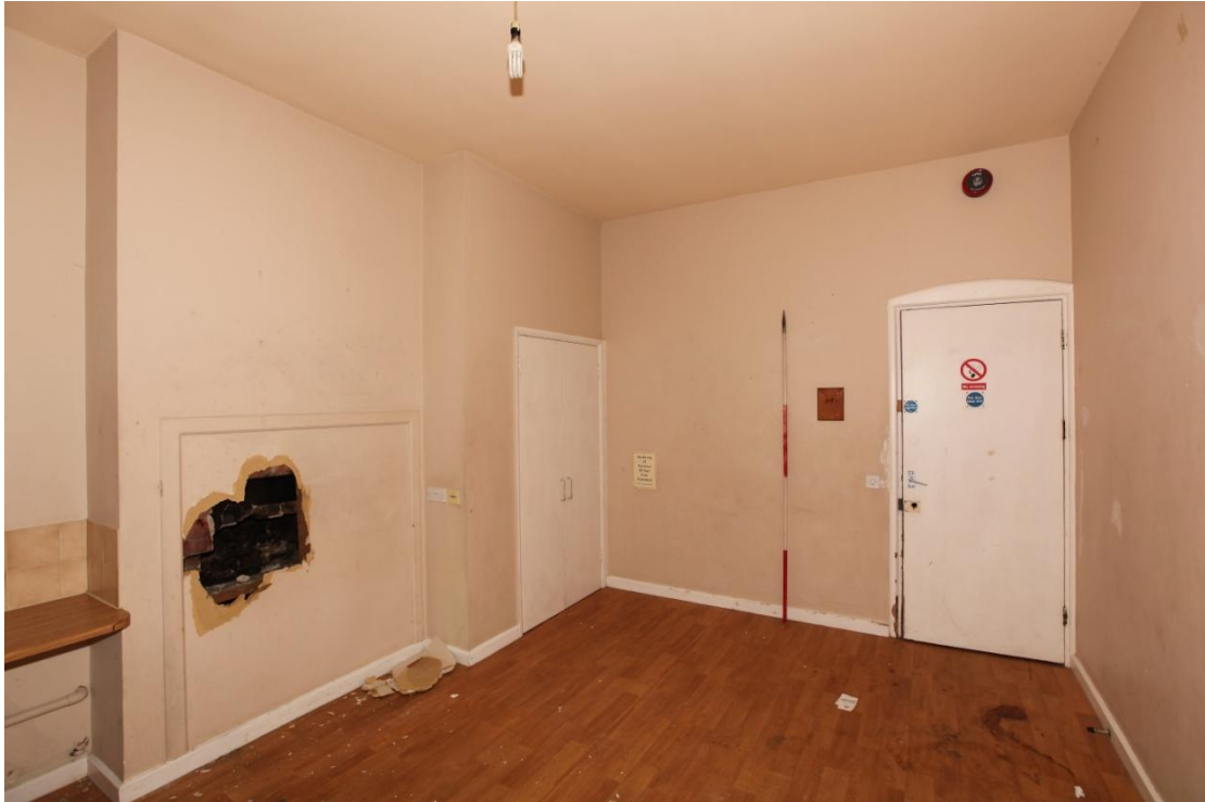
Illus. 11. The central ground-floor room to the rear (west) of the axial corridor in the two-storied northern half of the original structure (A). The door to the right opens into the corridor and a blocked fireplace is visible to the left. The latter was served by the missing chimney depicted in figure 2a. The late-20 th century cladding to the floor, wall and ceiling of this room is replicated throughout the building, effectively concealing its original fabric.
