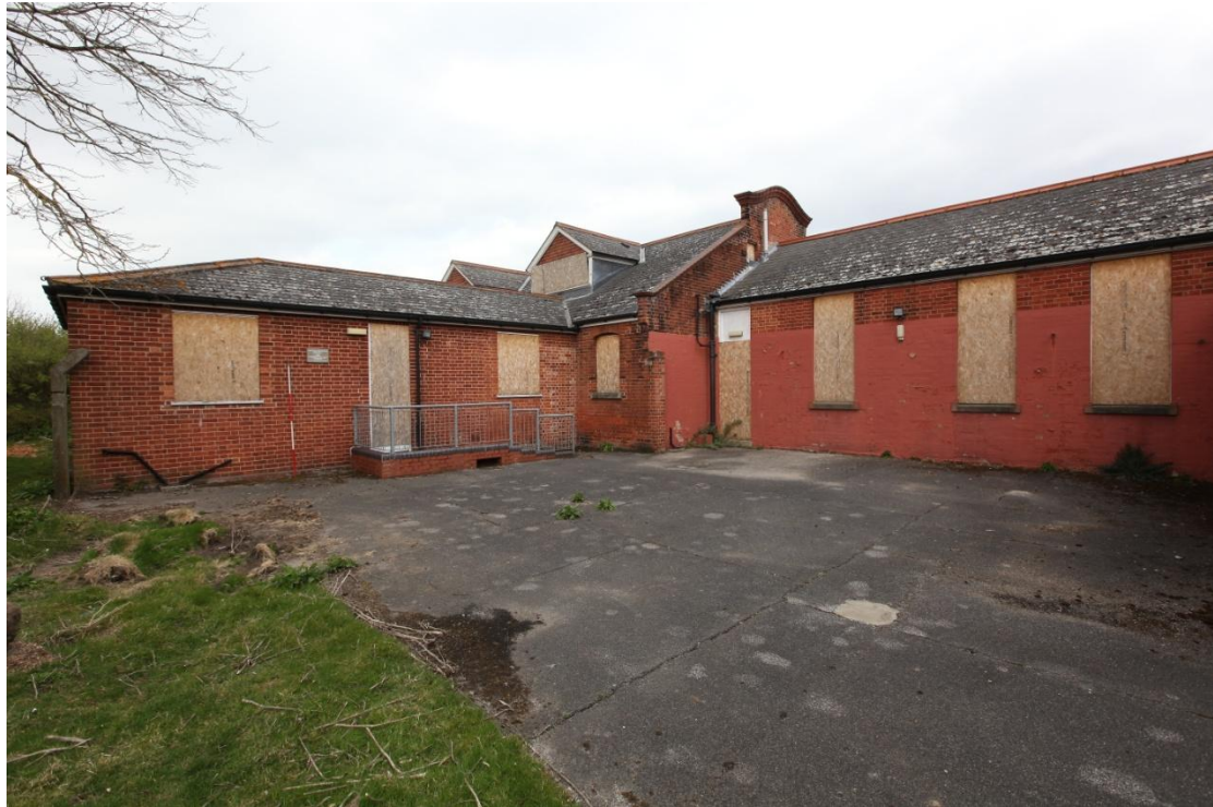
Illus. 5. The original structure (A) from the south-west with the mid-20 th century extension on the left (C3). The wall of the single-storied range on the right has been rebuilt and it was formerly of the same width as the two-storied range, as indicated by the scar of the original roof on the latter's gable. Note the loss of the chimney depicted in figure 2 which belonged to the fireplace in illus. A2.11.
