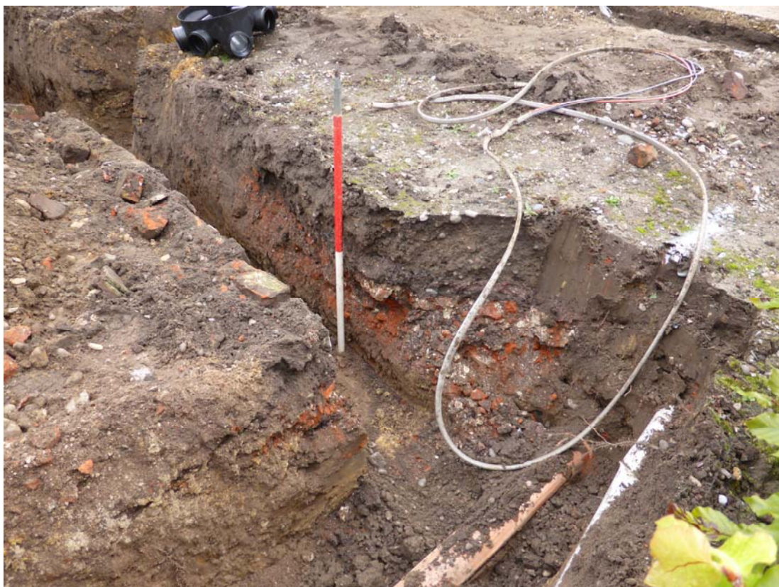
Plate 1. View of the drain run showing thickness of disturbed topsoil over brick rubble and hard-core (behind 1m ranging rod). Some sand natural apparent in base of trench to right of ranging rod. The drain to the right of the frame is within an existing service trench.
