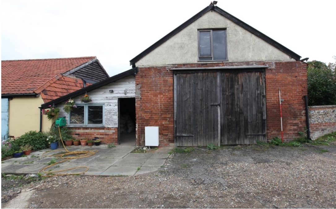
Illus. 3. The southern exterior of Barn 1 showing the original double doors of the mid-19 th century vehicle shed (1) respected by closers (quarter bricks) in both brick jambs. These doors are interrupted internally by the secondary ceiling, and the gable window dates from the alterations of circa 1980. The lean-to shed adjoining on the left (1a) and the yellow-painted workshop beyond (1b) were built on the site of the 19 th century sheds depicted on the Ordnance Survey of 1958 (figure 6).
