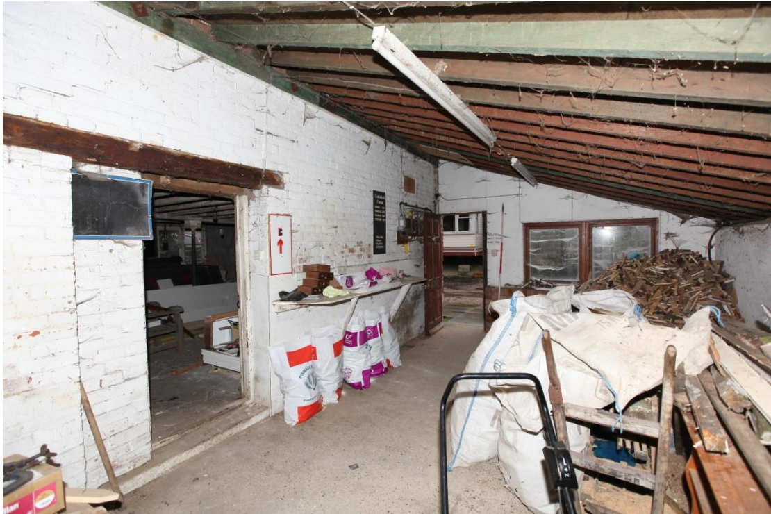
Illus. 11. The interior from the north of the 20 th century lean-to shed (1a) showing the original side door of the vehicle shed (1) on the left. This doorway is respected by closers in the brickwork but has been reduced in width by inserting a new brick pier to its left. The right-hand (western) wall of this shed consists of cement block-work.
