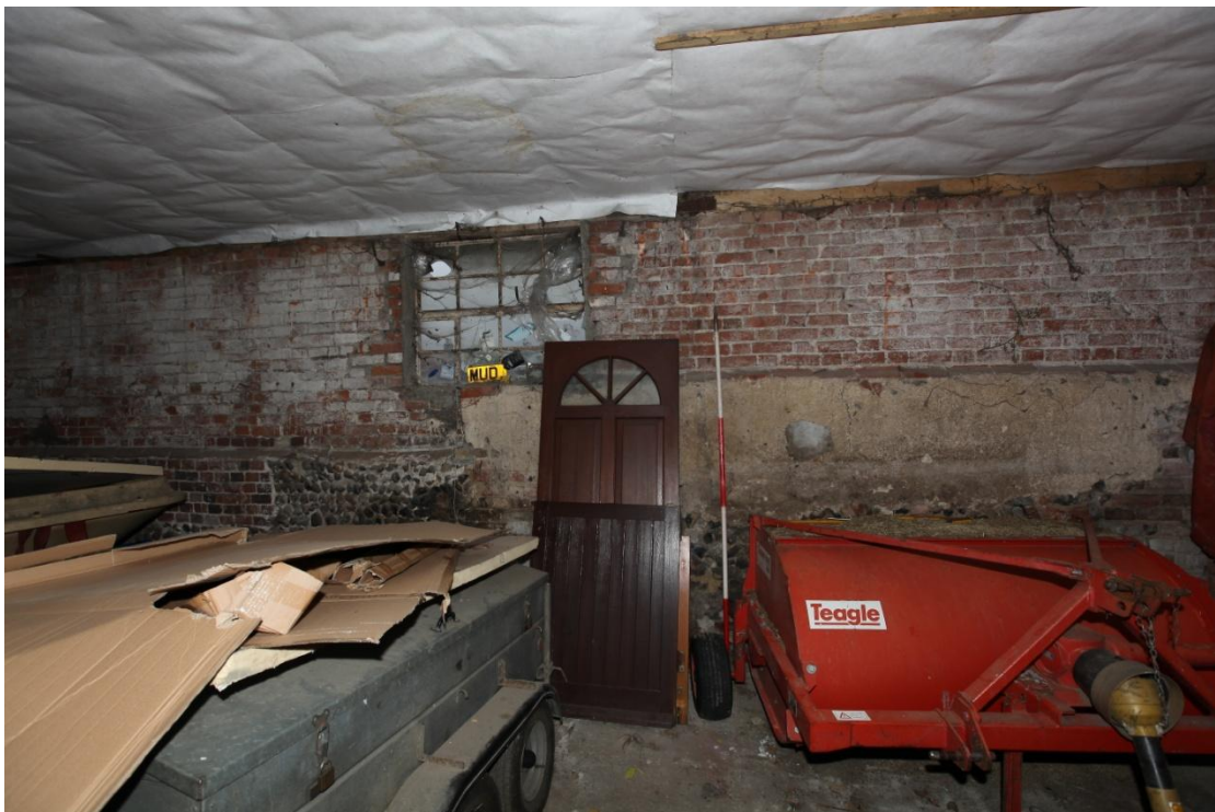
Illus. 12. A detail of the original 19 th century northern internal wall of the workshop (1b) showing its secondary window. The rest of the shed consists of cement block-work and represents a 20 th century reconstruction on the site of the 19 th century sheds to which this wall belonged.
