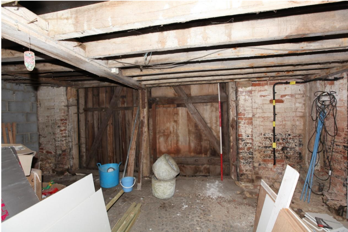
Illus. 9. The original entrance doors in the southern gable of the vehicle shed (1) now partly blocked by the later ceiling and its central supporting post.
