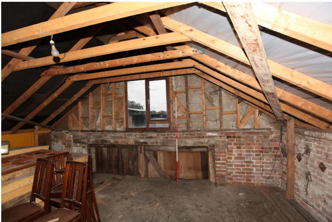
Illus. 10. The top of the original entrance doors in the southern gable of the vehicle shed (1) as seen from the loft. The window and studwork above the original brickwork are part of the alterations of circa 1980, as is the entire roof structure.
