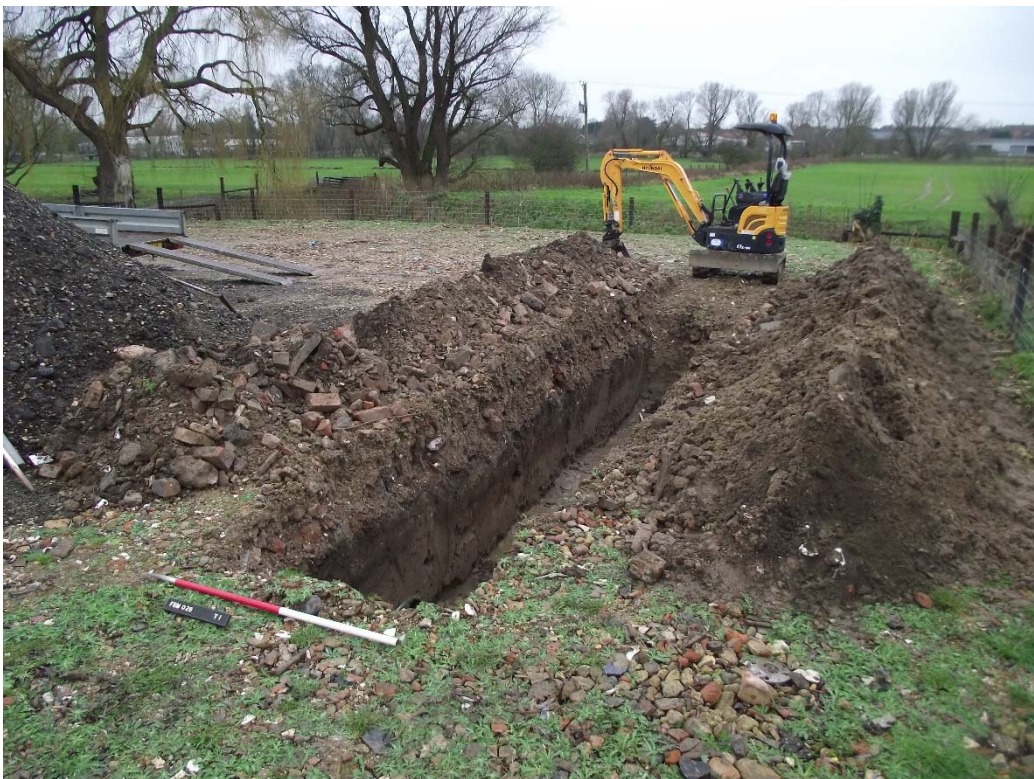
Plate 3. General view of trench looking south with the floodplain of River Lark behind.
