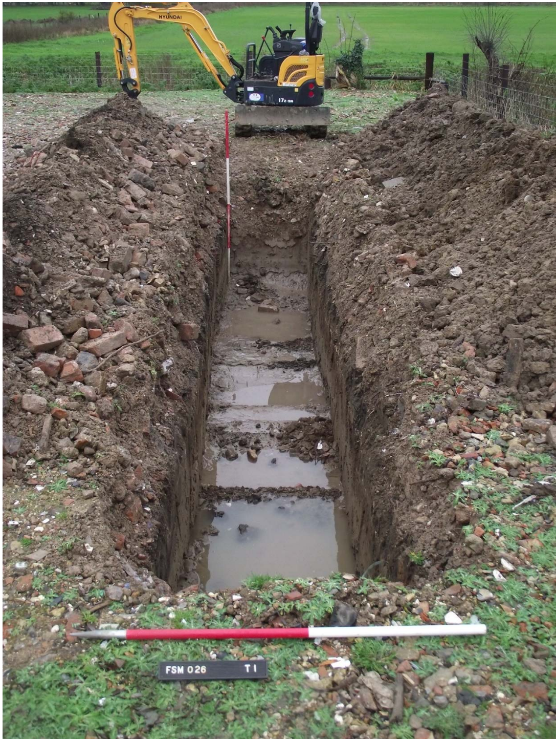
Plate 1. View of the trench looking south-west. The ranging rod in the foreground is 1m.
