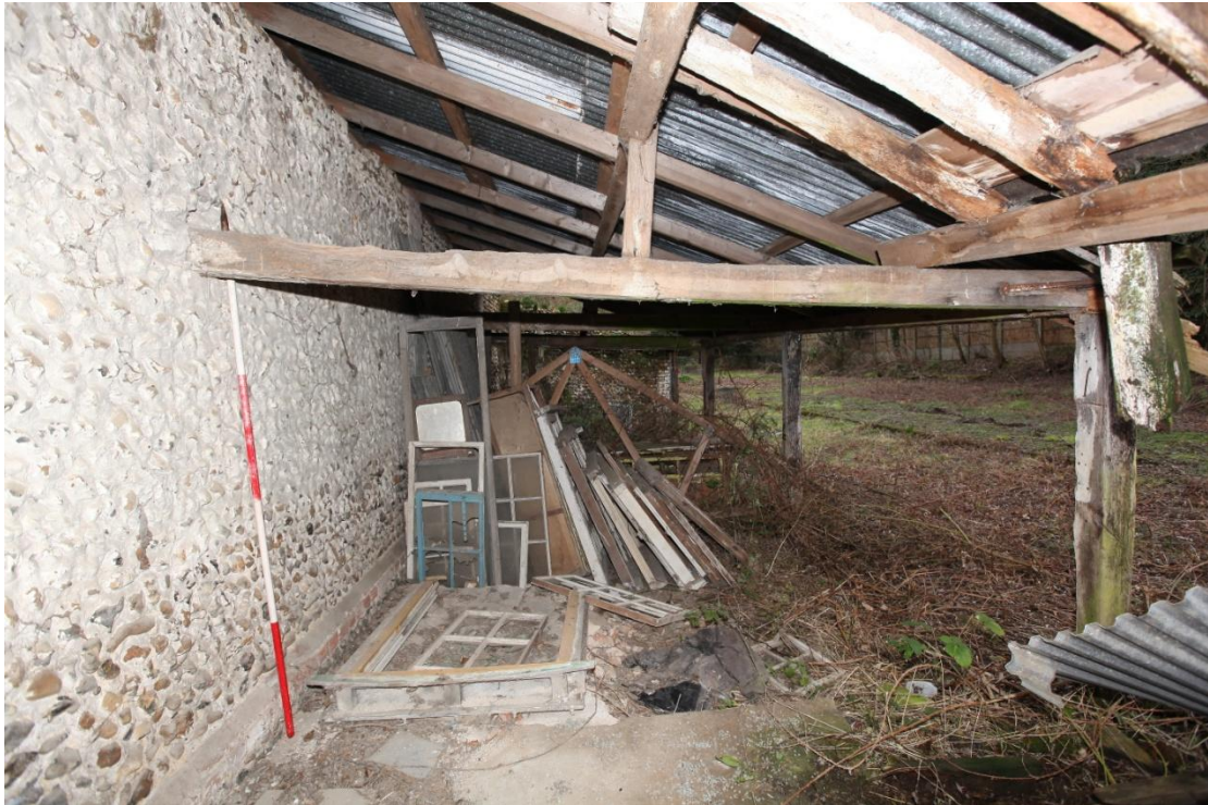
Illus. 13. The interior of the western open-sided shed (1a) seen from the west. An original tie-beam is embedded in the whitewashed flint-rubble wall to the left, with a small number of original rafters (top right). The majority of the present roof is a 20 th century replacement of machine-sawn softwood.
