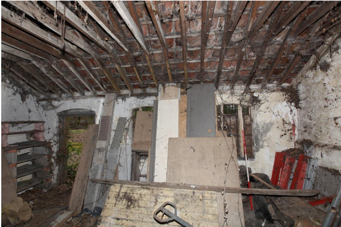
Illus. 5. The rendered and colourwashed interior of the pantiled shed’s western facade (3a) showing its original windows with iron glazing bars. The roof structure of machine-sawn softwood with nailed collars also appears to be original to the walls.
