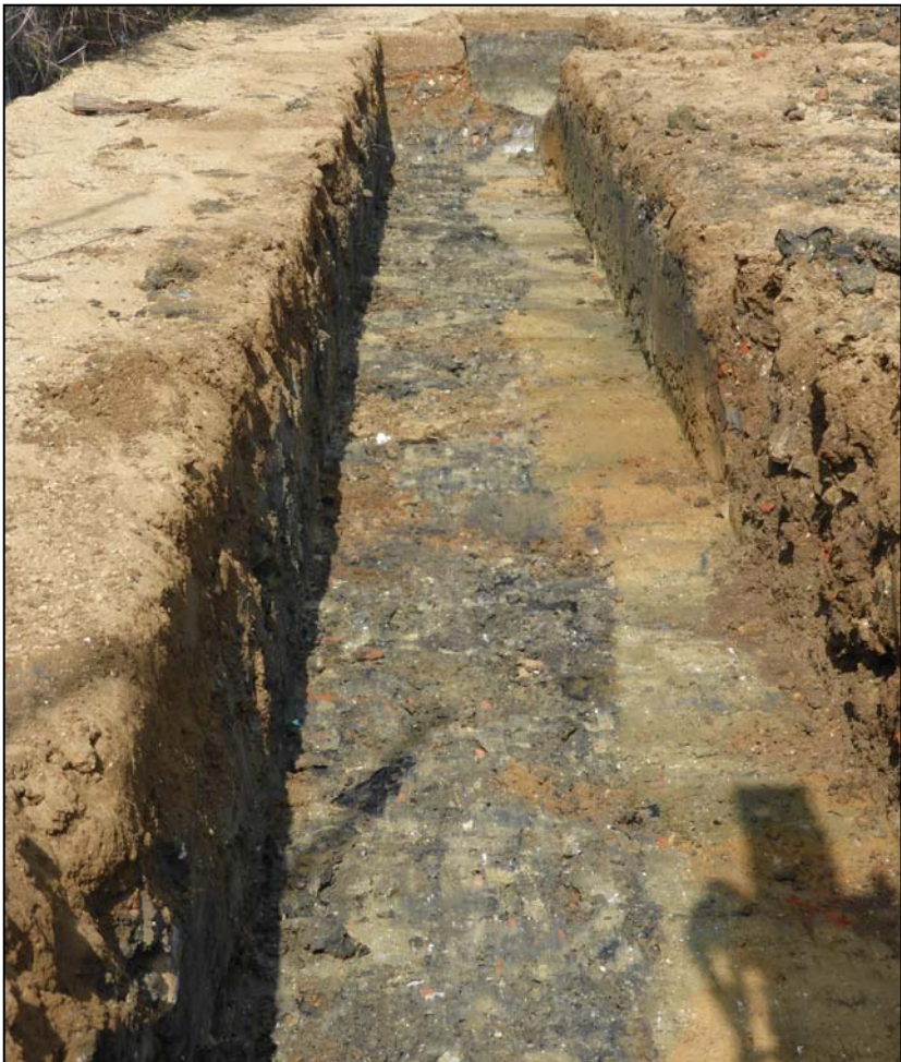
Plate 2. General view of Trench 1, showing service run along east edge (camera facing north)
