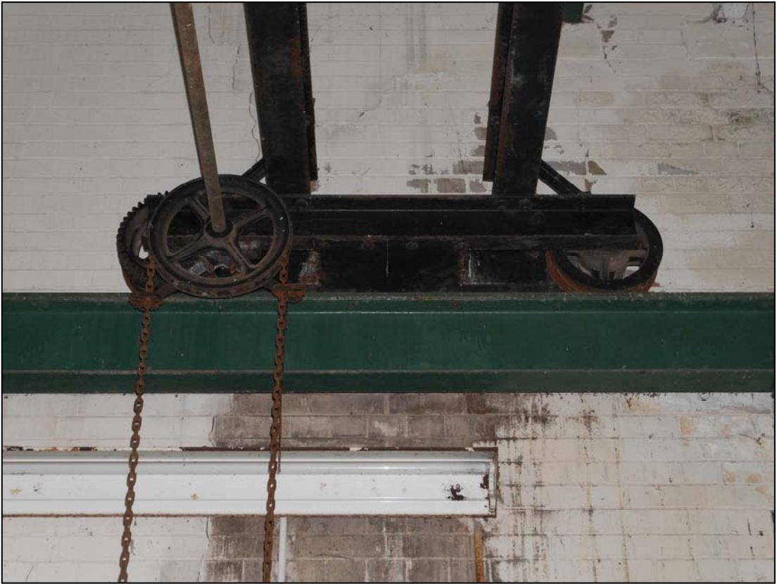
Plate 61. Crane truck, at the southwest end of the bridging girders. The chain operated drive mechanism can also be seen
