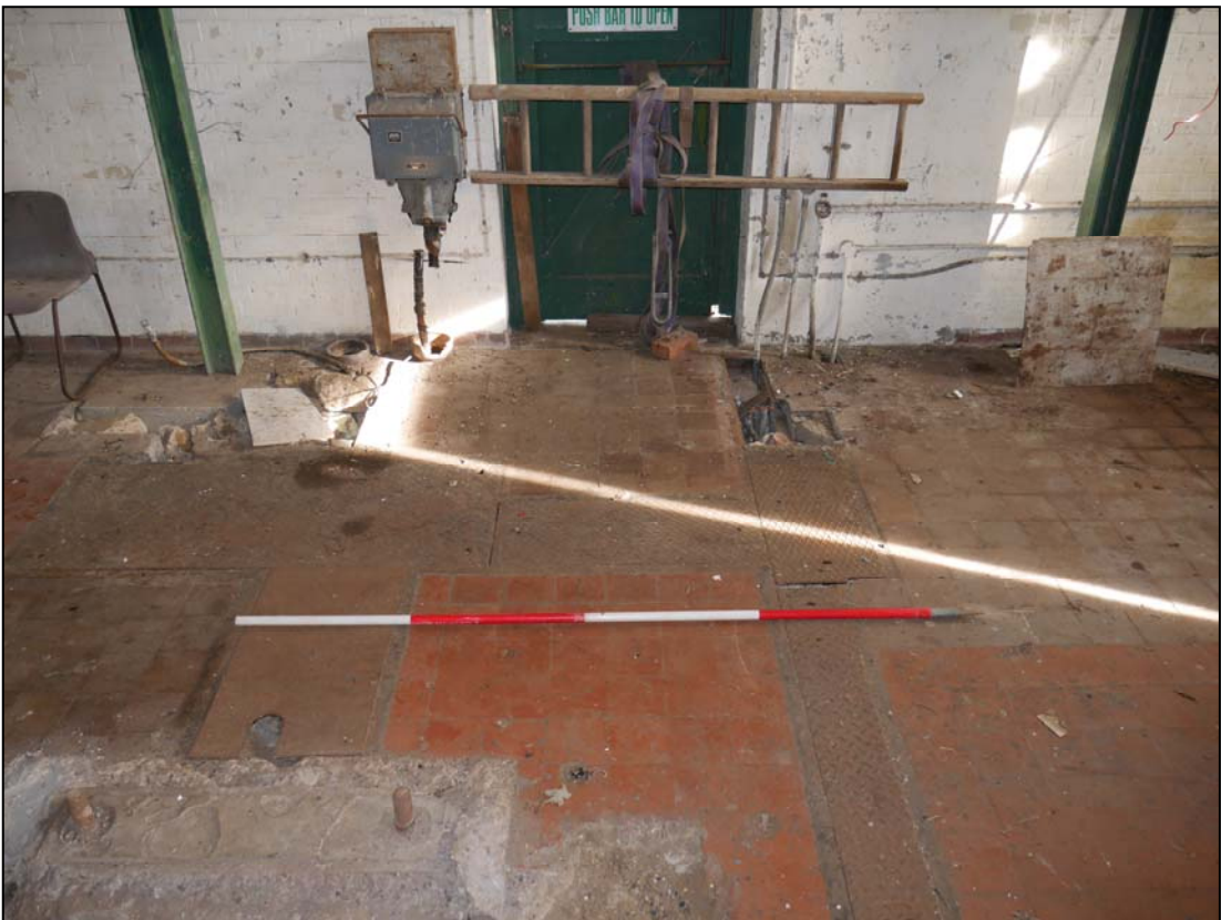
Plate 54. Covered service ducts in vicinity of northeast doorway. A disconnected electric isolator mounted on the wall is also visible
