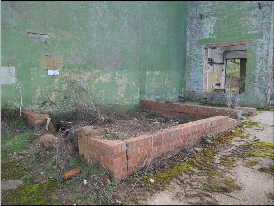
Plate 25. Transformer enclosure on southwest side of Generator House, camera facing east
