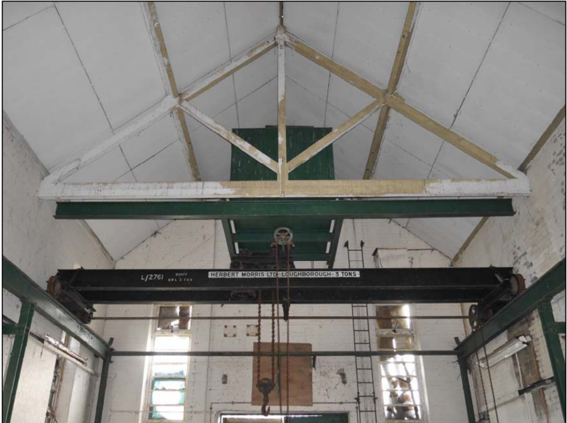
Plate 47. View of the king post timber roof truss and the gantry crane. Also visible is the large water tank and its supporting girders
