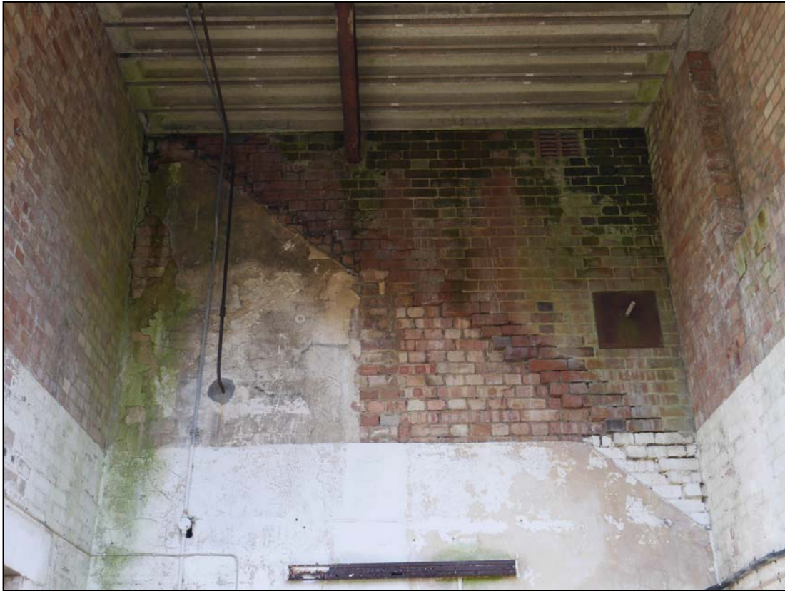
Plate 27. 'Scar' in brickwork of southwest wall, visible within the cooling tower
