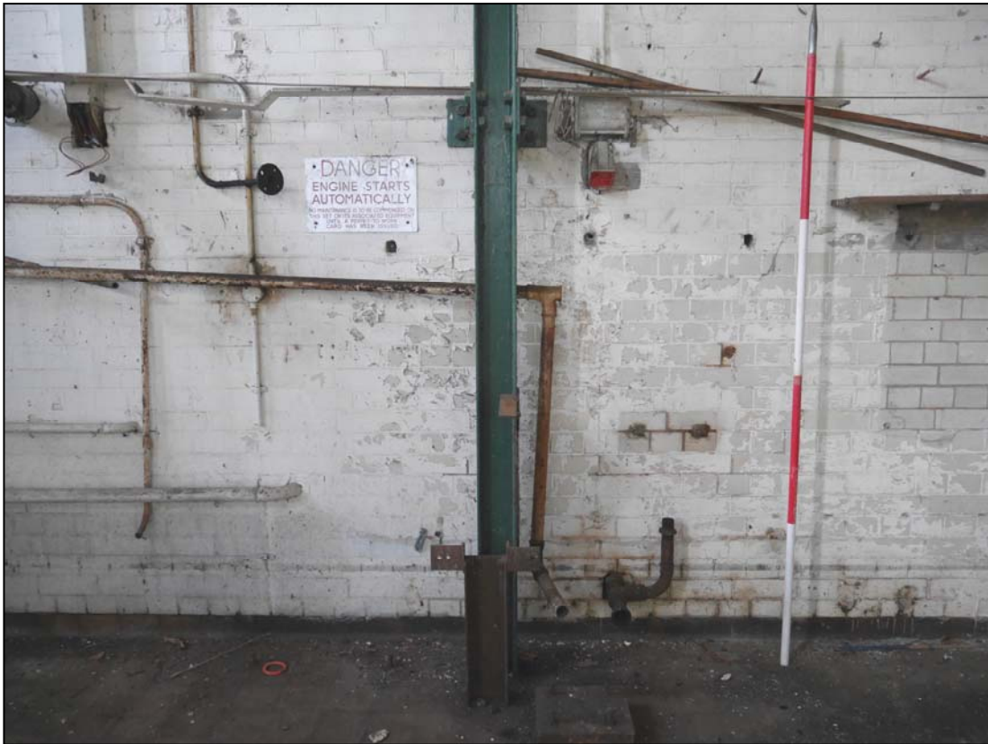
Plate 49. General view of the northwest wall within the main room showing the glazed and unglazed brickwork with remnants of later white paint
