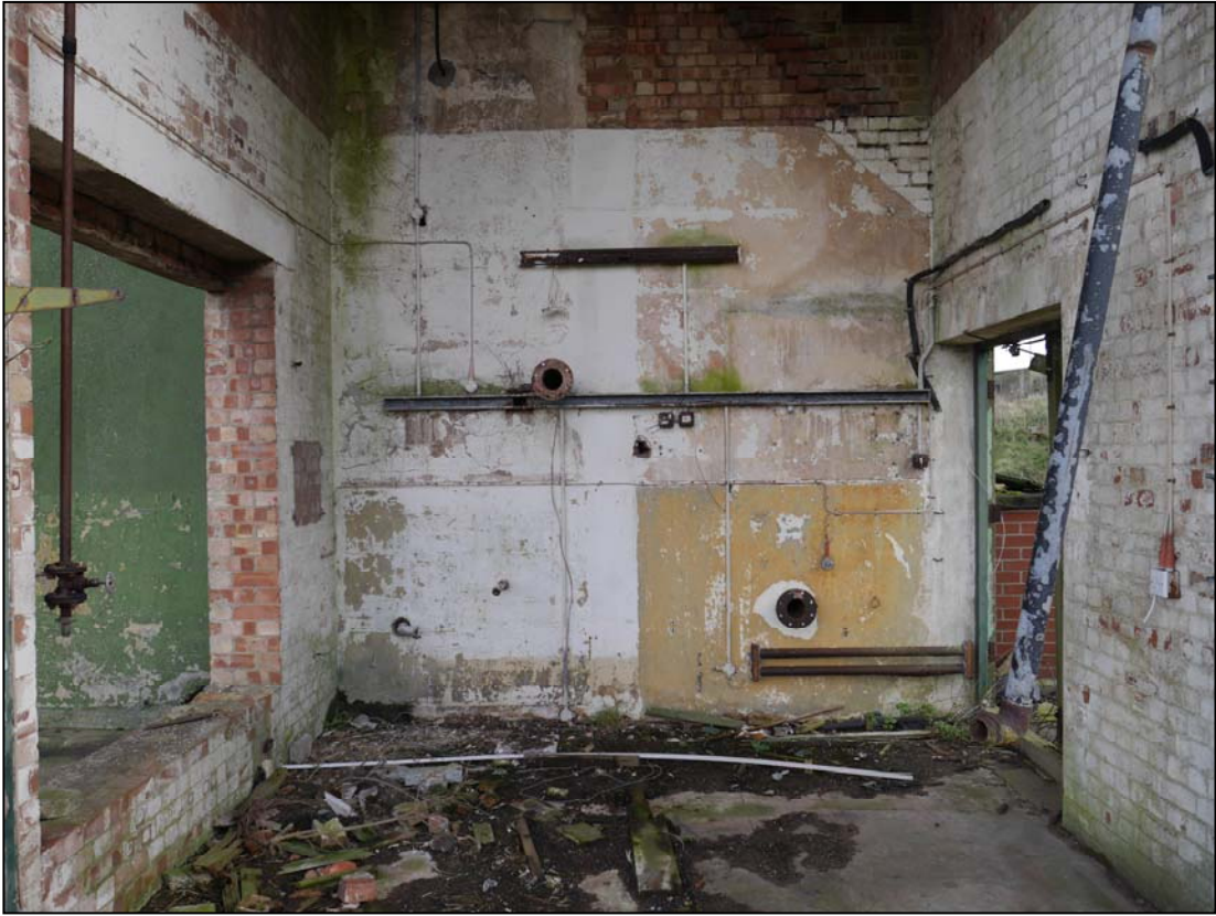
Plate 37. View into the cooling tower showing pipes etc. on the northeast wall
