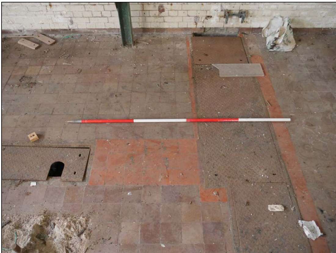
Plate 50. Floor surface within the main room showing the use of different colour tiles
