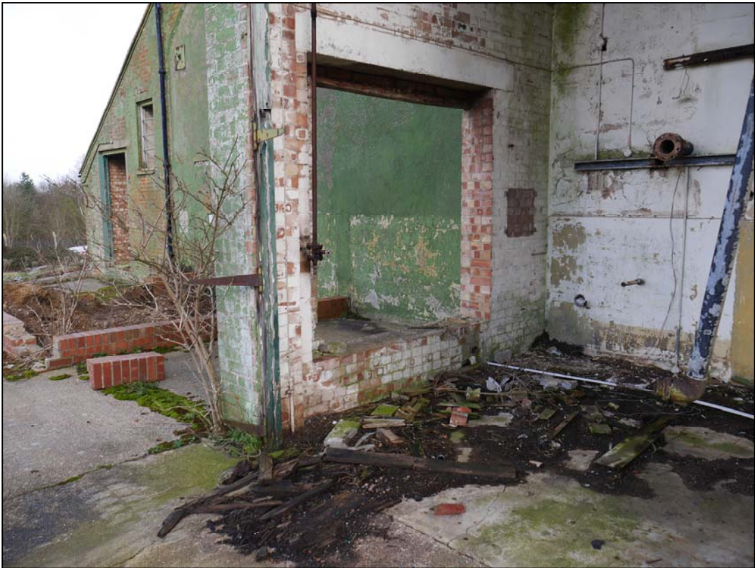
Plate 36. View through large opening in southwest wall of cooling tower showing hinges for a former door mounted on the northwest edge. Also visible is the opening in the northwest wall
