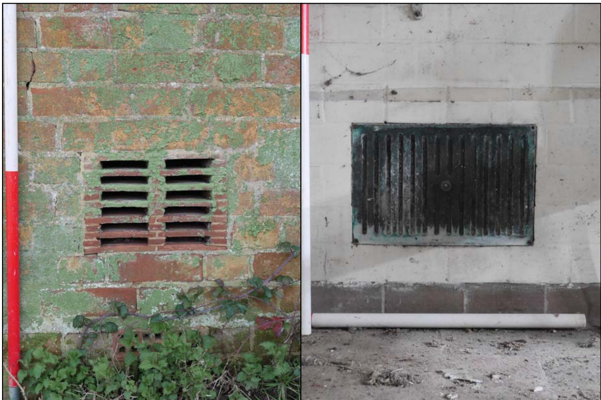
Plate 24. Generator House vents, external and internal views
