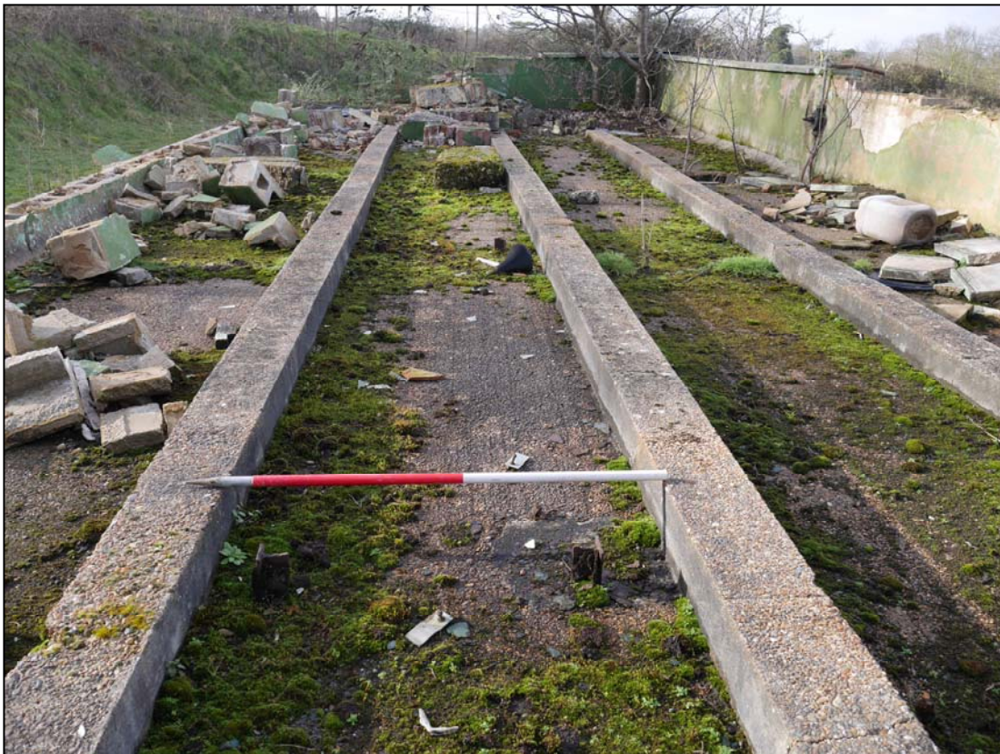
Plate 74. Concrete 'beams' and 'T'-section iron uprights within the fuel storage area camera facing southwest
