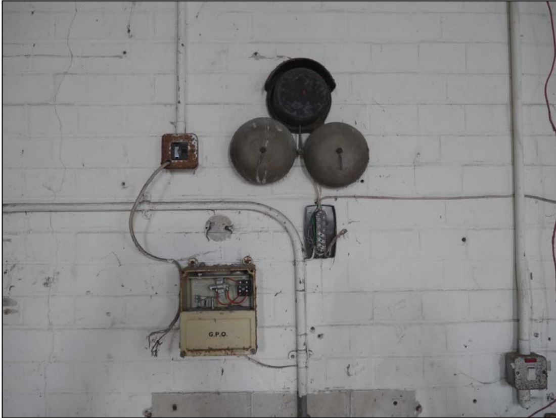
Plate 65. Telephone equipment on the northwest wall (a repeater set of bells were also located on the northeast wall)
