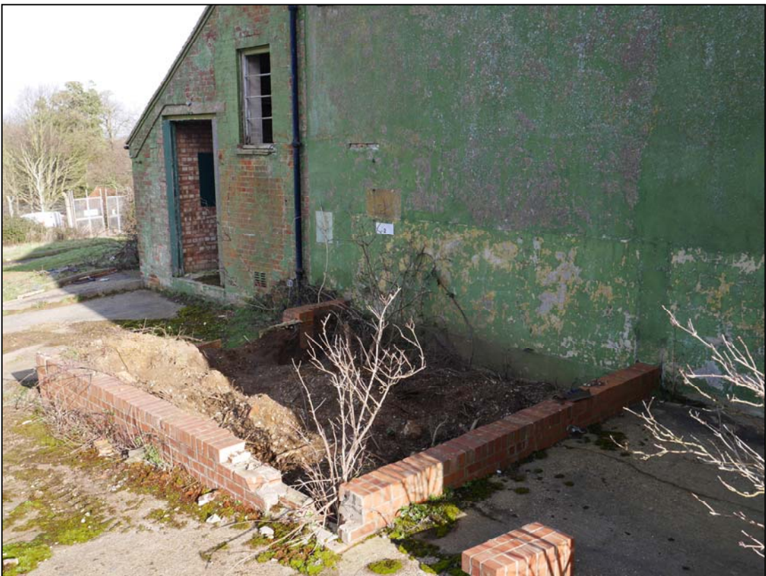
Plate 26. Transformer enclosure on southwest side of Generator House, camera facing north
