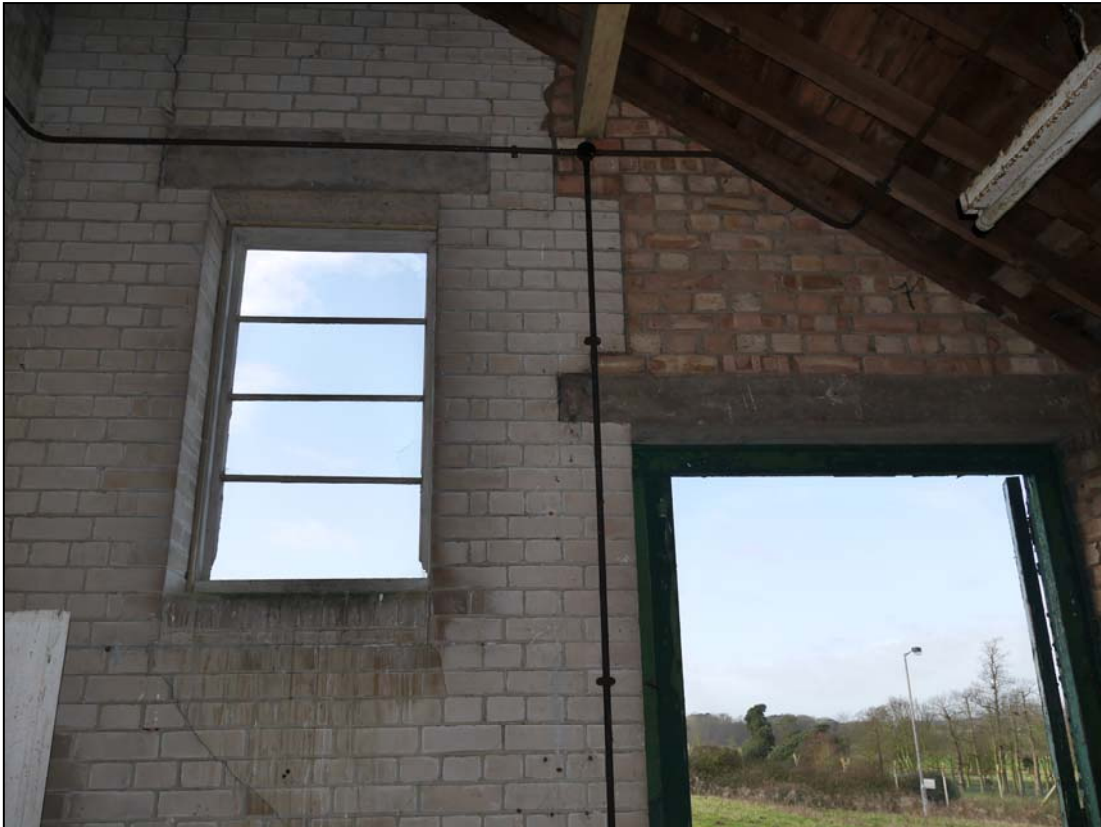
Plate 19. Fixed window in southwest wall of store, also shows the lintel and renewed brickwork associated with what is probably an inserted door
