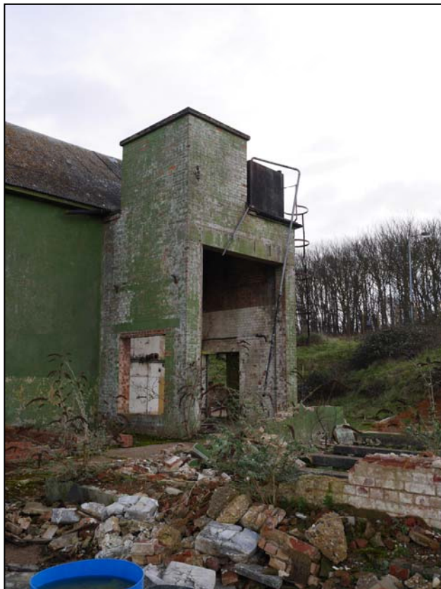
Plate 30. View of the cooling tower, camera facing east
