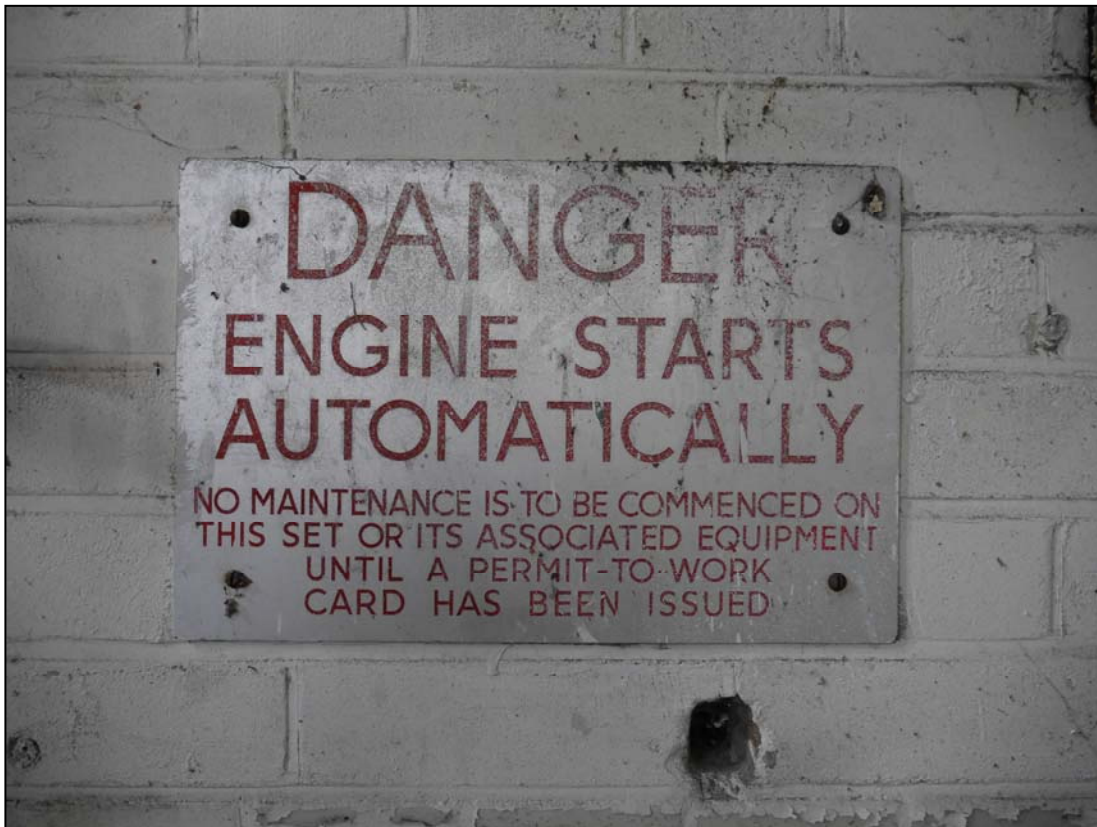
Plate 64. Warning sign, southwest wall
