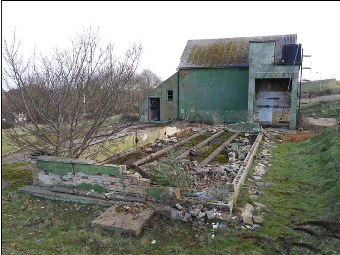
Plate 73. The fuel storage area, camera facing northeast. Note the change to blockwork.
