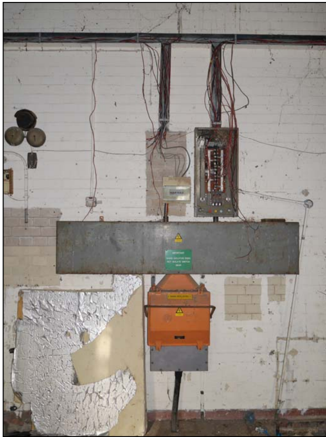
Plate 55. Electrical boxes and switchgear on the northwest wall of the main room
