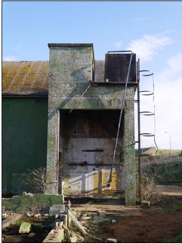
Plate 29. View of the cooling tower, camera facing northeast
