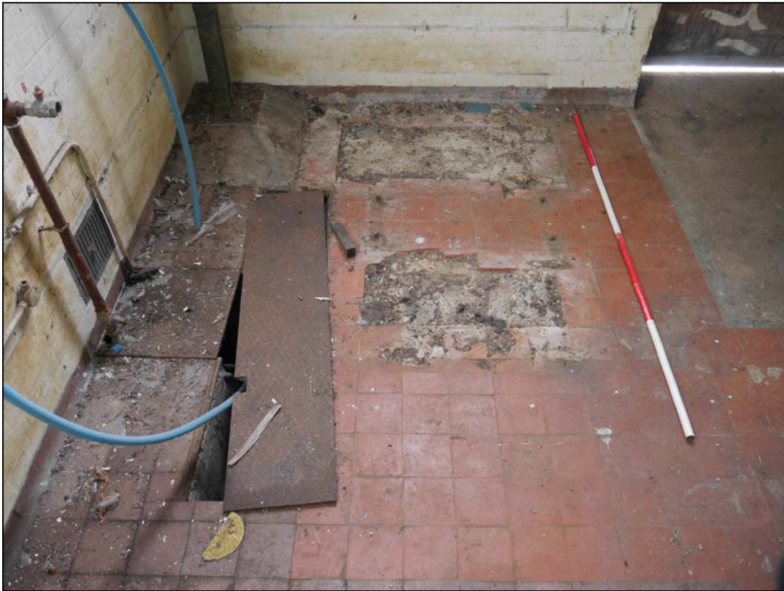
Plate 57. Site of Lister diesel compressor, eastern corner of main room
