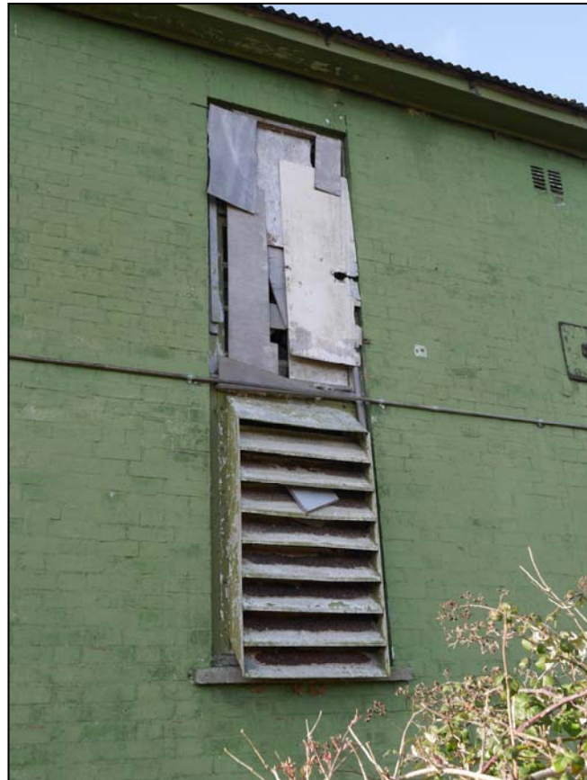
Plate 18. Mechanically operated louvered vent on main room window, external view
