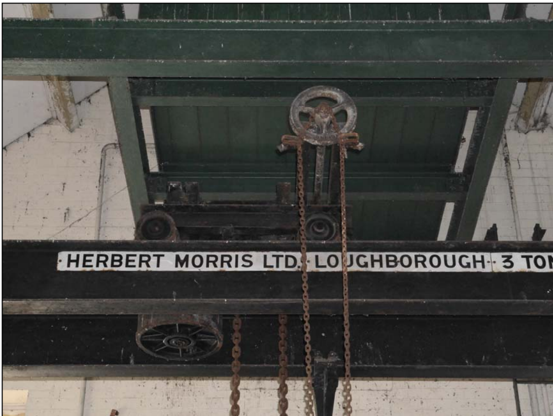
Plate 60. The gantry crane hoist trolley
