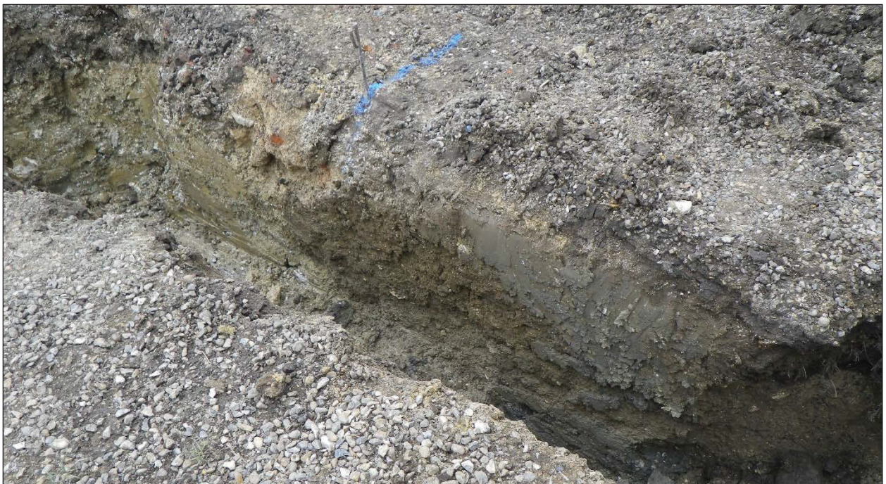
Plate 4. Southern edge of new foundation, showing possible pond underneath previous wall footing.
