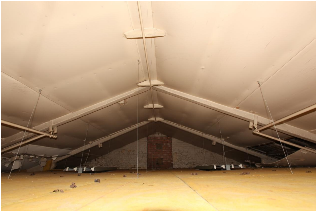
Illus. 8. The original ceiling of the southern classroom (1d) above the present suspended ceiling seen from the north, showing the blocked window in the southern gable. The chamfered principal rafters are of pre-cast concrete and the corrugated asbestos is hidden above nailed boarding.
