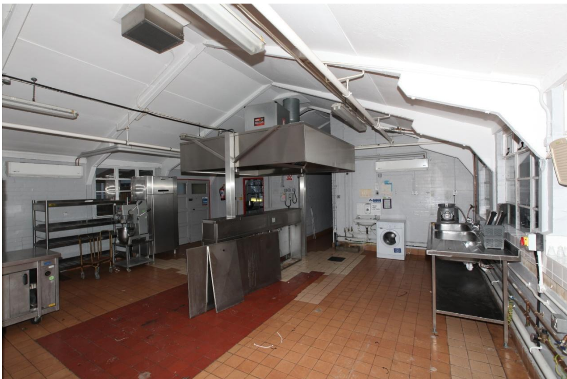
Illus. 10. The kitchen (2a) from the east, showing the original height of the ceiling with concrete principal rafters and bolted knee-braces. The axial passage (2f) is visible in the rear.
