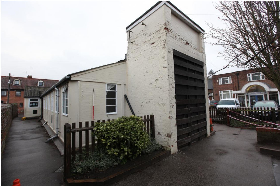
Illus. 5. The brick piers supporting a water tank adjoining the western gable (2e) with the main school building visible to the right. The wooden doors are recent insertions and the piers were formerly open to the yard.
