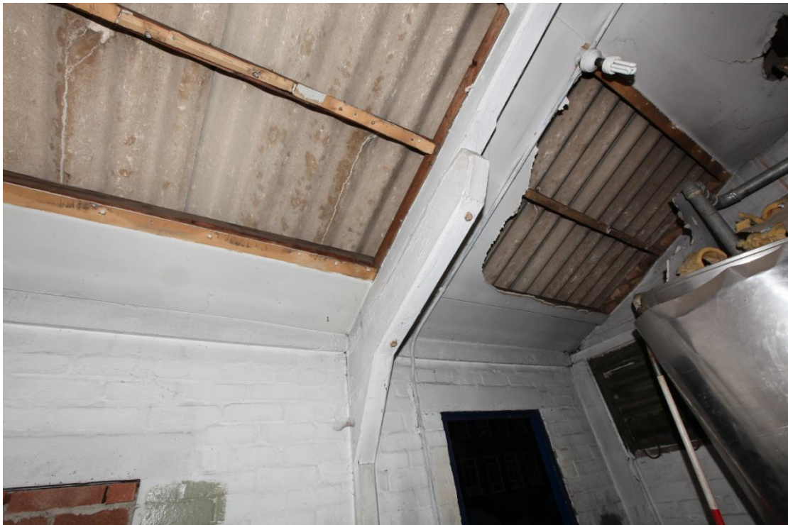
Illus. 16. The southern internal wall of the boiler room (2g) showing its external entrance door and exposed roof structure. The softwood battens supporting the corrugated asbestos are attached to concrete rafters which are linked to the wall piers by bolted knee-braces of pre-cast concrete.
