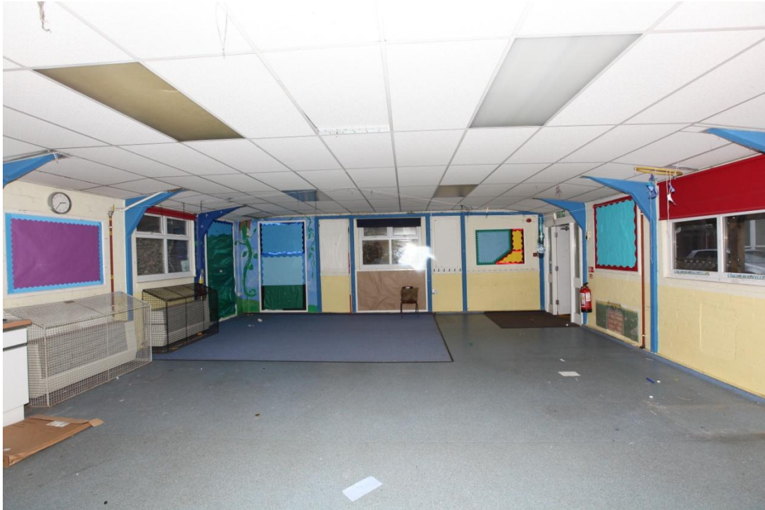
Illus. 7. The southern classroom (1d) from the north showing the original bolted pre-cast concrete knee-braces beneath the later ceiling.
