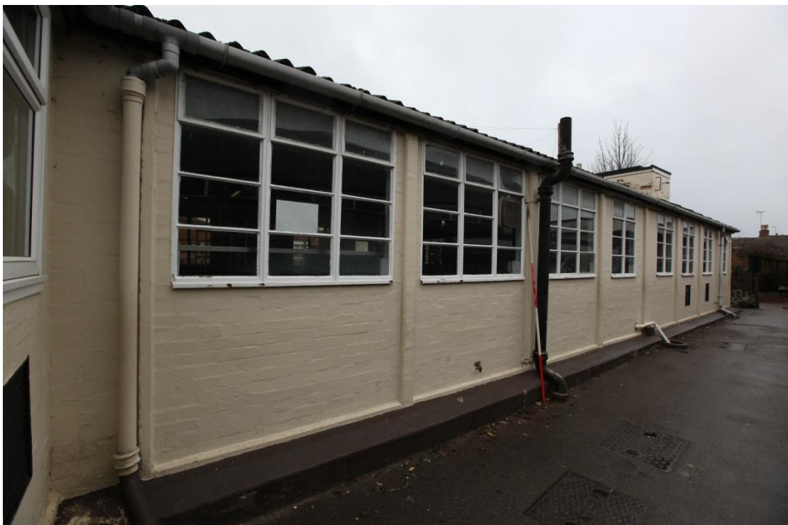
Illus. 4. The northern exterior of the western range (2) showing its largely unaltered appearance with a full complement of original Crittall windows. Its junction with the eastern range is visible on the left.
