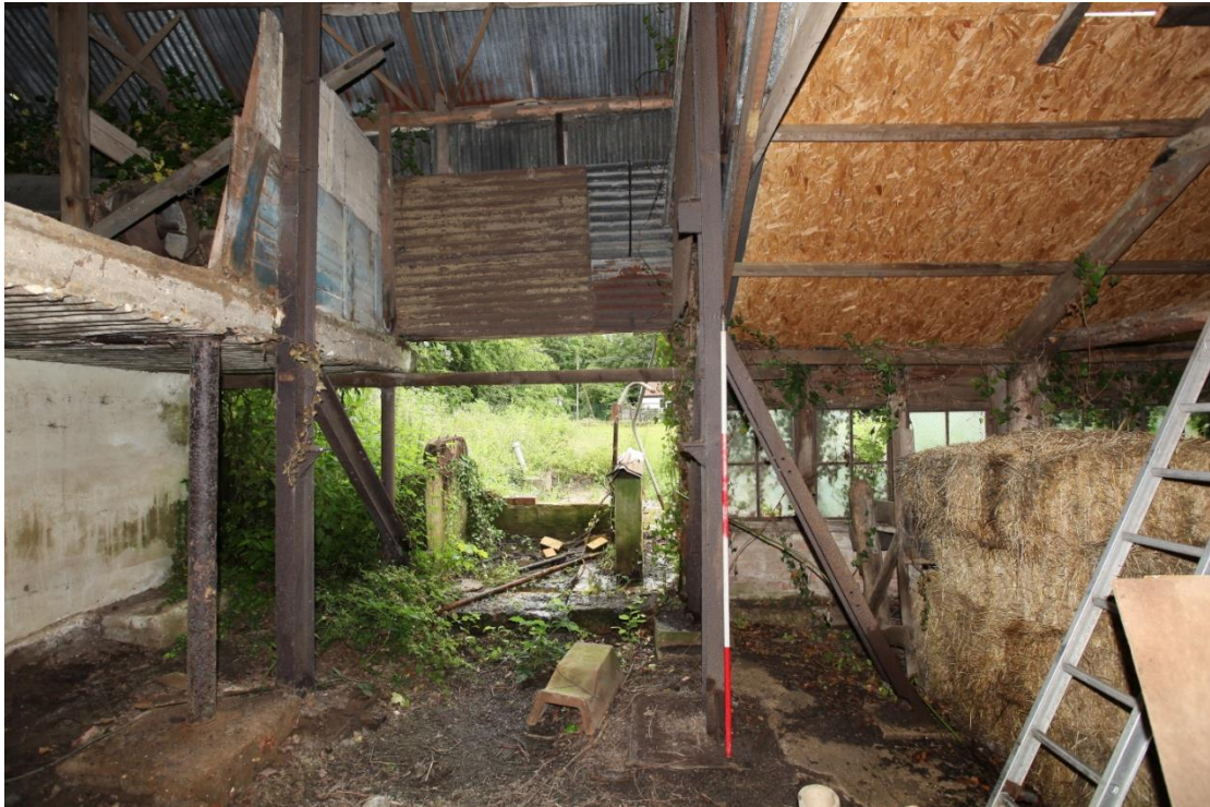
Illus. 15. The lower level of the extrusion shed (3a) from the south showing the position of the missing machinery in the centre with the concrete platform of the loading and clay fining area on the left and the ‘making shed’ (3b) on the right. A demolished additional structure extended northwards from this part of the structure.
