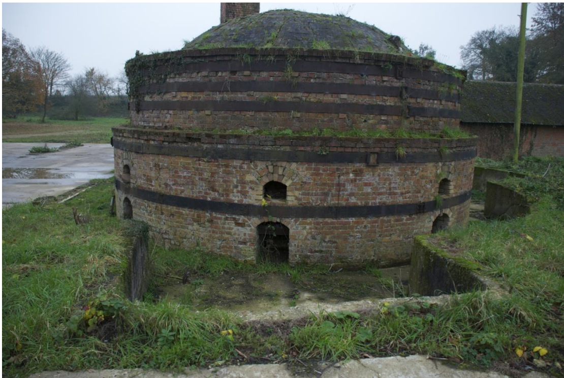
Illus. 18. A 2014 photograph of the kiln (1) from the north without a tarpaulin showing its domed roof and multiple iron straps.
