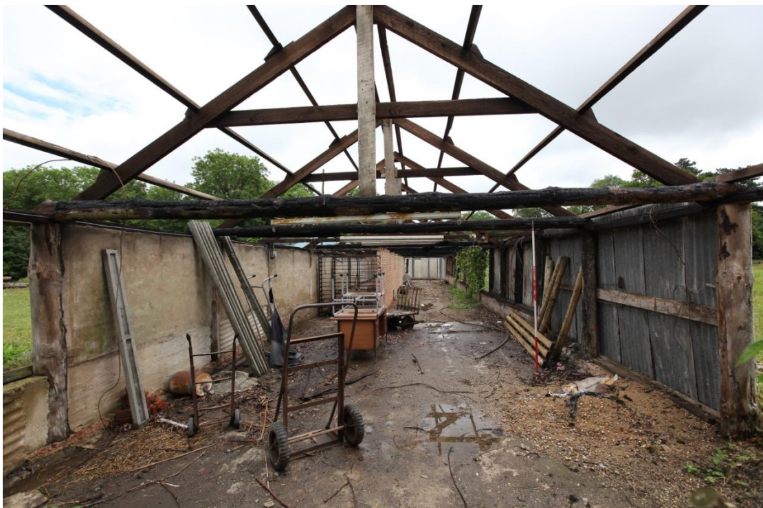
Illus. 12. The drying shed (4) from its western gable showing its charred tie-beams and wall posts with a later softwood roof above. This area contains a wooden hand trolley and two sack barrows along with an office desk.
