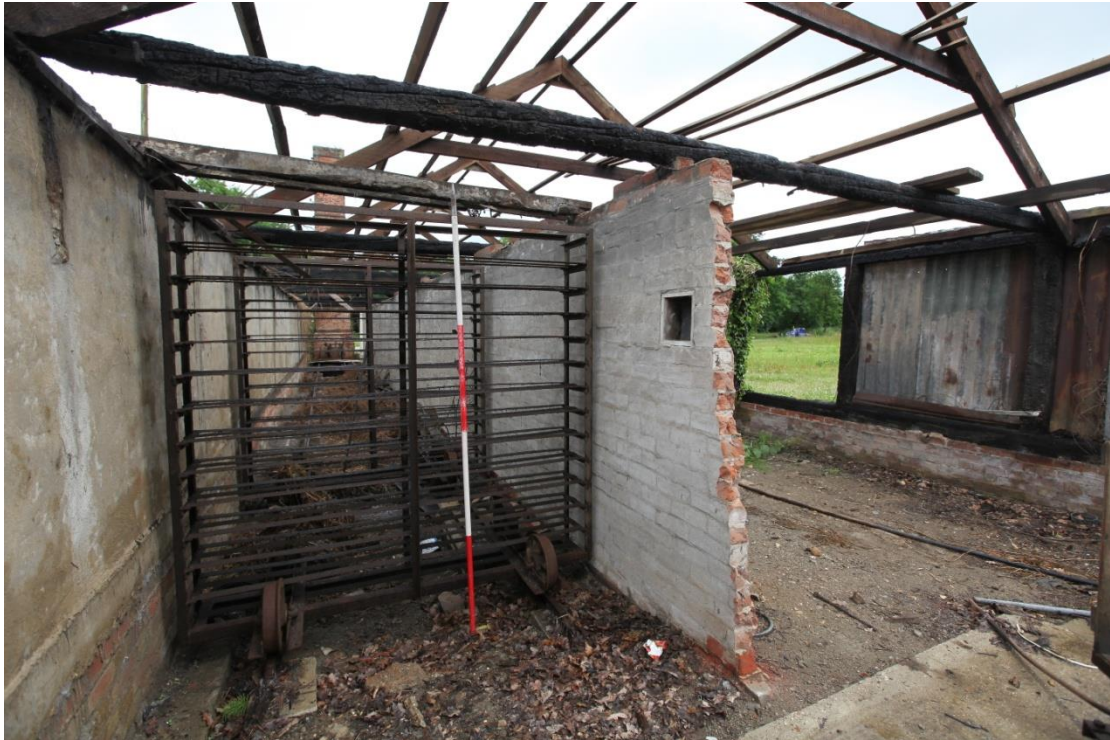
Illus. 11. The hot air drying tunnel (4a) from the west showing two drying racks on bogey wheels. The brick partition adjoining the central range (4b) on the right has been truncated by a later concrete floor and is a secondary insertion to the original shed.
