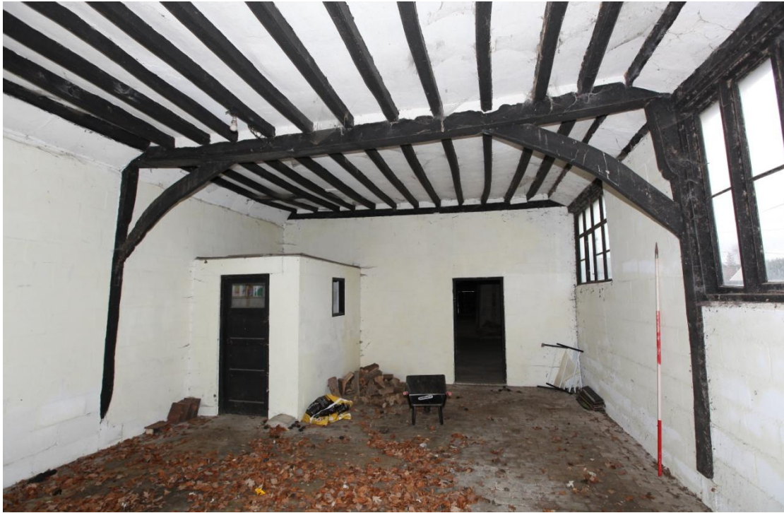
Illus. 13. The interior of the northern section of the former stable (2b), seen from the north, with the block-work partition to the southern section (2a) in the rear. The arch-braced tie-beam is original, but both storey posts contain pegged mortises for the binding joist of a missing original ceiling just below the braces – so the present ceiling is a later insertion that may relate to the building’s alleged conversion into a schoolroom. This compartment originally extended to the central tie of the southern section (2a).
