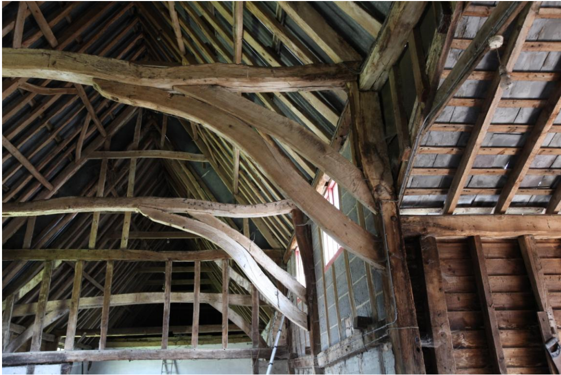
Illus. 7. A detail from the south of the two unusual serpentine bolted braces reinforcing the original arch-braces in the northern bays of the barn (1a). All but two of the original eight arch-braces survive intact. The right-hand post contains an empty double-pegged mortise for an original porch on the site of the present 19 th century porch (1b).
