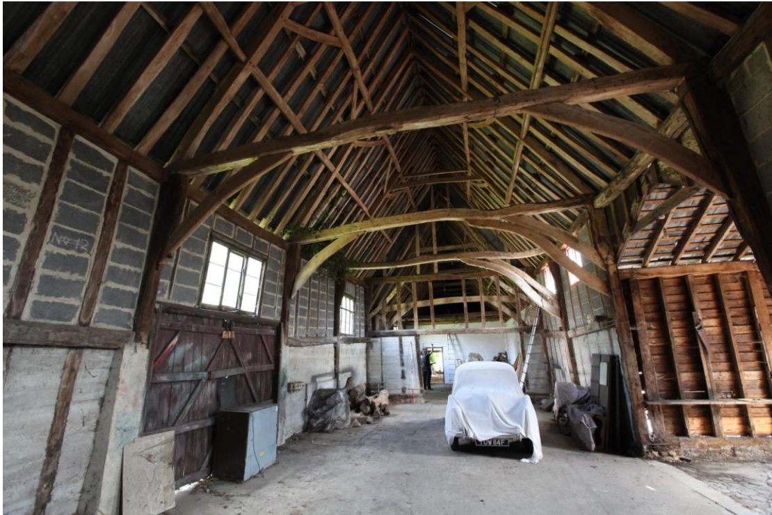
Illus. 5. The interior of the five-bay threshing barn (1a) from the south showing its largely complete timber-frame with mid-rails and externally trenched corner braces. The upper studs are infilled with cement blocks and the lower with shuttered concrete bearing the incised date 1947.
