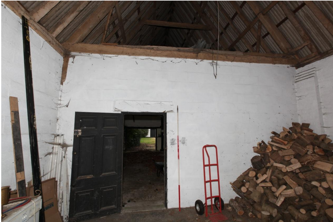
Illus. 11. The 20 th century cement-block northern wall of the former stable's southern section (2a), with a connecting door to the two northern bays (2b). The arch-braces of the original open truss survive within the block-work as their profiles are clearly visible to left and right. The framing of the external walls has been replaced with block-work to the west (left) and 20 th century brickwork to the right.
