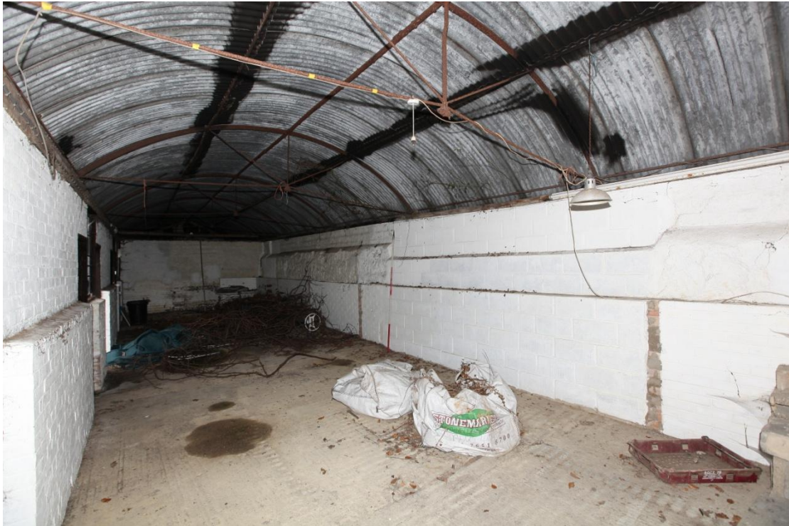
Illus. 17. The interior from the south of the former shelter-shed (3a) showing its early-20th century steel-framed segmental roof of corrugated iron. Part of the eastern wall on the right consists of shuttered or rammed clay, but has been raised in height with clay-lump (i.e. pre-fabricated blocks of clay). The internal partition in the rear also consists of clay-lump.
