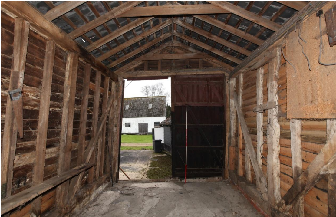
Illus. 9. The interior from the main barn to the west of the eastern porch (1b), showing fragments of mid-19 th century framing in the right-hand wall with nailed primary braces interrupting the studs. The roof and much of the left-hand wall have been rebuilt in softwood, probably when the doors were replaced early in the 20 th century - as dated by an incised inscription to the latter's right-hand jamb: EP AGE 16 JAN 11 1913.
