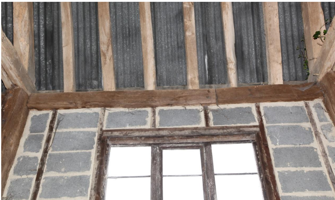
Illus. 8. The western roof-plate of the barn's central bay (1a) showing later, narrow studs infilled with 20 th century cement block-work and a modern glazed window. The face-half and bladed scarf joint above the right-hand window mullion was first introduced in circa 1600 and indicates an early-17 th century date for the structure. The circular holes for the 'pin' hinges of the original barn doors are visible in the underside of the roof-plate to the left and right. The central threshing floor therefore appears to have been entered from Church Green rather than the base court on the east.
