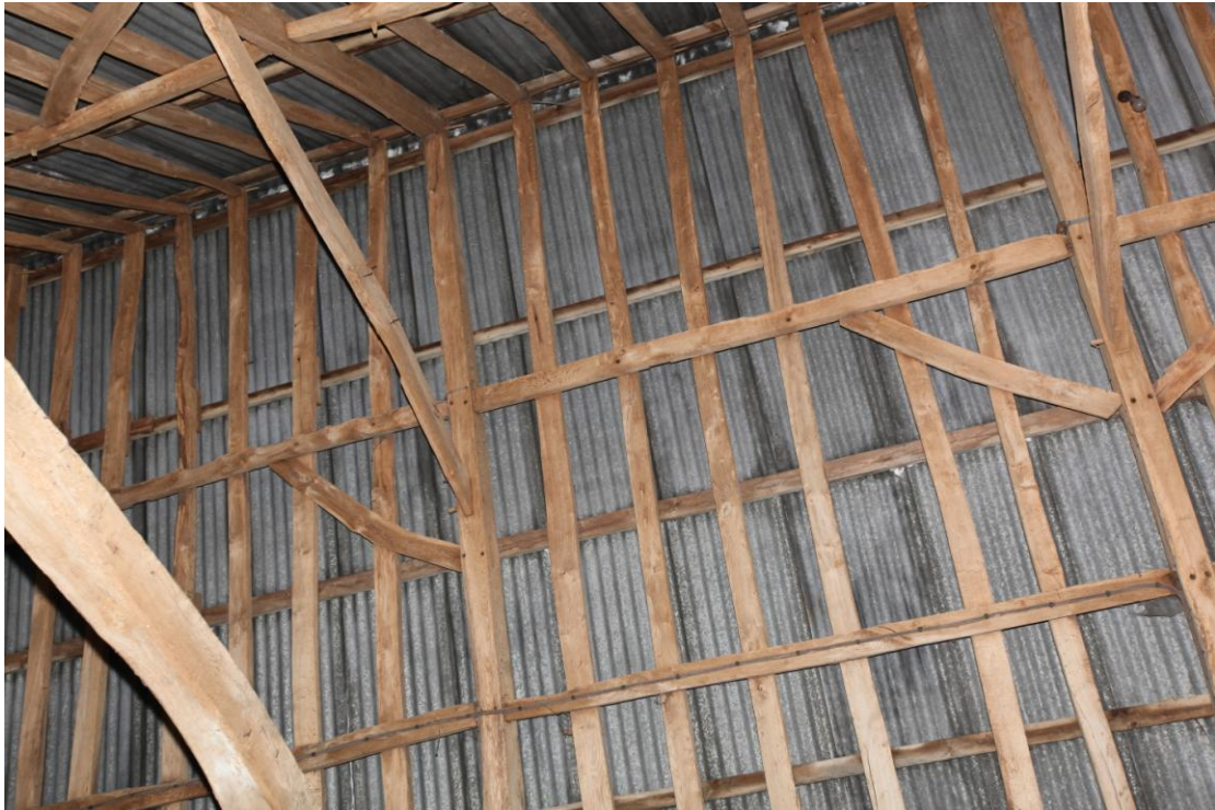
Illus. 19. A detail from the west of the intact two-tier butt-purlin roof structure of the barn (1a) showing a pegged mortise for a missing wind-brace in the principal rafter to the left.
