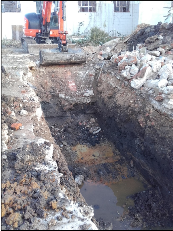
Plate 5. Trench 3, looking east. Brick footings visible in the section below the machine bucket
