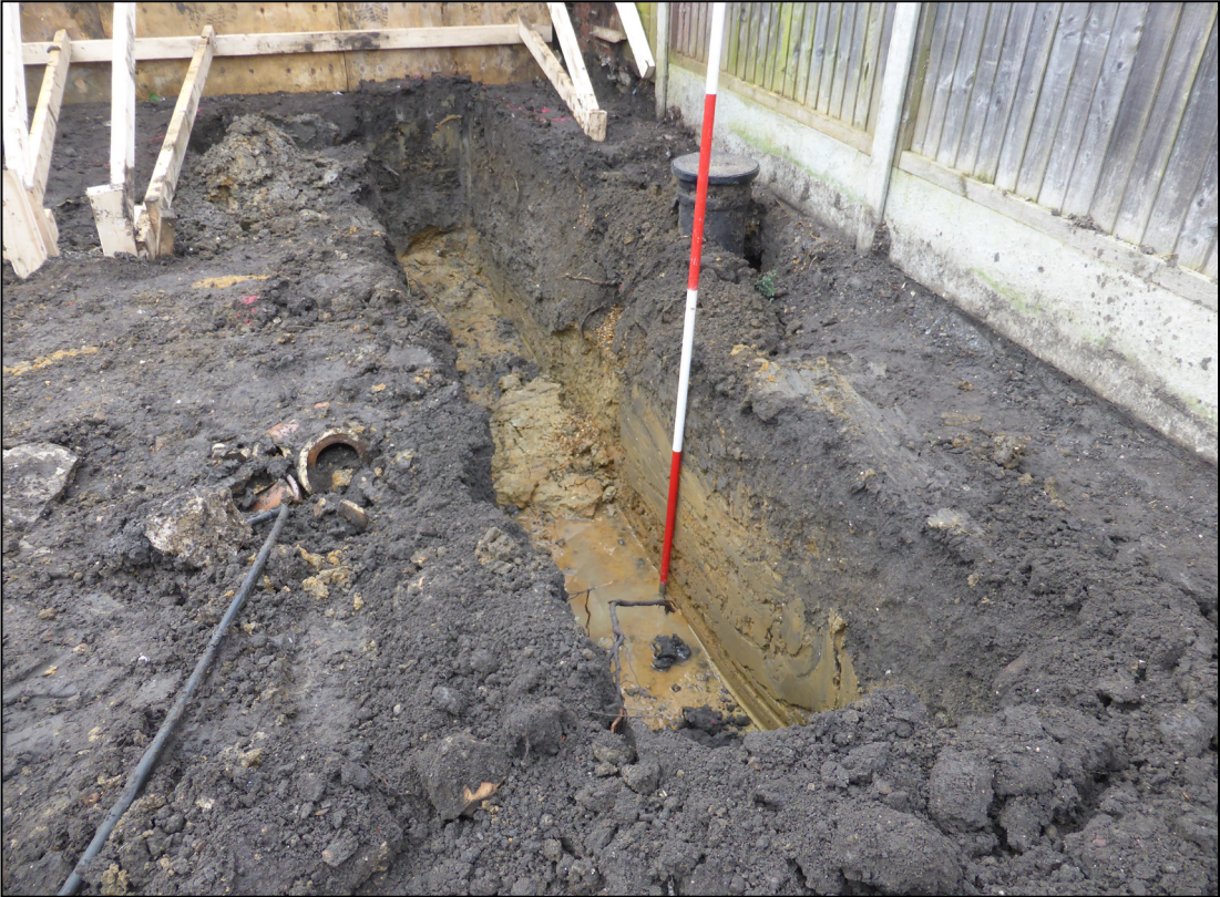
Plate 2. General view of footing trench showing typical soil profile, camera facing southwest
