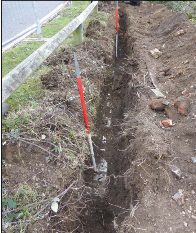
Plate 29. Item 11, length of brick wall running along base of trench (camera facing NE)
