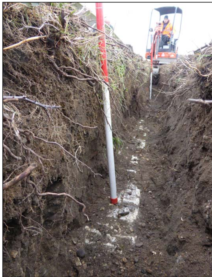
Plate 30. Item 11, length of brick wall running along base of trench (camera facing NE)
