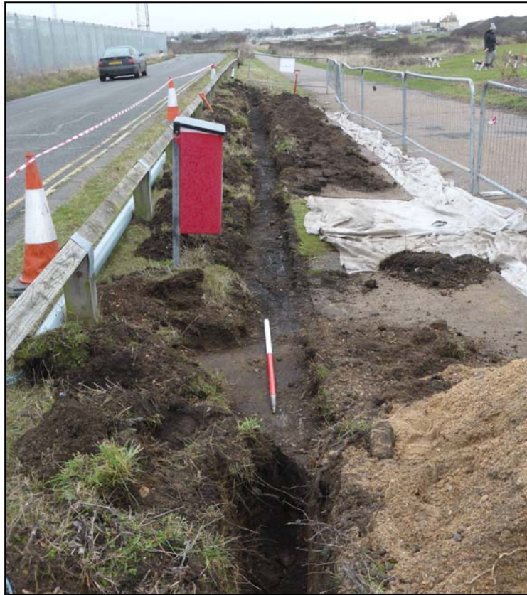
Plate 35. Item 13, concrete slab forming a lay-by adjacent earlier fort road (camera facing NE)
