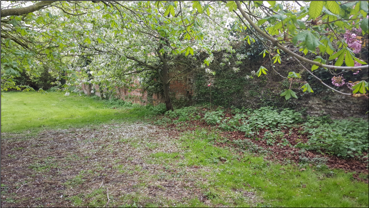
Plate 6. Interior of the curtilage wall, facing south-west, at point where medieval flintwork terminates
