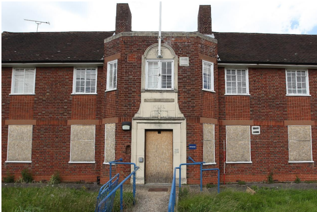
Illus. 2. The symmetrical southern facade showing the stone detailing of the entrance porch with a crown behind the flagpole and the incised word 'POLICE' above the door. A blue lamp bearing the same word is shown in earlier photographs but has been removed. Note the original Crittall windows and the tiled panels between the ground and first-floor windows.
