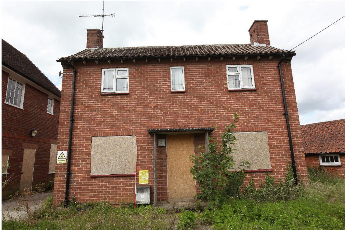
Illus. 5. The southern facade of the 1960s Police House showing its later PVC windows with the main station to the left and the 19 th century brick sheds to the right. The house operated most recently as additional office accommodation.
