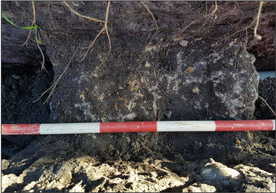
Plate 15. Item F: probable concrete footing, northern of a group of three, showing linear slot
