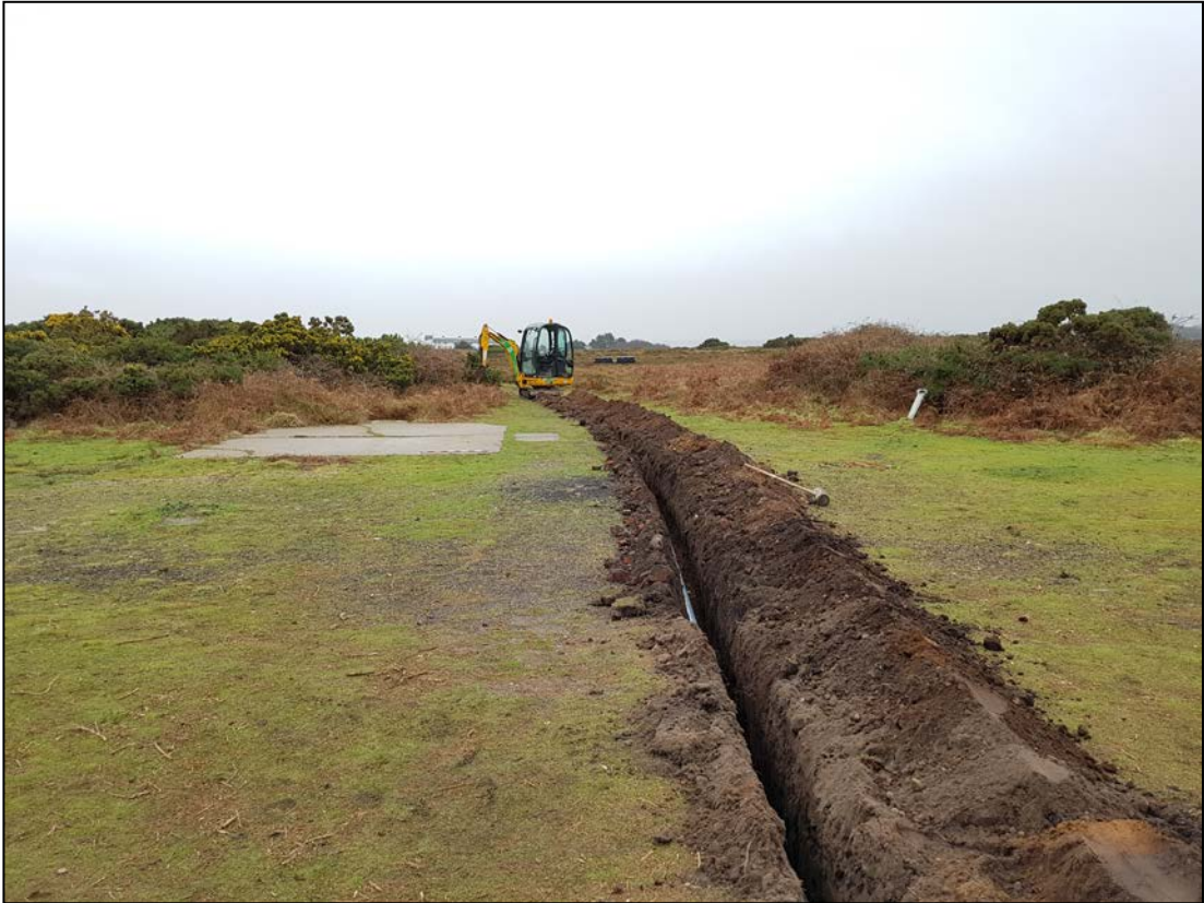
Plate 9. Base of guard room with trench running to the west (camera facing NE)
