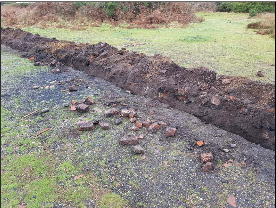
Plate 10. Brick rubble evident in area to the north of the guard room (camera facing SW)
