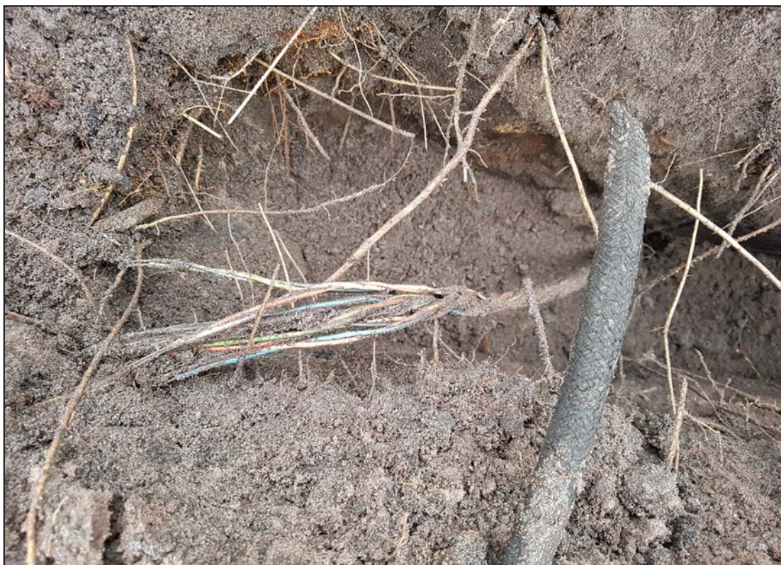
Plate 2. Item A: probable communications cable, the insulation, which was removed during excavation, is to the right (camera facing N)
