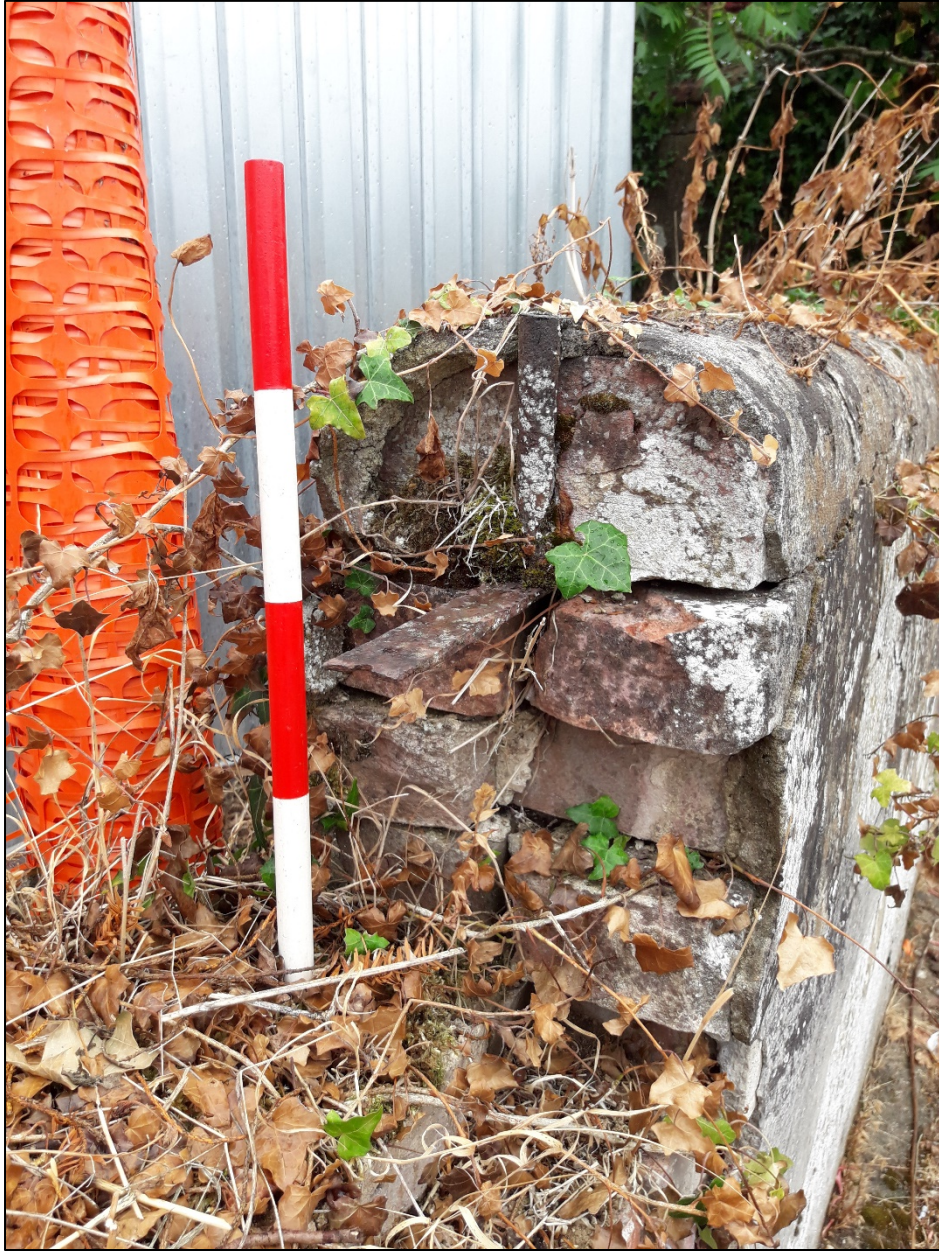
Plate 20. Section through the front wall, showing remnants of former iron railings. Looking NE, 0.4m scale
