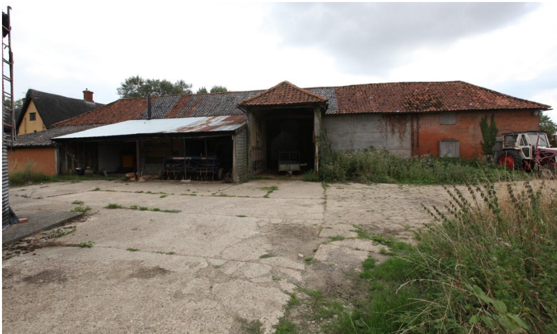
Illus. 2. The farm buildings from the north-east showing the long pantiled and hipped range of the mid-19 th century which encompasses contemporary brick extensions at both ends (2 and 3) and a four-bay barn of circa 1600 in the centre (1). The hipped porch (1e) projects from the back of the latter's threshing floor and is an exceptional and apparently in situ structure of just 3.8 m (12.5 ft) in width that initially contained a loft and was lit by three windows with pegged mullions.
