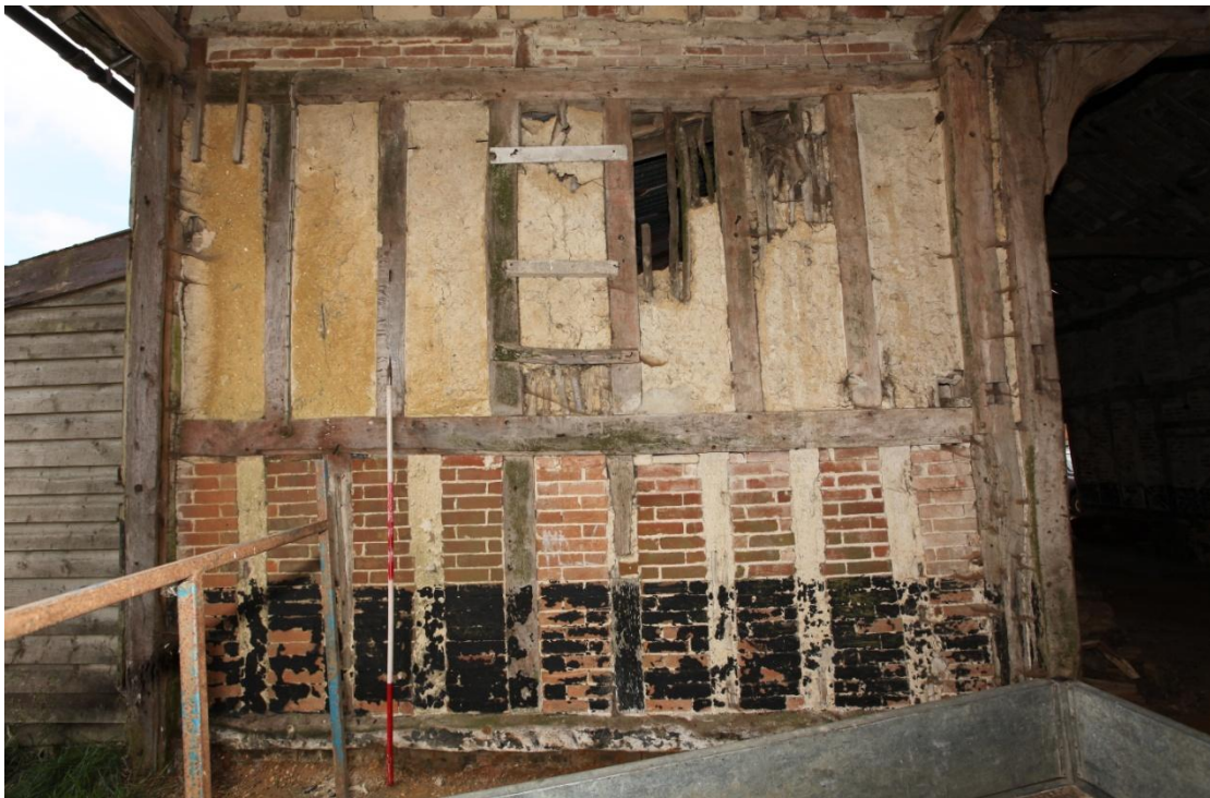
Illus. 10. The south-eastern interior of the porch (1e) showing evidence of a window with a shutter rebate and three pegged mullions on the left and a blocked original door to the right. The right-hand ground-floor stud is an unpegged insertion and the door rebate extends from the mid-rail to the corner post. The structure contained a ceiling of joists lodged on the mid-rails with corresponding pegged mortises in the truss adjoining the barn, but appears to have been open-framed against the barn both above and beneath the loft.
