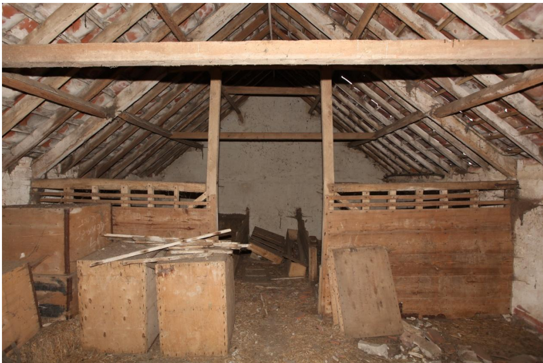
Illus. 14. The granary above the coach house (2) showing the remains of ostensibly original grain bins with an axial passage (as seen from the south-east).
