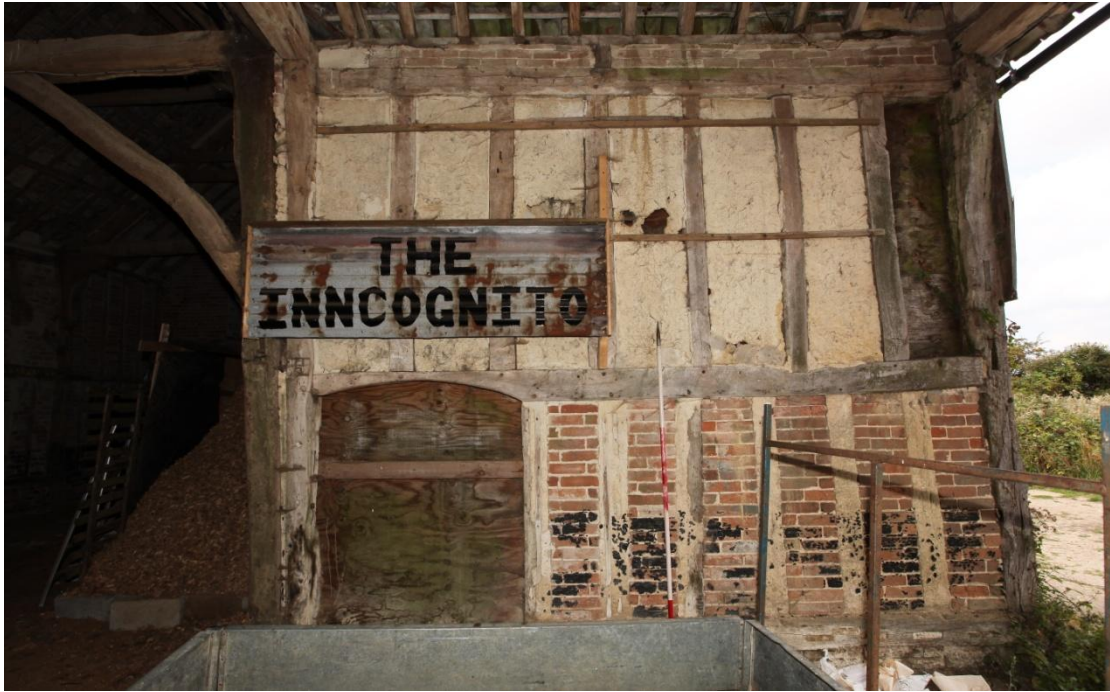
Illus. 9. The north-western interior of the porch (1e) showing its largely intact timber frame with a re-used ground sill. The wide door opened into a demolished lean-to shed, cutting the mid-rail and leaving no obvious evidence of an original door. The upper studs are infilled with original wattle-and-daub with 19 th century brick beneath.
