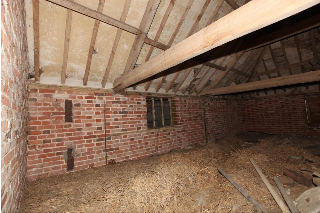
Illus. 15. The south-western internal wall of the hay loft to the north-west of the barn (3) showing an original window with a second window or loading hatch in the gable to the right. This loft is reached by the hatch shown in illus. A2. 7 and replicates the original arrangement of the barn's south-eastern bay (1a).
