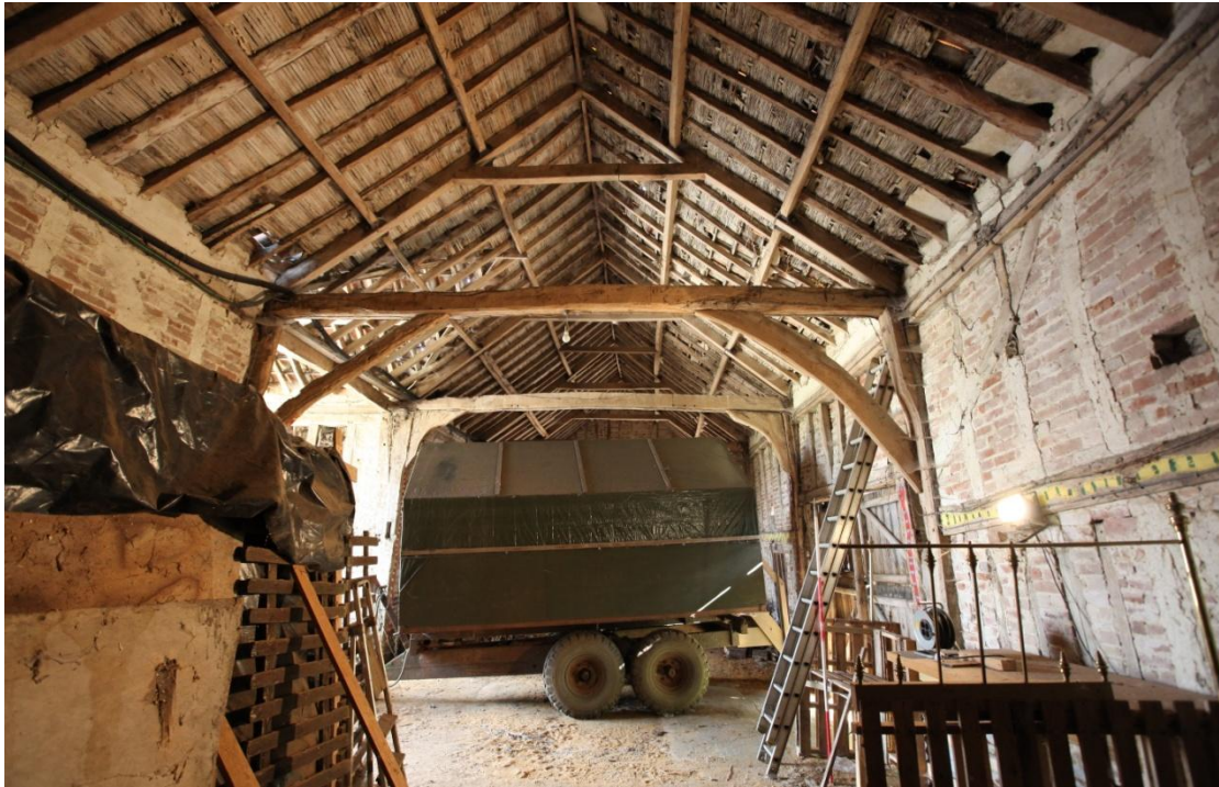
Illus. 5. A general view of the barn (1) from its missing north-western gable showing the intact original arch-braces to the tie-beam between the entrance bay (1c) and the end-bay in the foreground (1d). The butt-purlin roof is a mid-19 th century replacement which extends into the brick additions (2 and 3) that are not shown on the 1838 map. The brick infill between the timbers dates from the same period.
