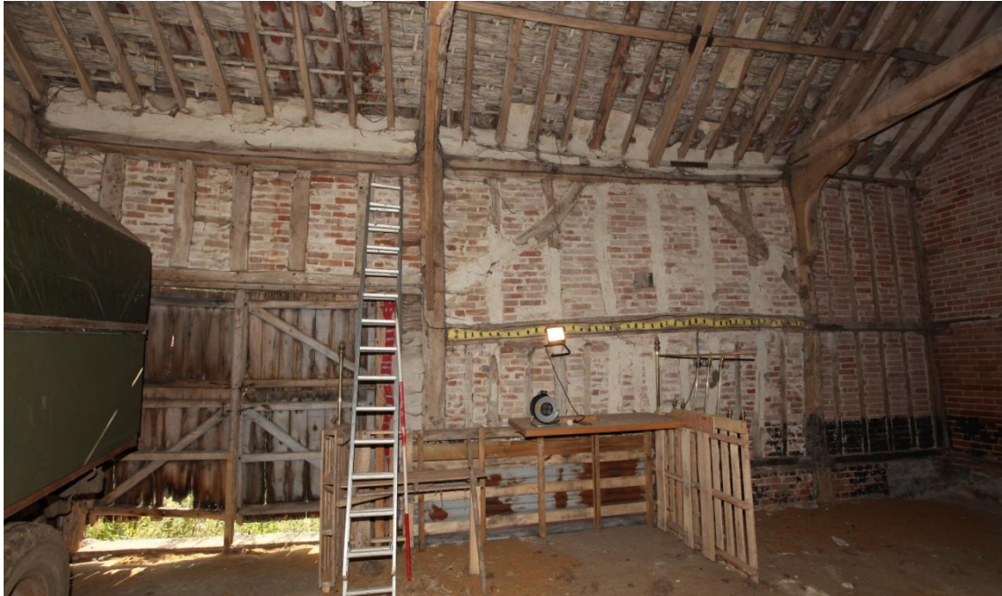
Illus. 6. The south-western interior of the original entrance bay on the left (1c) and the end-bay (1d) to right, with the 19 th century extension to the extreme right (3a). The studs and internal wall braces in bay 1d are original but the lintel of the present doors and the short studs above are later insertions that partly block the original entrance. These timbers appear to have been re-used from the porch (1e) and the lintel is a mid-rail with identical pegged mullion mortises for a central window to those in the porch's gable tie-beam and side wall. The floor is of concrete with no trace of a threshing floor.
