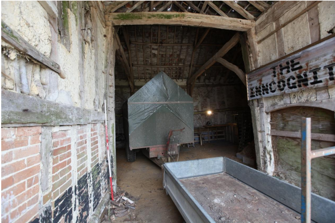
Illus. 11. The south-western truss of the porch (1e) looking towards the barn's original entrance. This bay of the barn contained a mid-rail with a solid wall above and possibly a small door in the usual fashion beneath, but the roof-plate has been cut out. The porch was open-framed against it, with jowled posts but no stud mortises in its intact tie-beam and a binding joist that was smaller than its counterpart in the external gable and is unlikely to have formed part of a ground-floor wall.
