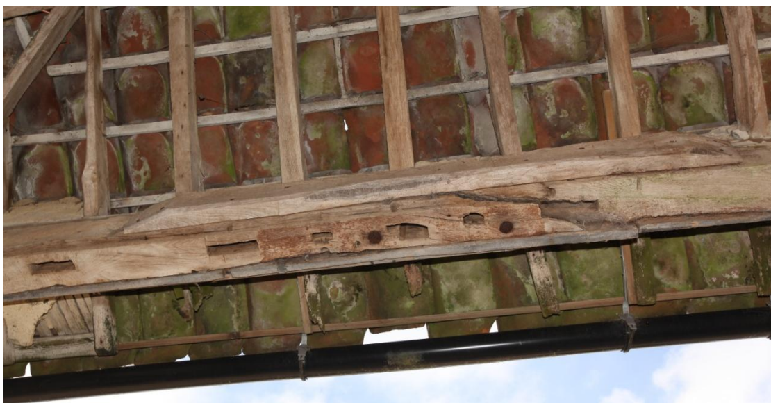
Illus. 12. A detail of the external (north-eastern) tie-beam of the porch (1e) showing empty mortises for studs on both sides of a central window lighting the missing loft with three pegged rectangular mullion mortises cut by a later housing for the locking bar of full-height barn doors. The tie-beam has split and is secured by vertical iron bolts. The corner posts of this gable contain mortises for a mid-rail that probably now forms the lintel of the barn's south-western doors and contains identical mullion mortises (A2. 6). The porch is contemporary or almost contemporary with the barn and probably formed a granary behind the threshing floor but is unique in my experience.
