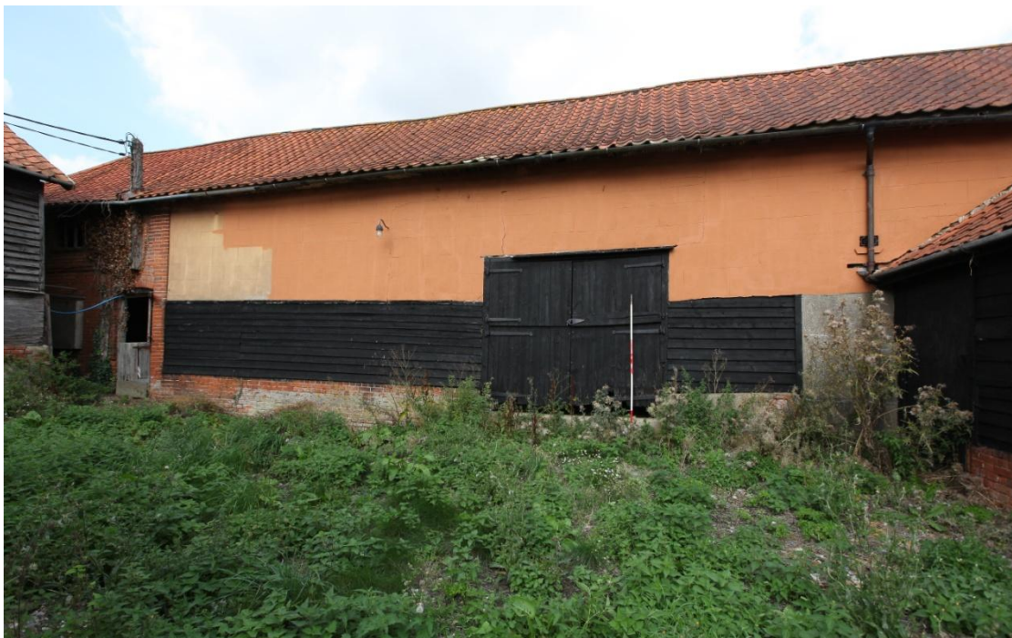
Illus. 4. The barn (1) from the south-west showing its traditional 19 th century ‘two-tier’ cladding with ashlar pargeting above tarred weatherboarding. The low doors occupy the position of the original full-height entrance to the barn’s threshing bay. Note that the brick plinth is integral to the extension (3) on the left and was renewed at the same time.
