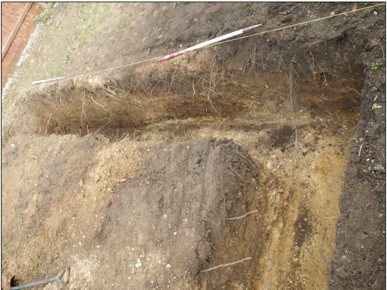
Plate 3. East and south footing trench, showing natural geology, looking north-east, 2x1m scale
