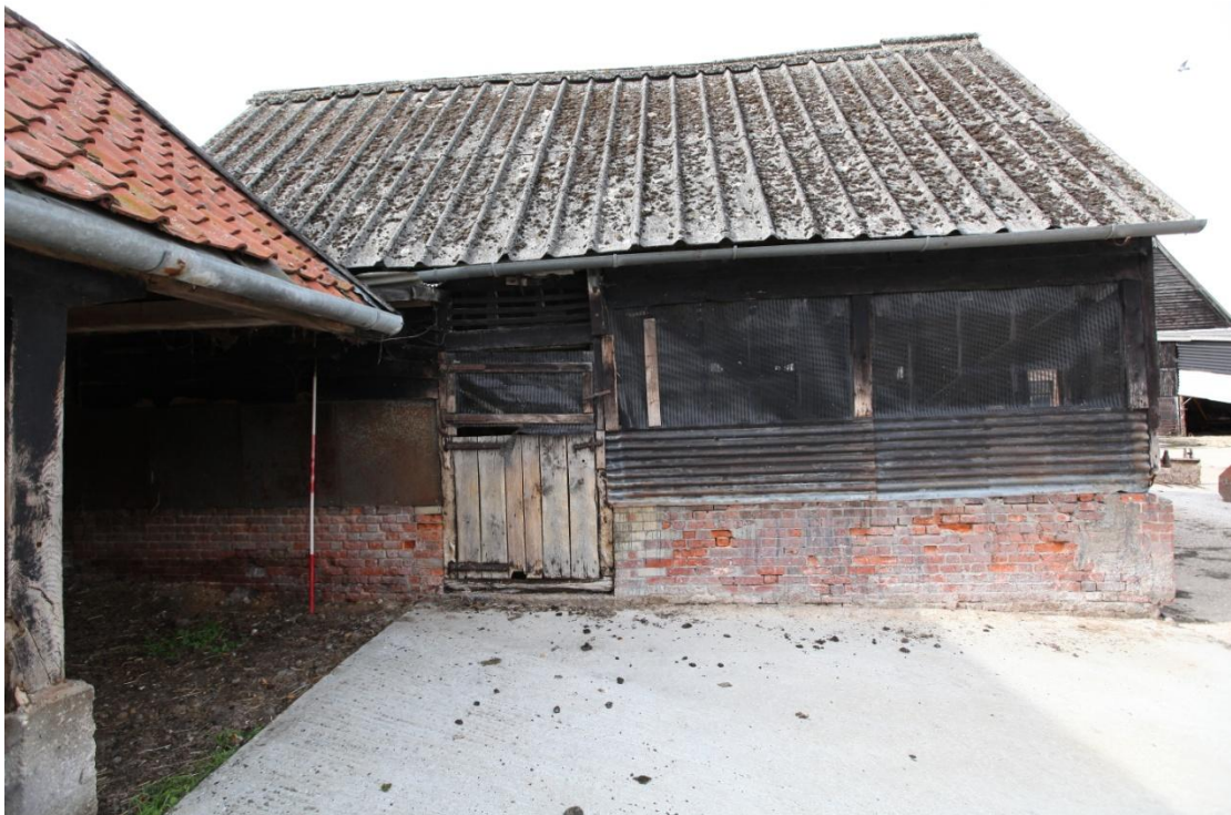
Illus. 12. The eastern facade of the stable (3) from the horse yard showing its corrugated asbestos roof and original central entrance respected by closers in the brick plinth. A tarred louver is visible above the half-hung door but the weatherboarding to the right was replaced with mesh to increase ventilation and combat pneumonia when the interior was used as a calf shed.
