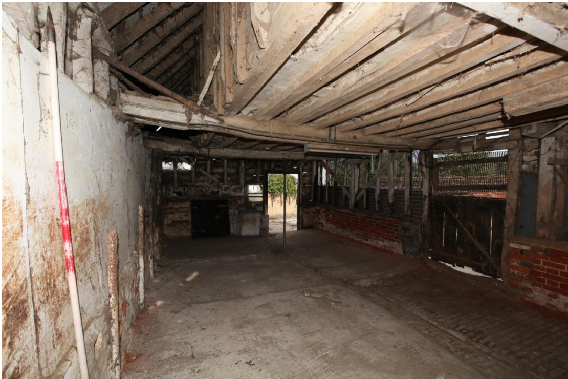
Illus. 14. The stable (3) from the south showing the western wall of the original boarded granary above. The reinforcing rails are deeper than the original principal joists they sandwich and have been neatly chamfered and curved to increase headroom above the hay rack and manger that would have adjoined the western wall on the left.
