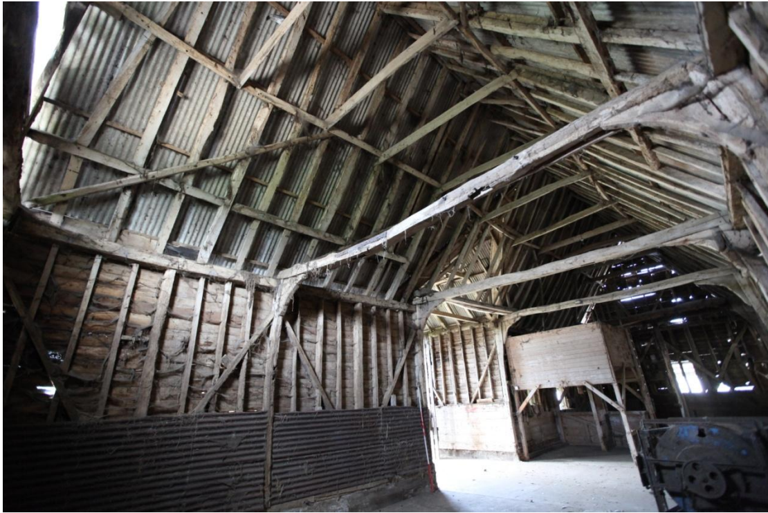
Illus. 5. The interior of the five-bay early-19 th century threshing barn (1) from the west showing the clasped-purlin roof structure with a lower tier of butt-purlins that unusually extends only over the western bays. The posts and tie-beams contain mortises for arch-braces that were replaced with knee-braces later in the 19 th century.
