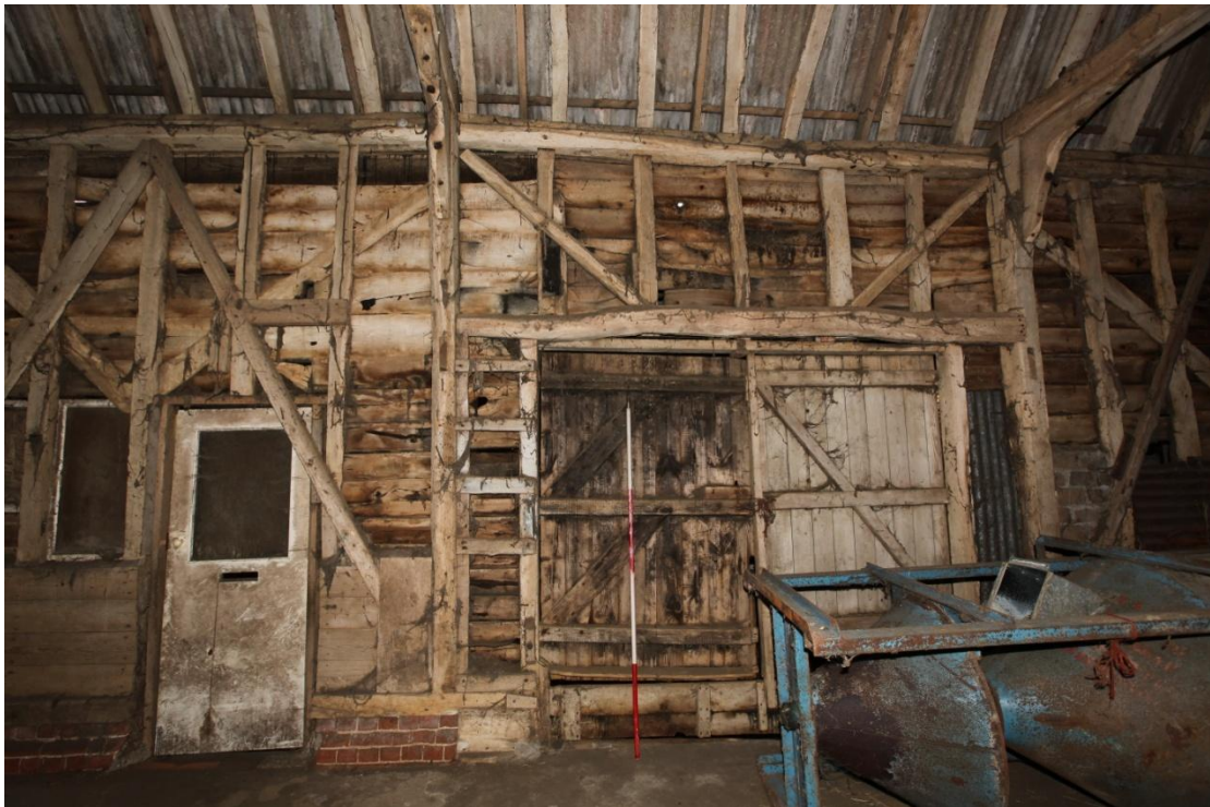
Illus. 6. The 19 th century rear doors in the southern interior of the barn's central bay (1), complete with a rare retaining board secured by vertical grooves. A number of horizontal rails indicate the presence of a former loft hence the nailed rungs of a wall ladder to the left. A notch in the storey post to the right suggests the door lintel has been raised by approximately 12 inches. The floor is now of concrete throughout.
