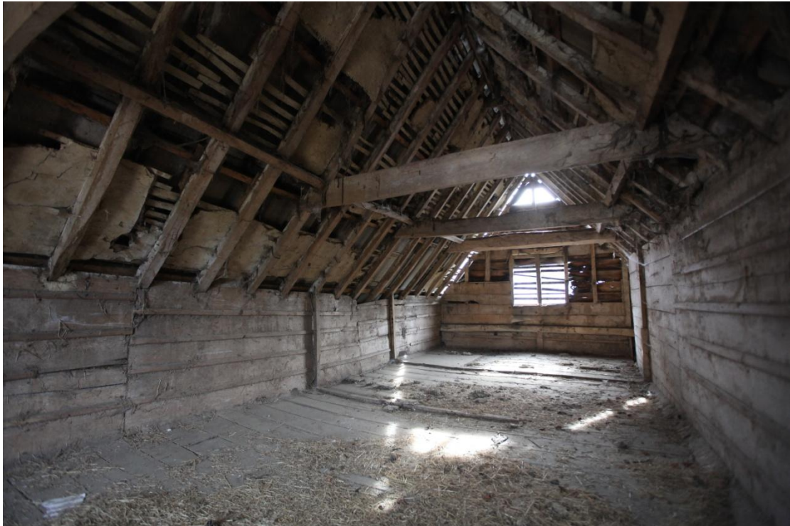
Illus. 15. The well preserved granary above the stable (3) from its northern entrance showing the original clasped-purlin roof with nailed collars and a ridge board. The roof retains a quantity of original clay plaster secured by laths to the outsides of the rafters. The original boards are sealed by fillets of wood covering their joints and there are mortises for missing grain bins in the floor. A board has been removed above the chaff box at the southern end of the right-hand wall.
