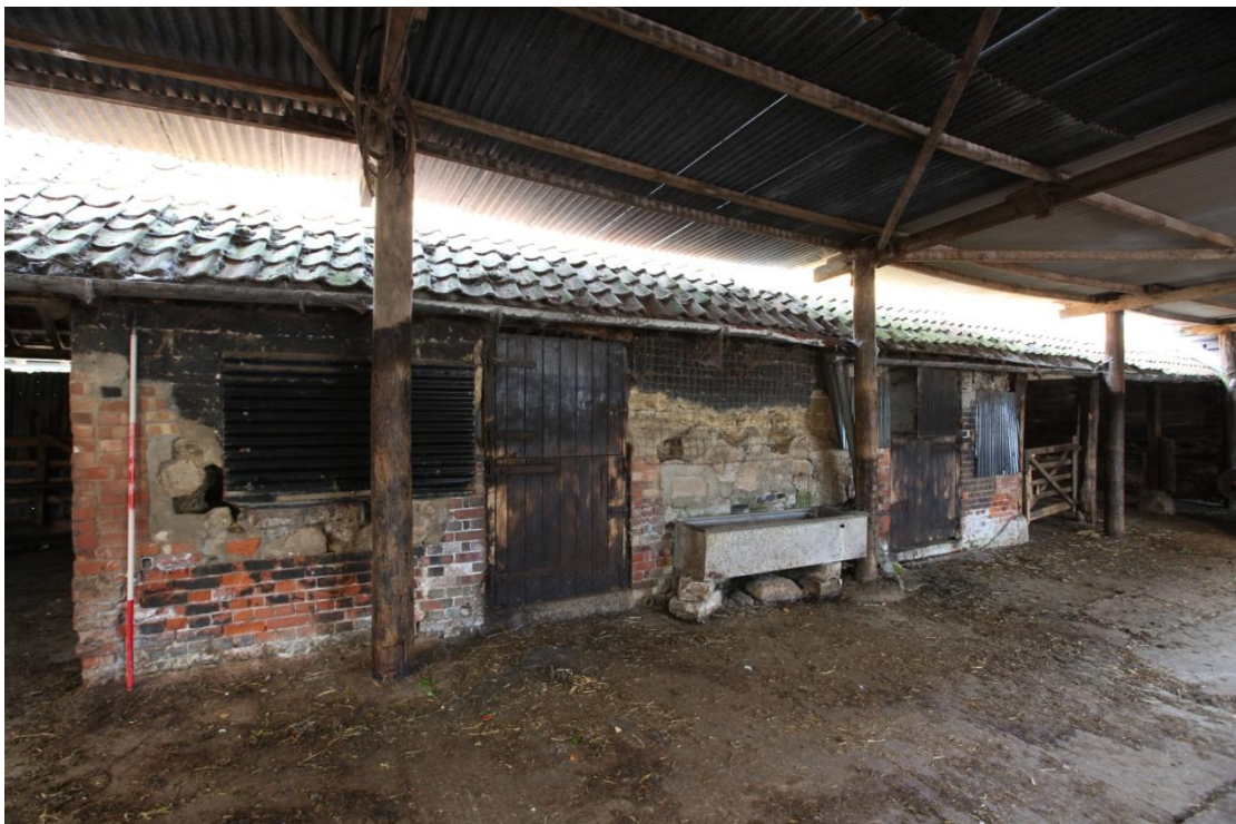
Illus. 10. The facade of the clay-lump shelter-shed (2b) from the 1970s covered cattle yard supported by telegraph poles to the east. Open-sided shelter-sheds (2a & 2c) are visible on both sides. This shed has been much altered but its original clay-lump fabric is still visible above its red-brick plinth. The interior was probably divided into two cattle boxes initially, although the present door surrounds have been largely rebuilt.
