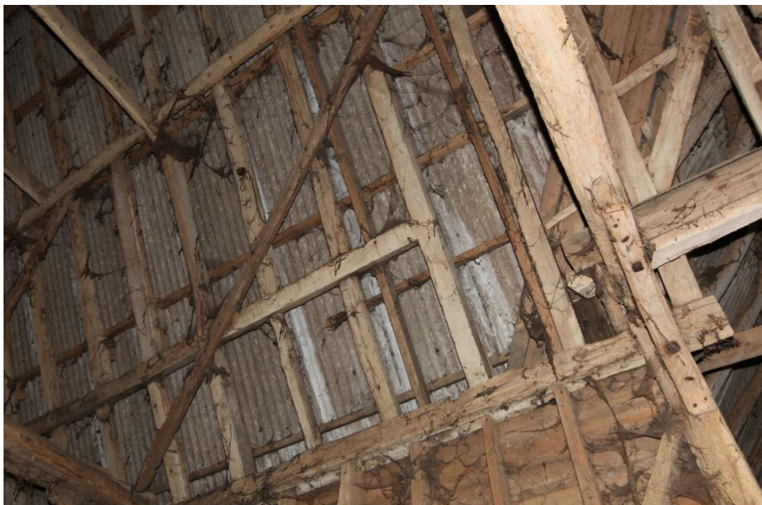
Illus. 8. The northern roof showing the lower butt-purlin terminating short of the central porch on the right. A pegged mortice in the right-hand edge of the rafter suggests it continued further but it is unclear whether this results from the use of second-hand timber or the reconstruction of the eastern section of roof in the mid-19 th century – although the former is more likely.
