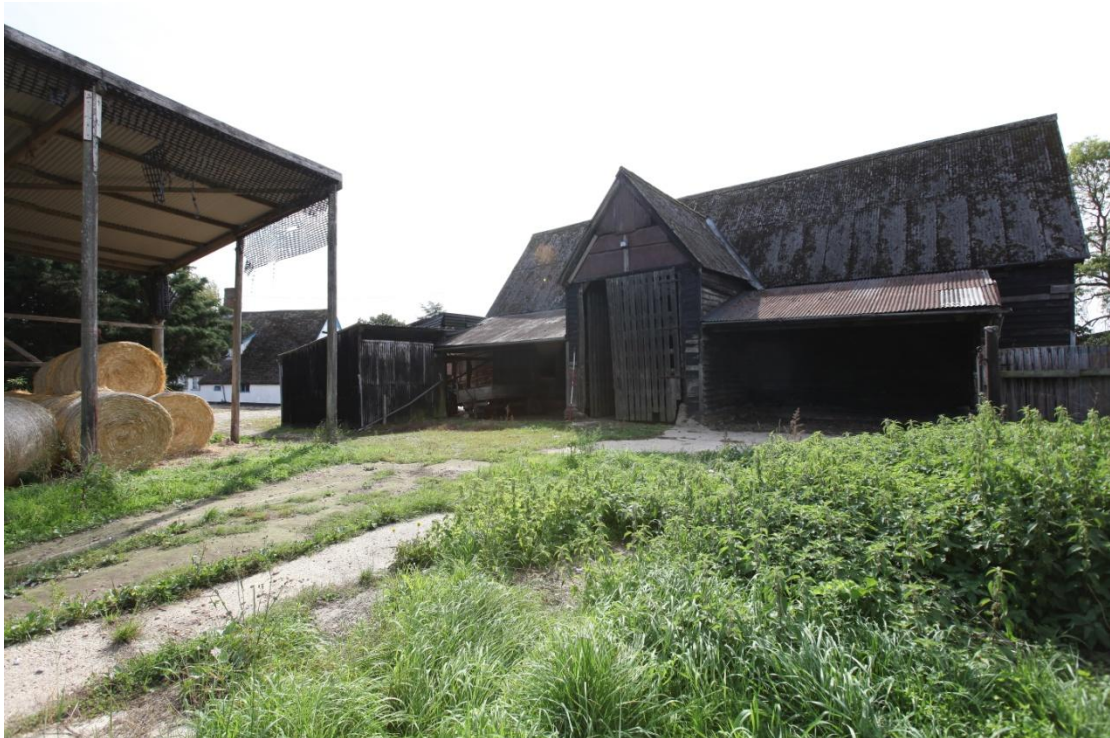
Illus. 4. The early-19th century threshing barn (1) from the north showing its corrugated asbestos roof and central entrance porch. The corrugated iron lean-to implement sheds on each side are 20 th century additions.
