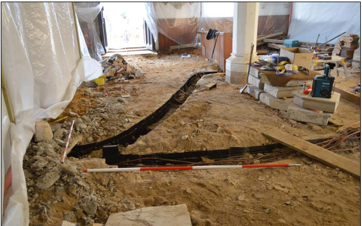
Plate 27. Heating ducts at the west end of the nave, camera facing north
