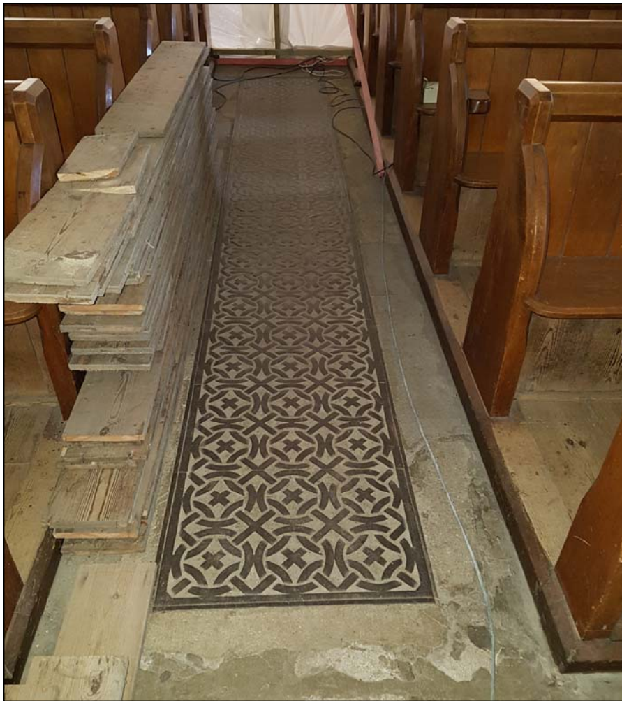
Plate 28. Cast iron panel in nave forming part of the heating system, camera facing west
