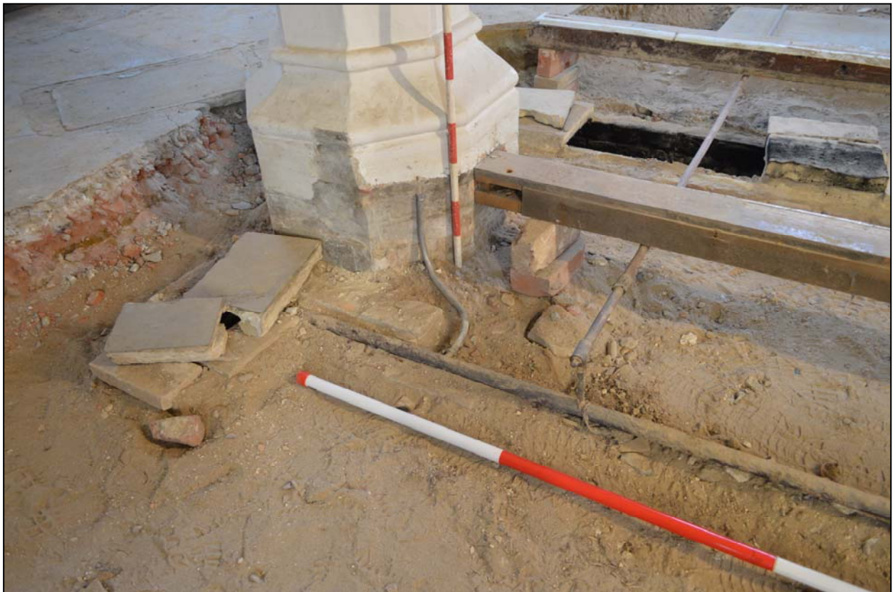
Plate 31. Gas pipes at the west end of the nave, camera facing northwest
