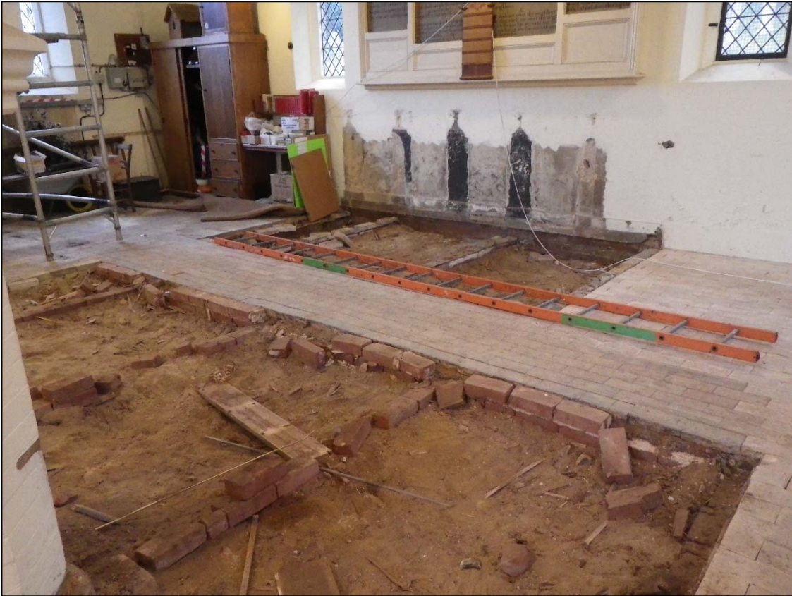
Plate 1. Area A and northern half of Area B before ground level reduction. Looking NW.
