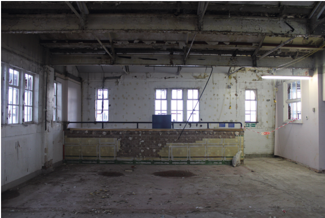
Exposed tiles on the first floor adjacent to the north stair
