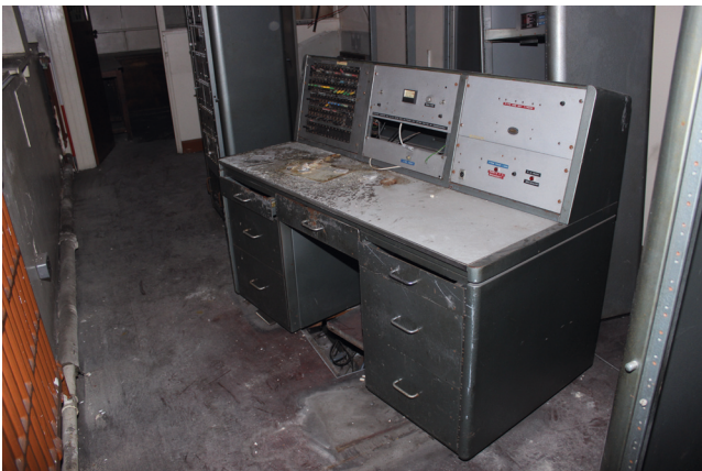
View of plant equipment ground floor room in west portion of north wing
