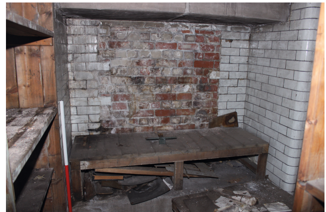
View of glazed bricks and blocked flue, potential location of a former cooking range.
