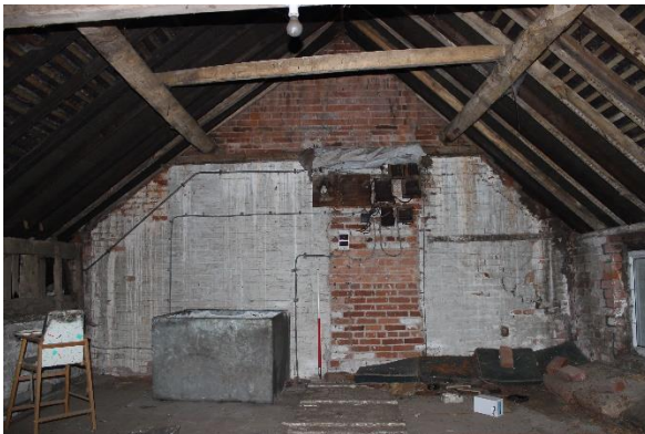
Figure 29: View of interior of loft at south end, blocked door to the rear range
