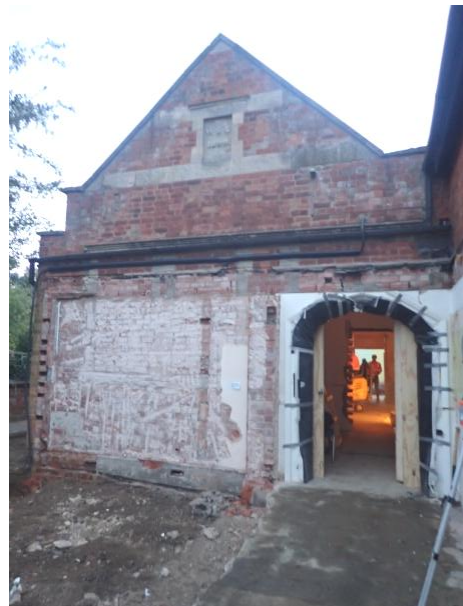
Plate 77: View of the exposed external face or north elevation of the former Sunday School building of 1899, from the north
