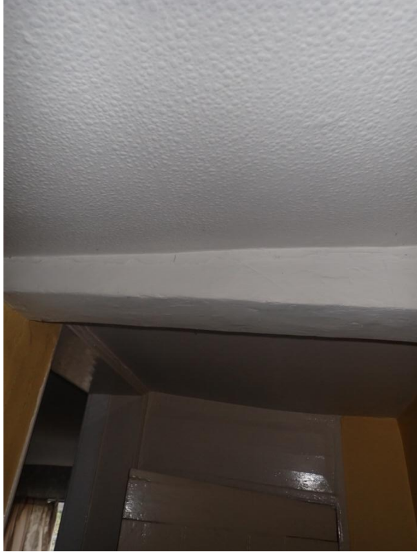
Plate 221: View of the ceiling of the first floor landing of Building 2, from the south-east
