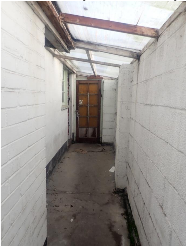
Plate 341: General view of the interior of the Corridor leading to Cell 17, from the south-west
