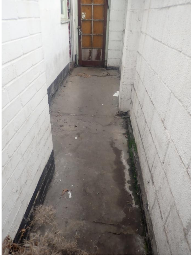
Plate 340: View of the flooring of the Corridor leading to Cell 17, from the south-west
