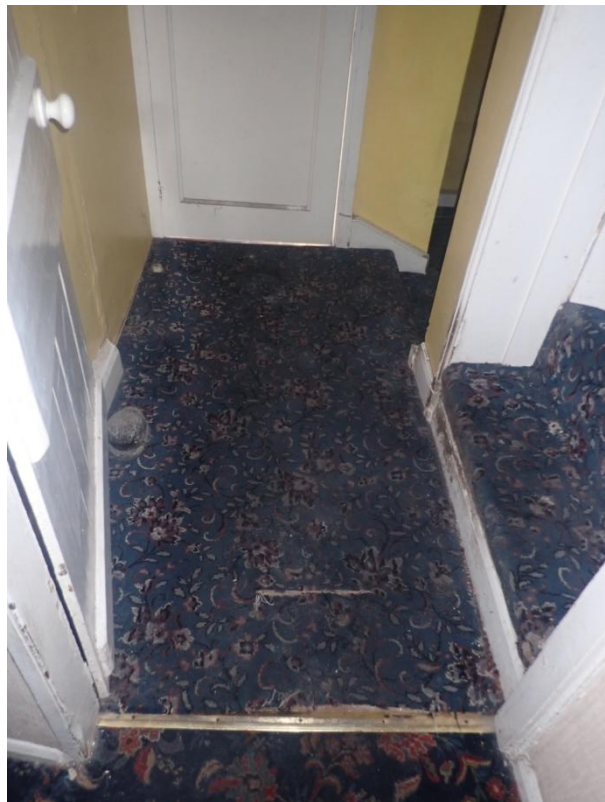
Plate 217: View of the flooring of the upper levels of the first floor landing of Building 2, from the north-west
