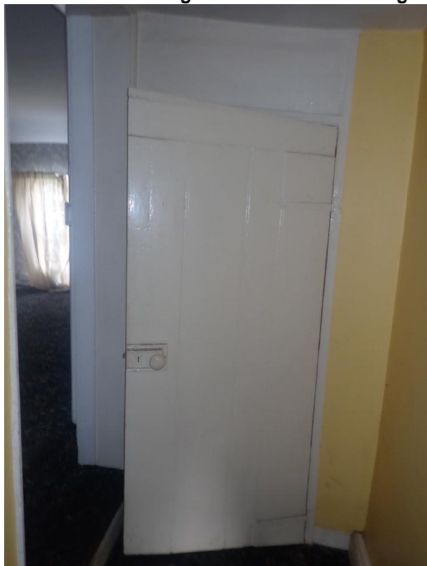
Plate 220: View of the north wall of the first floor landing of Building 2, from the south-east
