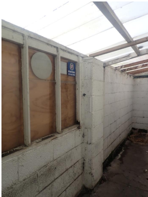
Plate 351: View of the south wall of the Corridor leading to Cell 17, from the north-east
