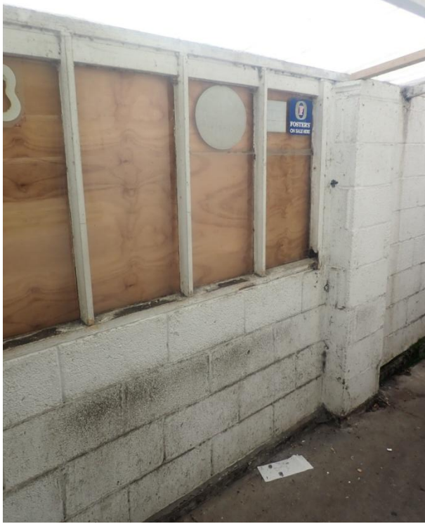
Plate 354: View of the south wall of the Corridor leading to Cell 17, from the north-east
