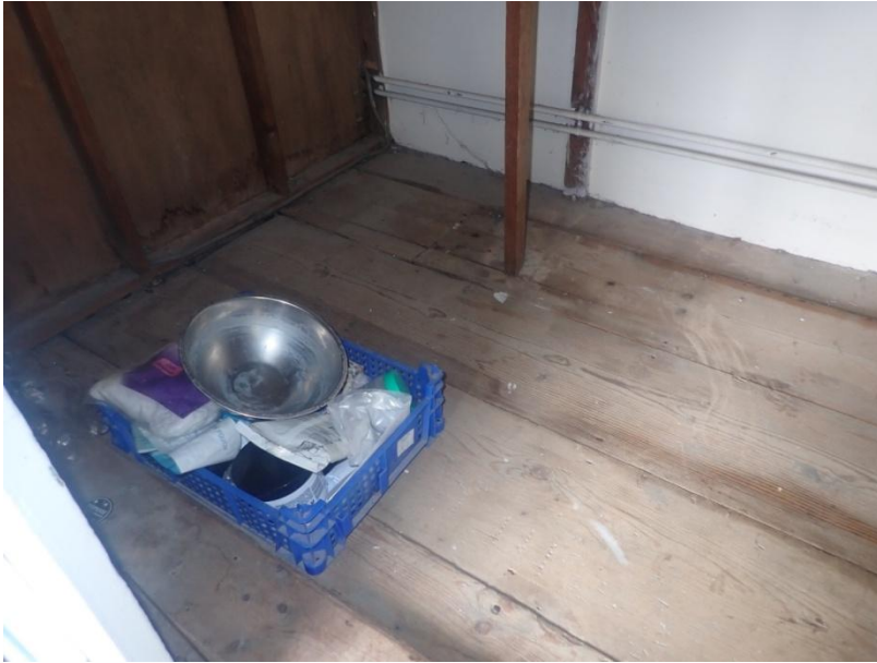
Plate 269: View of the airing cupboard within the north wall of Cell 14, from the south-east
