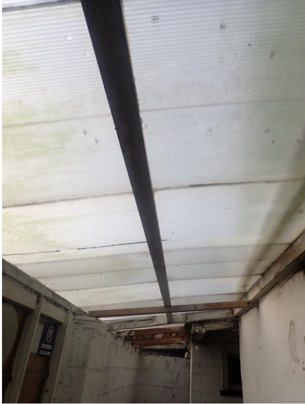
Plate 338: View of the roofing structure of the Corridor leading to Cell 17, from the north-east
