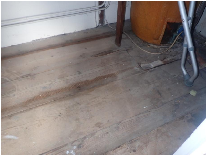
Plate 270: View of the airing cupboard within the north wall of Cell 14, from the south-west
