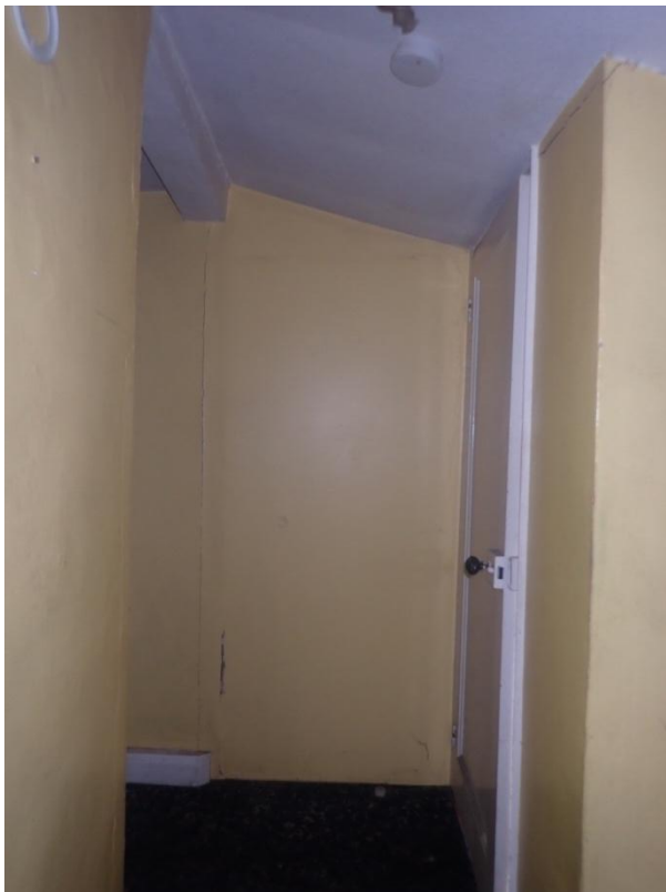
Plate 213: View of part of the east wall of the first floor landing of Building 2, from the south-west
