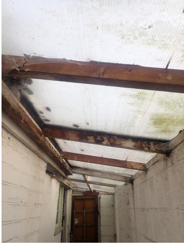
Plate 342: View of the roofing structure of the Corridor leading to Cell 17, from the south-west
