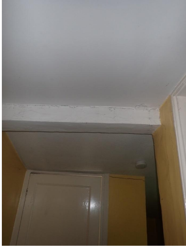
Plate 219: View of the ceiling of the first floor landing of Building 2, from the north-west
