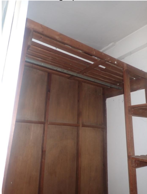
Plate 272: View of the airing cupboard within the north wall of Cell 14, from the south-west
