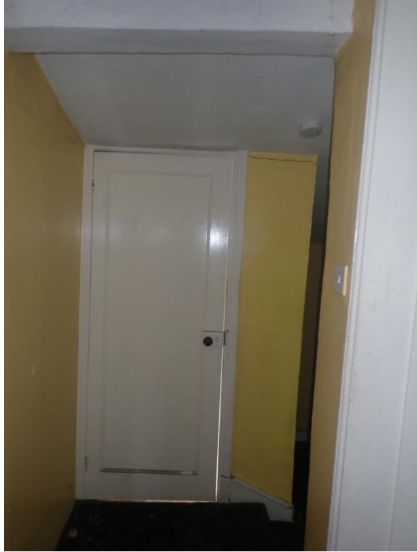
Plate 218: View of the south wall and of the ceiling of the first floor landing of Building 2, from the north-west
