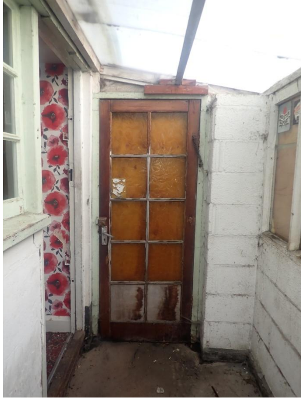
Plate 350: View of the east wall of the Corridor leading to Cell 17, from the south-west
