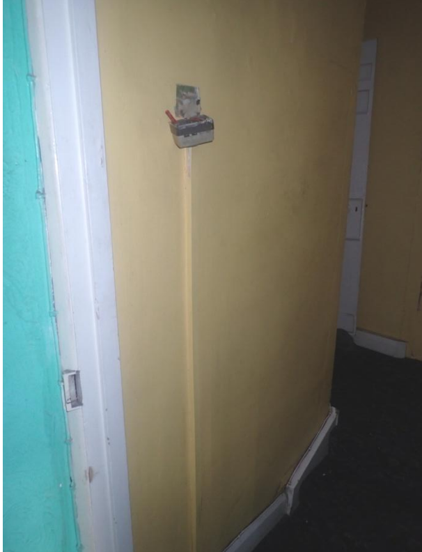
Plate 214: View of the north wall of the first floor landing of Building 2, from the south-west
