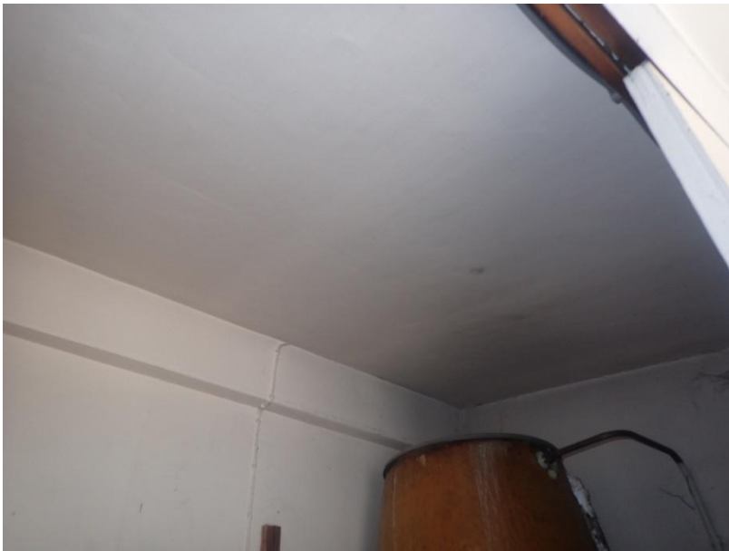
Plate 278: View of the airing cupboard within the north wall of Cell 14, from the south-west
