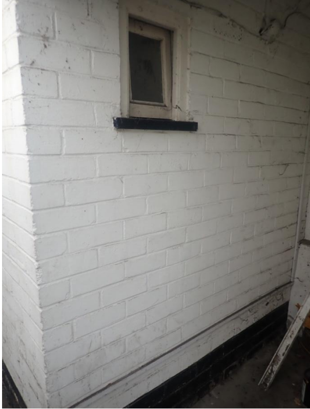
Plate 346: View of the exterior of Cell 17 within the Corridor leading to Cell 17, from the south-east
