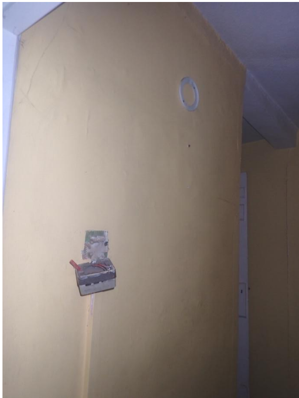
Plate 215: View of the north wall of the first floor landing of Building 2, from the south-west
