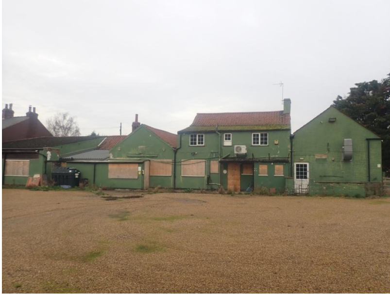
Plate 4: General view of the Duke of York public house complex, from the south
