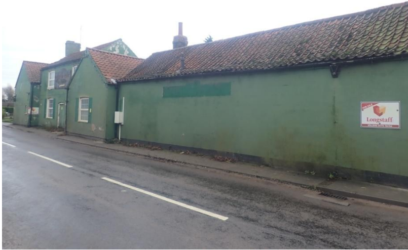
Plate 10: General view of the Duke of York public house complex, from the north-west
