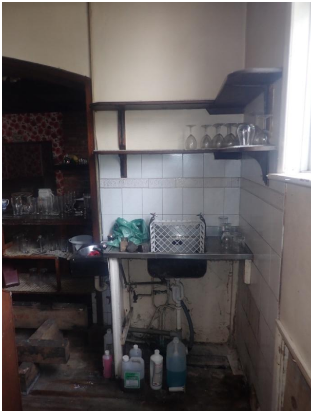
Plate 125: View of the northern portion of the west wall of Cell 6, from the north-east
