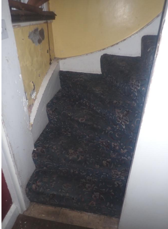
Plate 186: View of the lower levels of the stairwell of Cell 10, from the north-east
