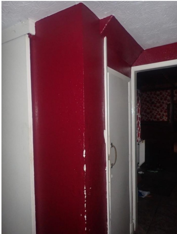
Plate 147: View of the western portion of the South Wall of Cell 7, from the north-east
