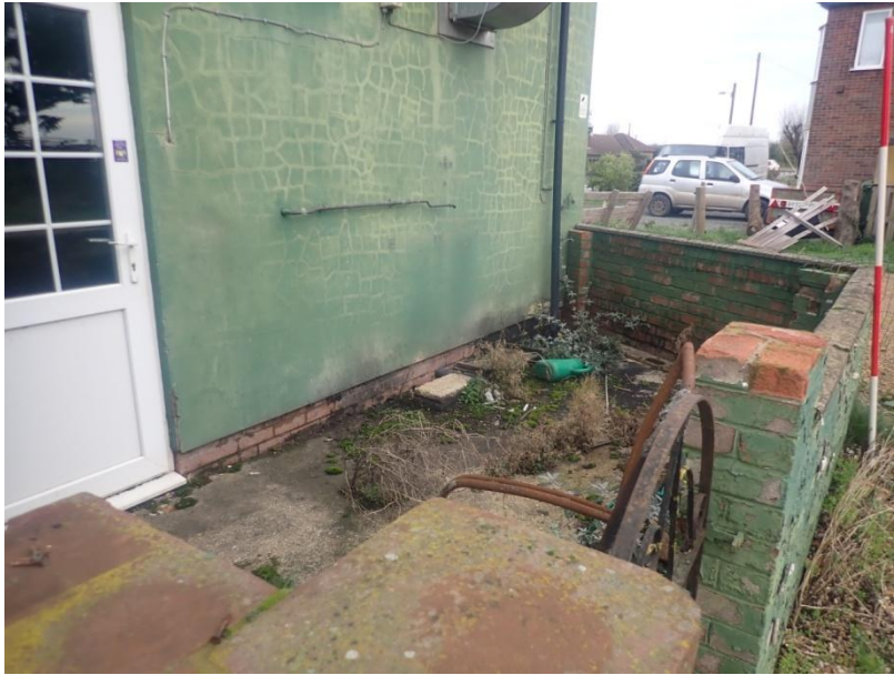
Plate 15: View of the small enclosed rear yard at the South Elevation of Building 1, from the south-west
