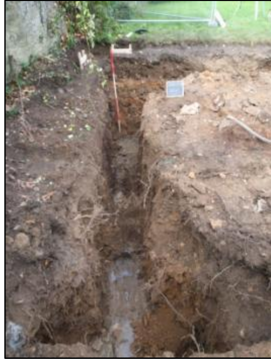
Plate 21: Completed mechanical excavation of the westerly foundation trench showing Section 2 , from the south
