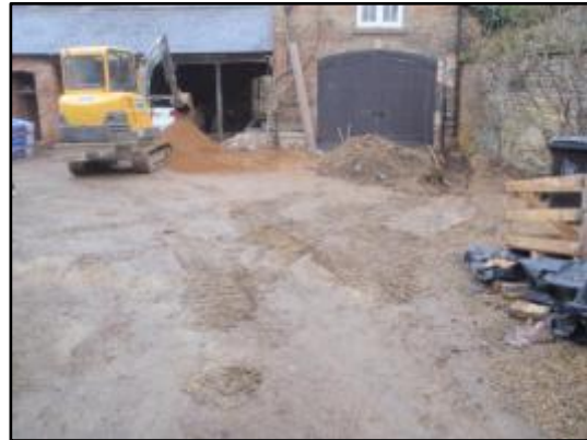
Plate 32: View of the location & extent of the first service trench & pre-groundworks, second trench, from the south
