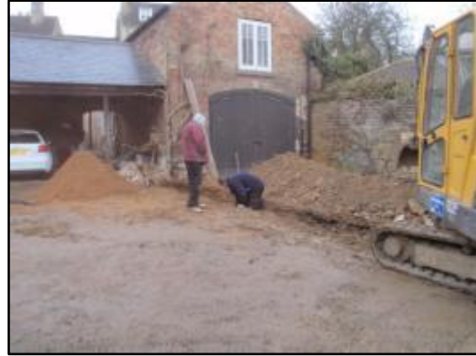
Plate 35: Work in progress, excavation of the second service trench, from the south-west
