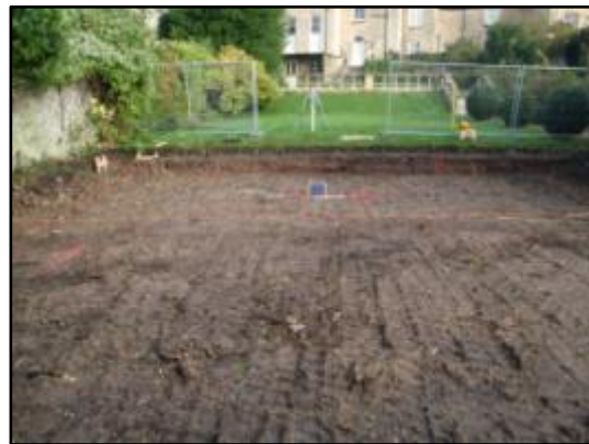
Plate 5: Set out foundations for the new build within secondary area of ground reduction, from the south
