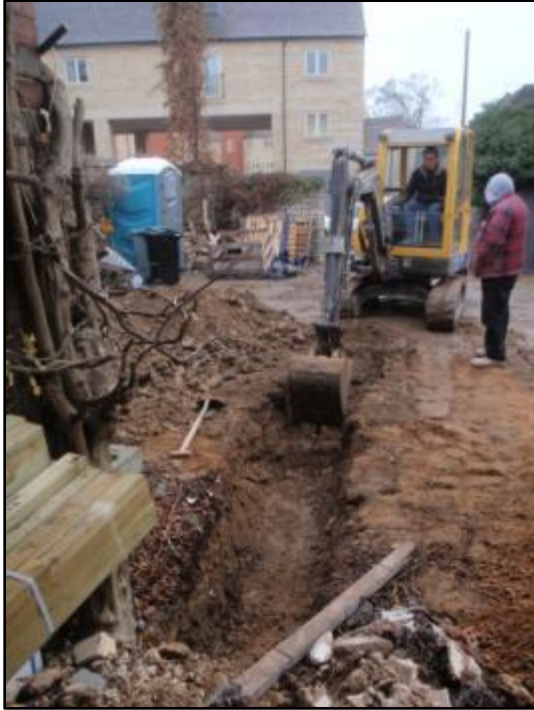
Plate 33: Work in progress, excavation of the second service trench, from the south-west
