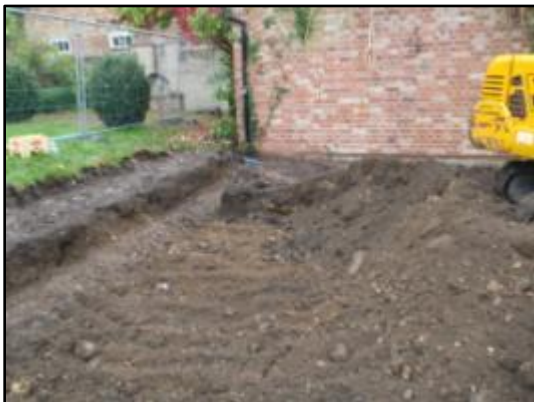
Plate 3: Secondary ground reduction, mechanical removal of the remainder of the topsoil (001) & the upper levels of the made ground deposit (002), from the west
