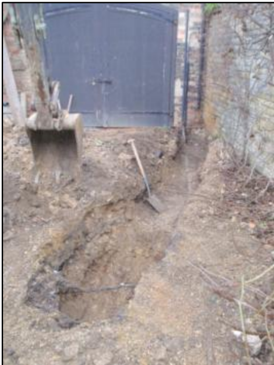
Plate 30: Work in progress, excavation of the first service trench, from the south-west
