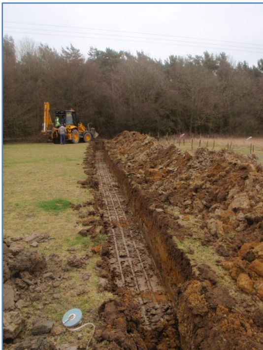
Plate 9: Work in progress,excavation of the second service trench eastwards from the soakaway, from the west
