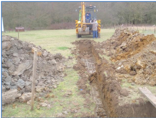
Plate 8: Work in progress,excavation of the second service trench eastwards from the soakaway, from the west
