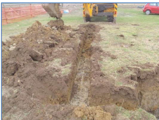
Plate 3: Work in progress,excavation of service trench northwards from the soakaway, from the south
