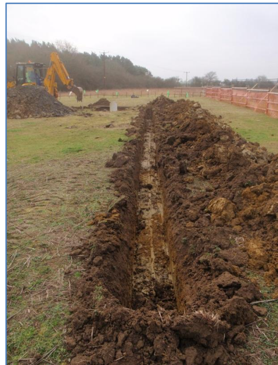
Plate 6: Work in progress,excavation of service trench northwards from the soakaway, from the north
