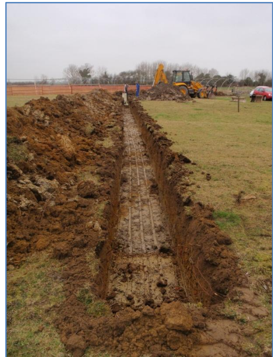
Plate 11: Work in progress,excavation of the second service trench eastwards from the soakaway, from the east
