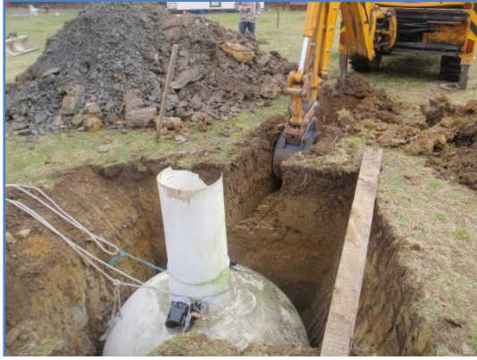
Plate 7: Work in progress,excavation of the second service trench eastwards from the soakaway, from the west
