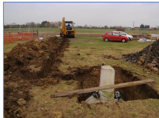
Plate 5: Work in progress,excavation of service trench northwards from the soakaway, from the south
