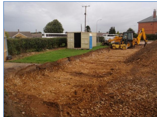
Plate 29: Area of further ground reduction within the south western corner of the area strip, from the south
