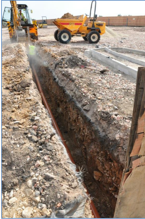
Plate 47: Excavation of a second service trench to the western side of the new build footprint, from the west
