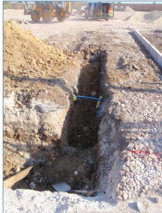
Plate 45: Excavation of a service trench for a new manhole at the western site entrance, from the west
