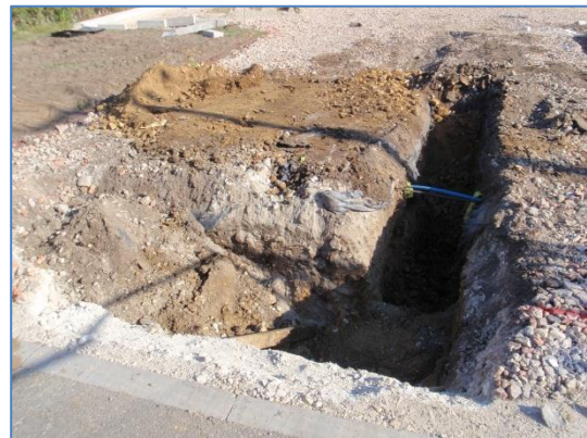
Plate 46: Excavation of a service trench for a new manhole at the western site entrance, from the west
