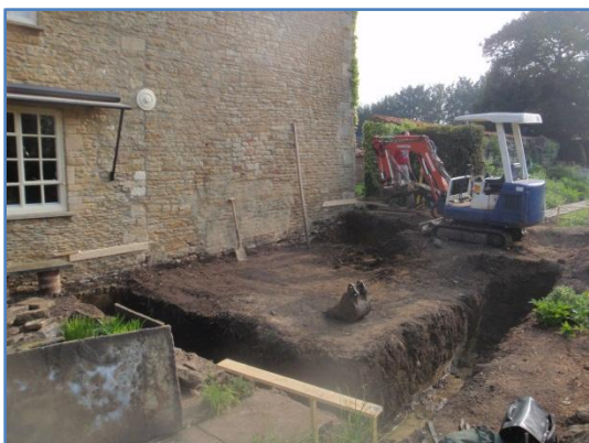
Plate 13: Work in progress, ground reduction within the new build footprint & excavation of the foundations, from the south-west
