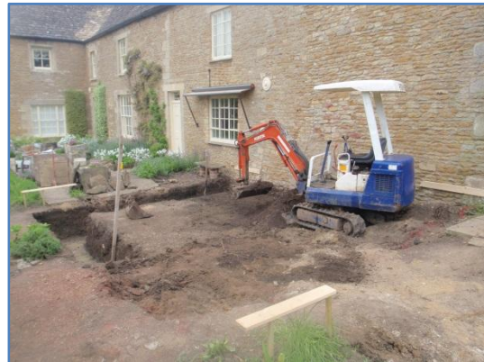
Plate 10: Work in progress, ground reduction within the new build footprint, from the east
