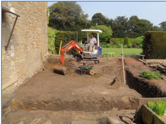
Plate 12: Work in progress, ground reduction within the new build footprint, from the west
