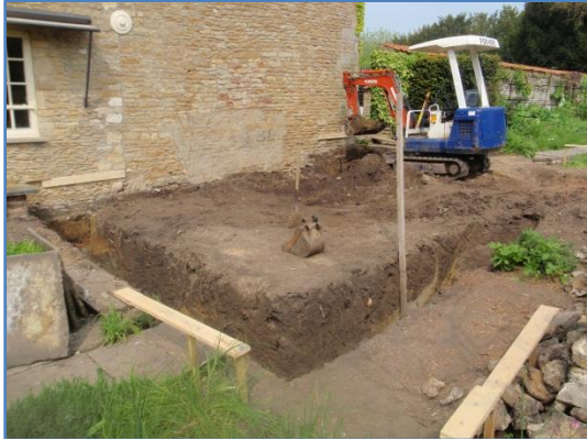
Plate 11: Work in progress, ground reduction within the new build footprint, from the south
