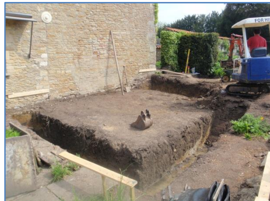
Plate 15: Work in progress, ground reduction within the new build footprint & excavation of the foundations, from the south-west
