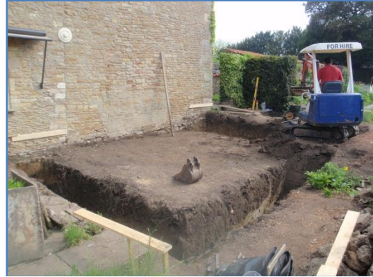
Plate 14: Work in progress, ground reduction within the new build footprint & excavation of the foundations, from the south-west
