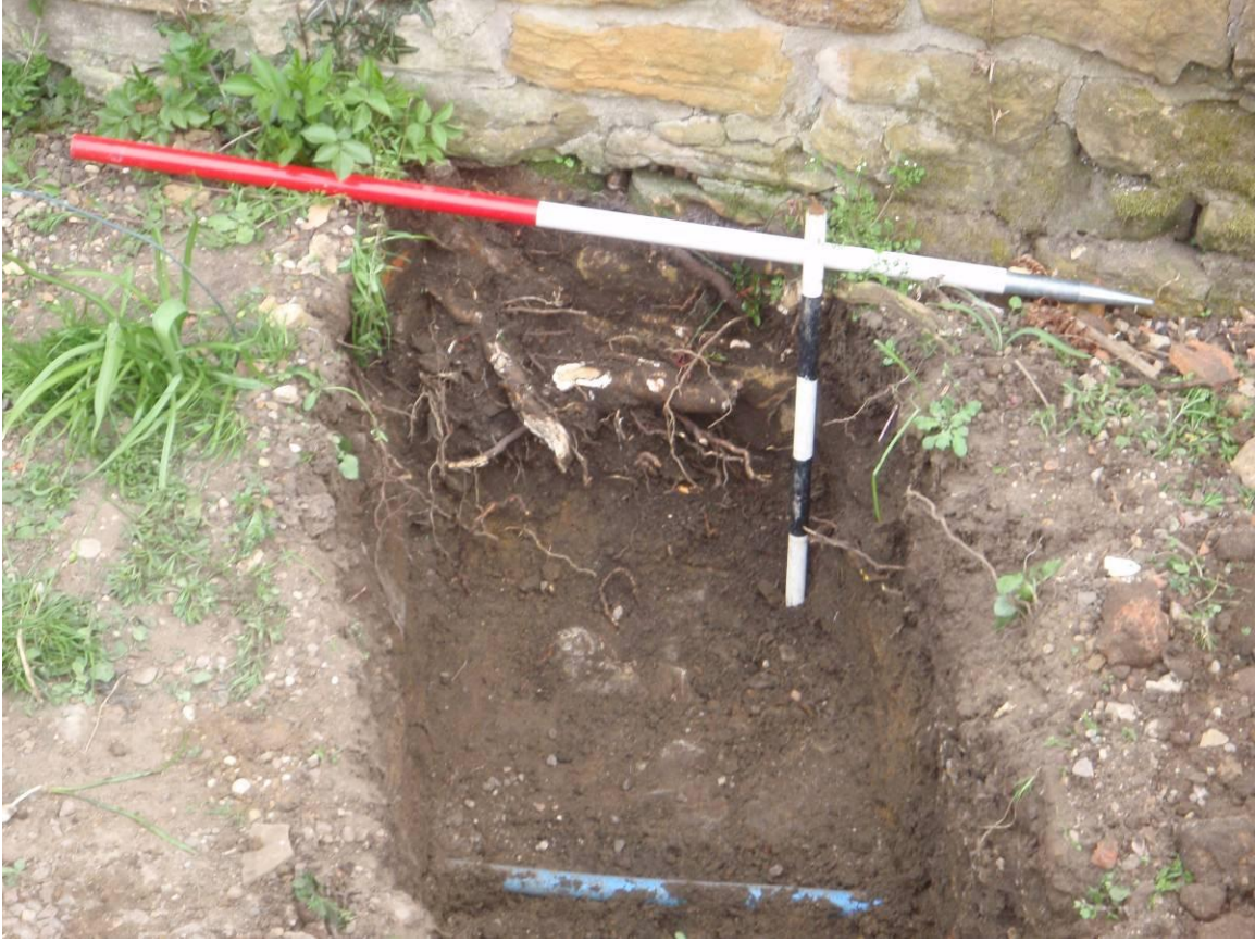
Plate 5: Exposed Foundations of the west wall of the Cart Shed, from the west
