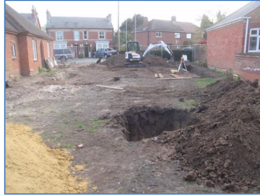
Plate 30: Location of the completed soakaway in relation to the excavated foundations from the south-west
