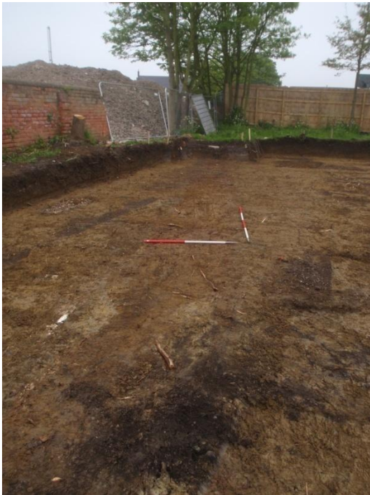
Plate 12: Ground reduction, showing the line of the ditch cut [005], from the south
