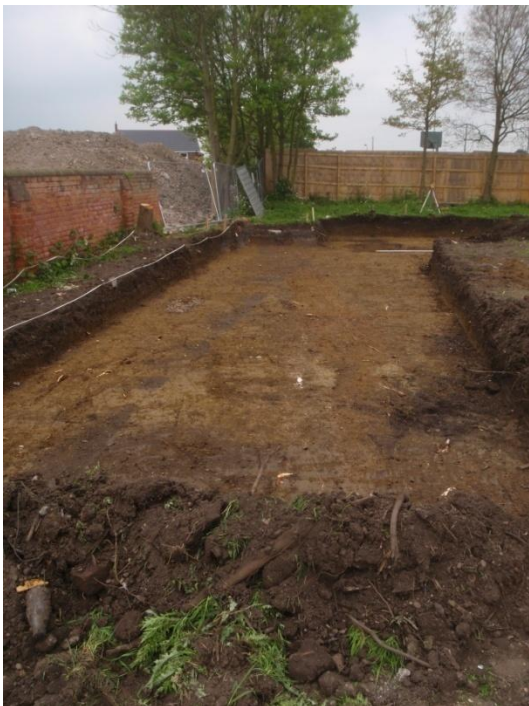
Plate 8: Ground reduction, showing the line of the ditch cut [005], from the south
