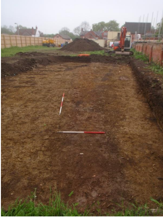
Plate 11: Ground reduction, showing the line of the ditch cut [005], from the north
