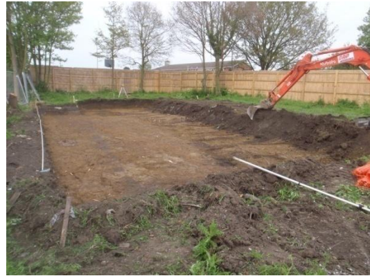
Plate 9: Ground reduction, showing the line of the ditch cut [005] from the south
