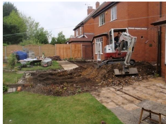
Plate 5: Ground reduction to the east of the rear extension, from the east
