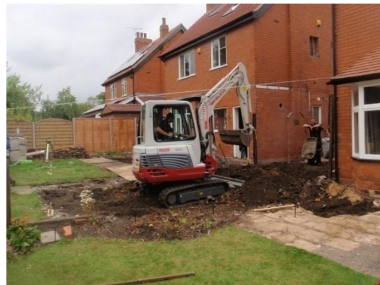
Plate 6: Ground reduction to the east of the rear extension, from the east
