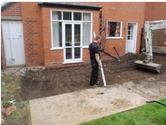
Plate 3: Ground reduction within the build footprint of the rear extension, from the south
