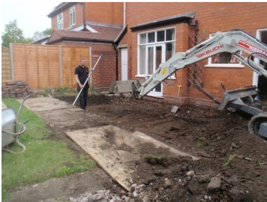
Plate 2: Ground reduction within the build footprint of the rear extension, from the east
