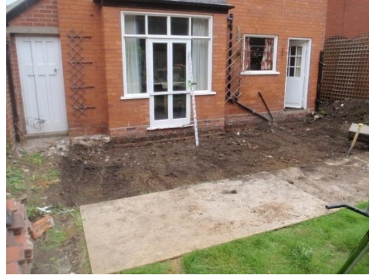
Plate 4: Ground reduction within the build footprint of the rear extension, from the south
