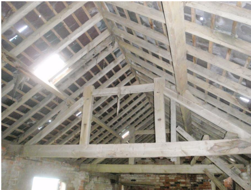
Plate 26: View of the remainder of the roof within Cell 1, from the west
