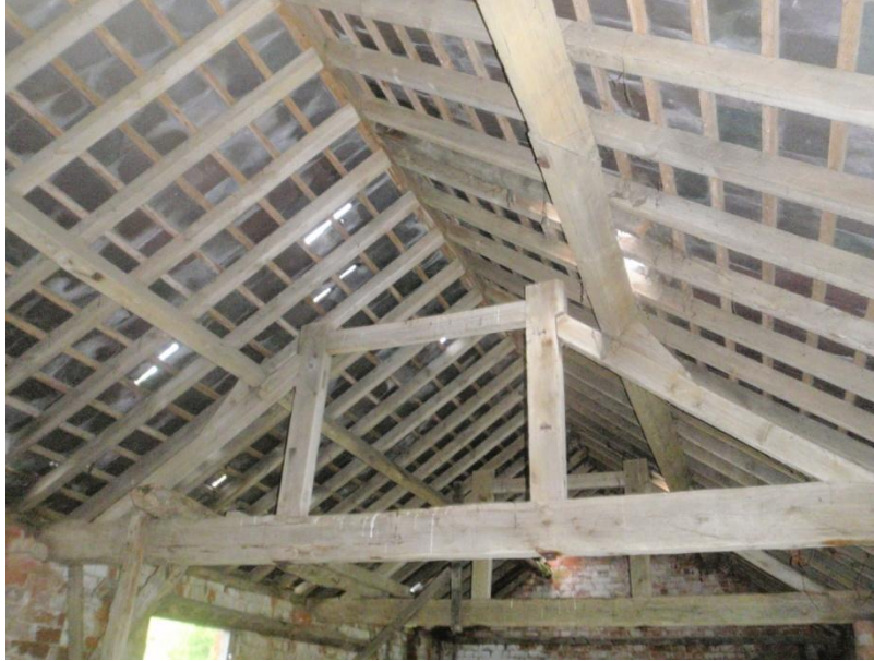
Plate 25: View of the remainder of the roof within Cell 1, from the east
