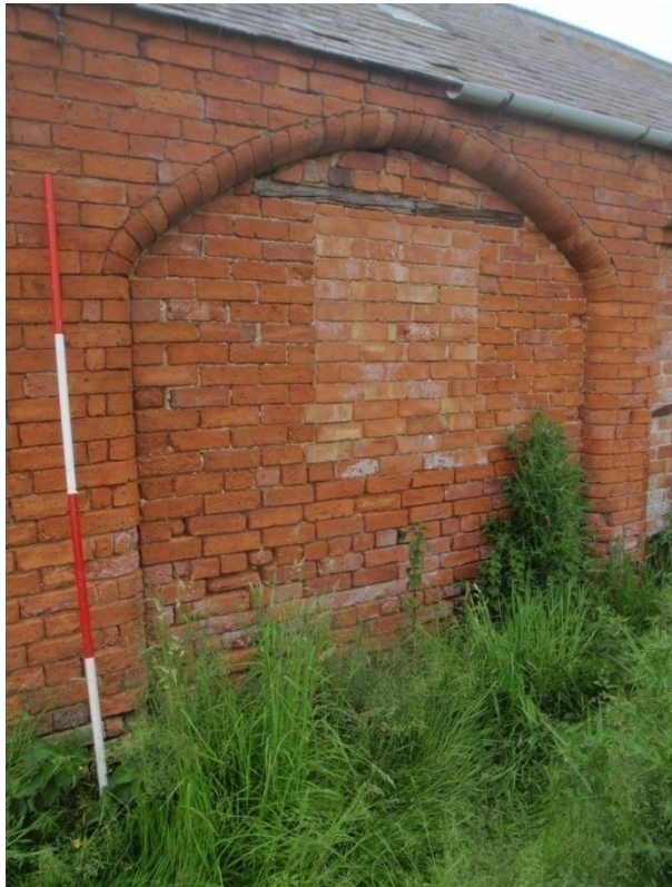
Plate 7: Detail: Infilled brick arch with infilled former window opening, from the south-west.
