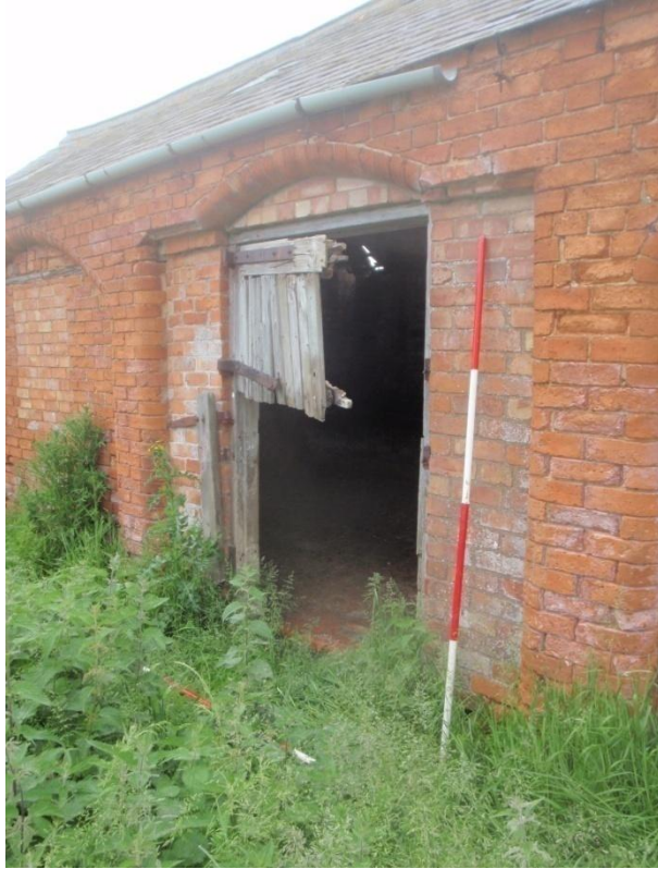
Plate 8: Detail: original arched entrance opening, infilled with modern brickwork and modern door opening, from the south-east
