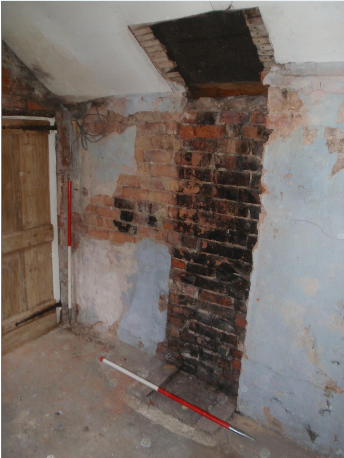
Plate 18: North wall of the first floor interior, Side Extension, from the south
