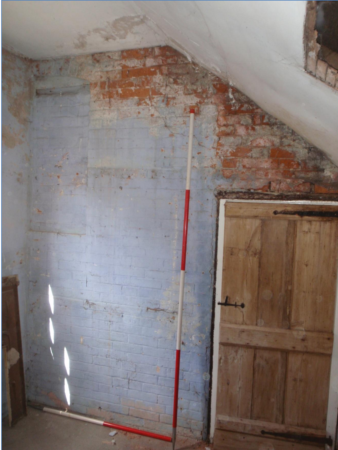
Plate 16: West wall of the first floor interior, Side Extension, from the east
