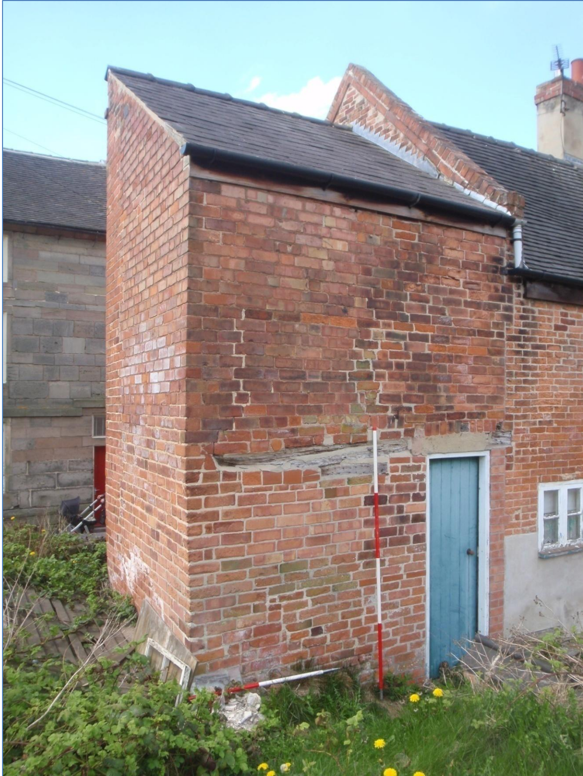
Plate 7: Rear Elevation of the Side Extension to 9, Apiary Gate, from the north
