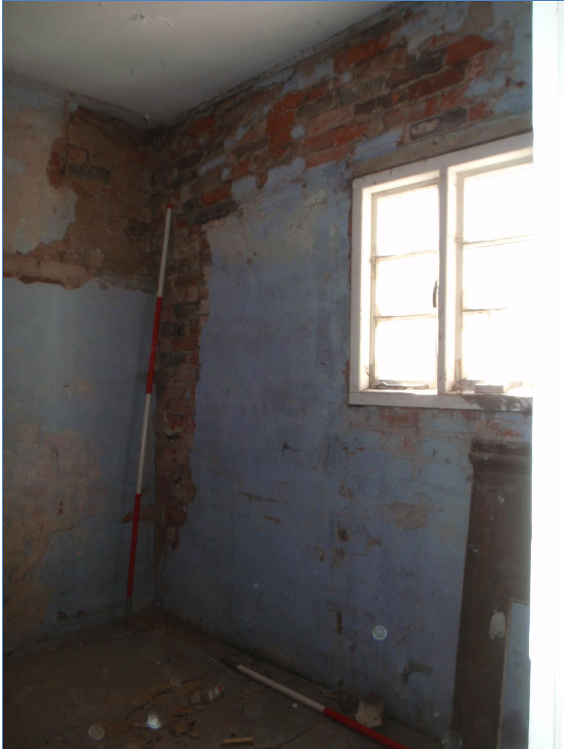
Plate 17: South wall of the first floor interior, Side Extension, from the north-west
