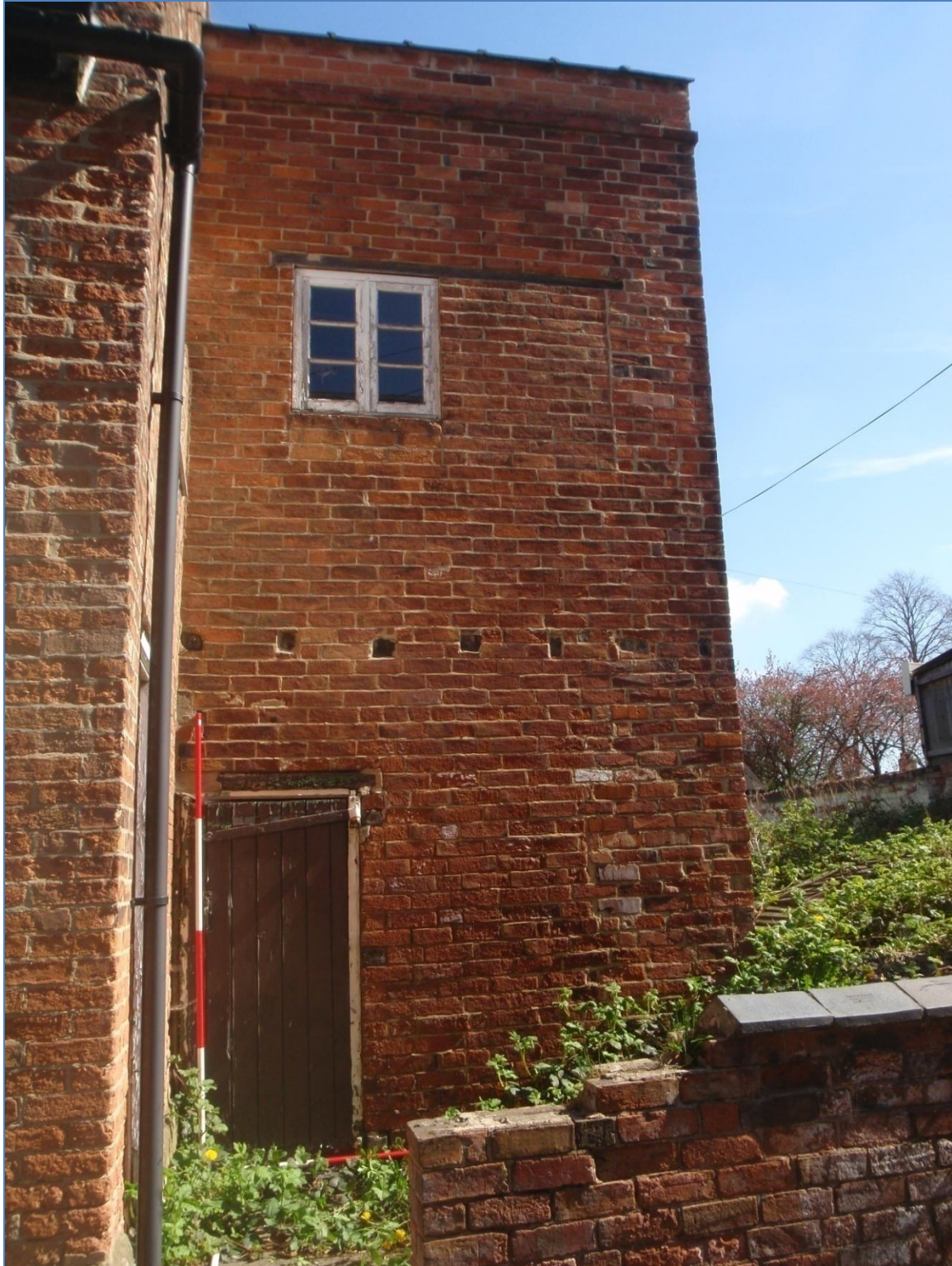
Plate 5: Front Elevation of the Side Extension to 9, Apiary Gate, from the south
