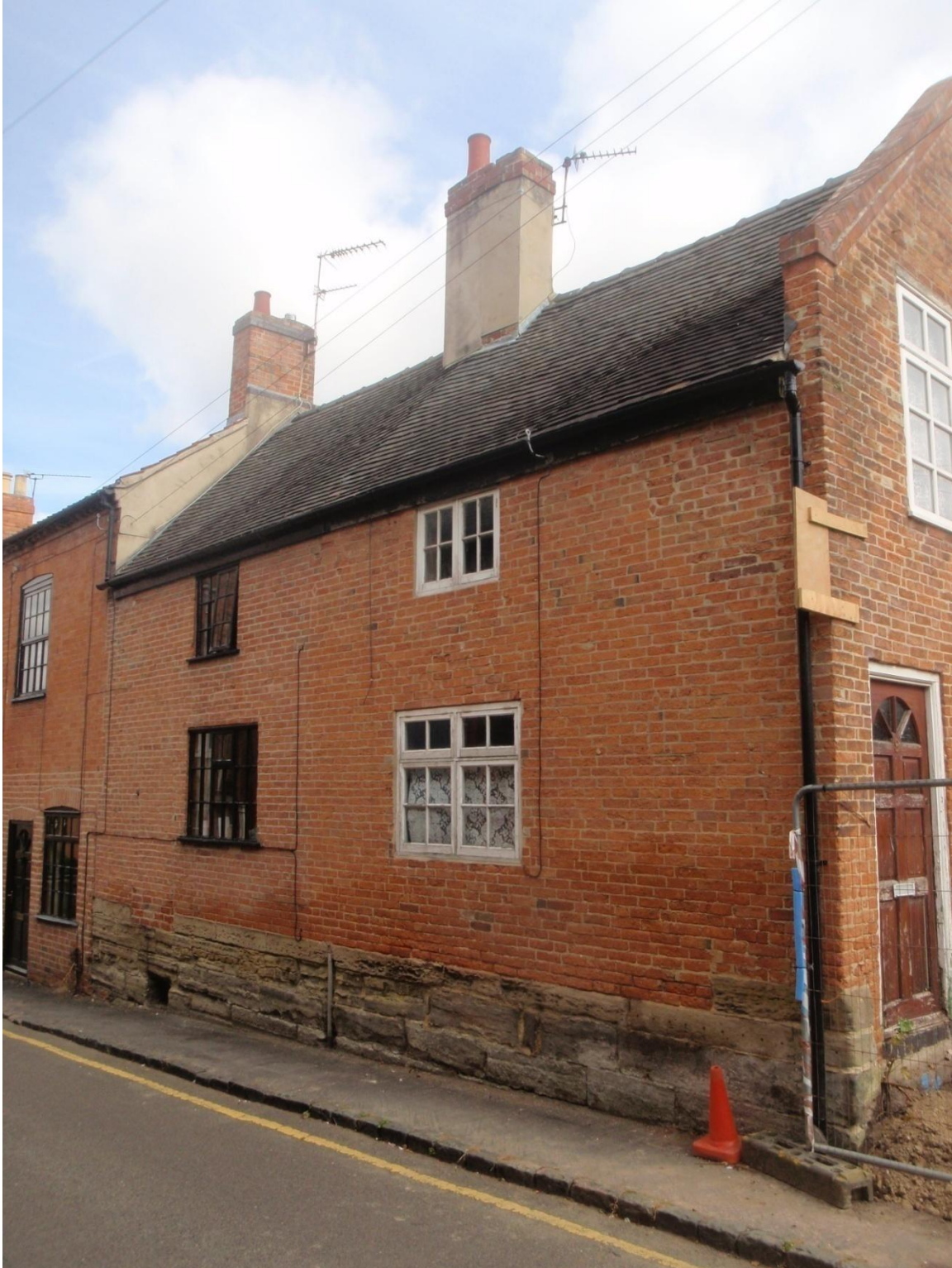
Plate 32: View of the Front (South) Elevation of 9, Apiary Gate, from the south-east
