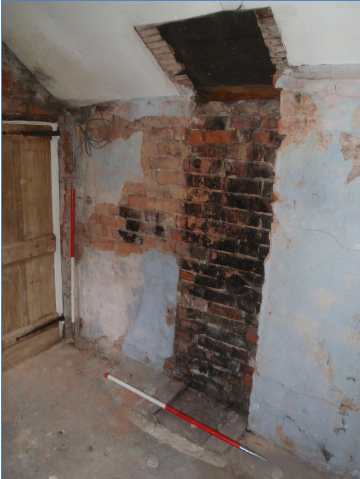
Plate 19: North wall of the first floor interior, Side Extension, from the south
