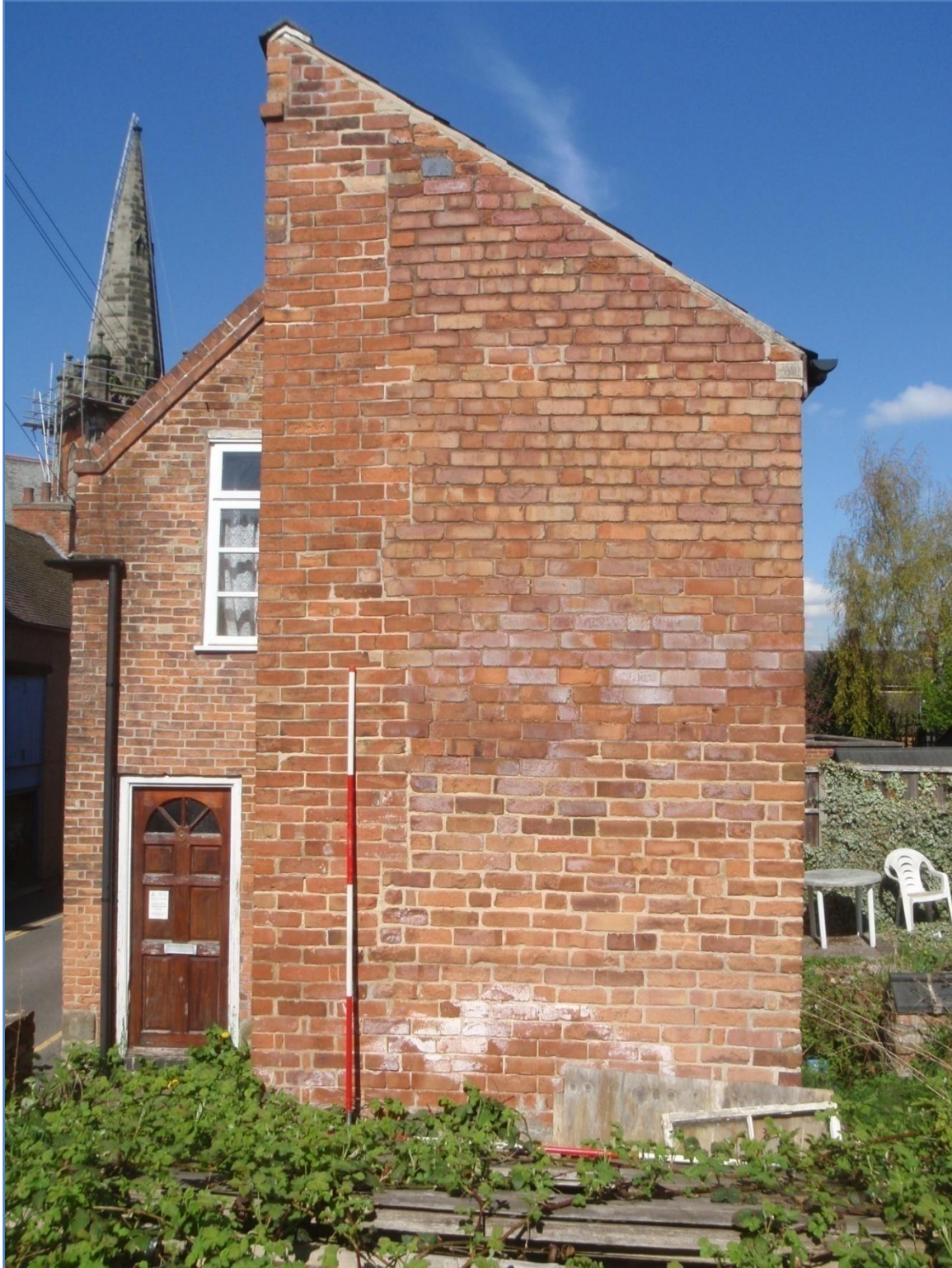
Plate 6: Side (East) Elevation of the Side Extension to 9, Apiary Gate, from the east
