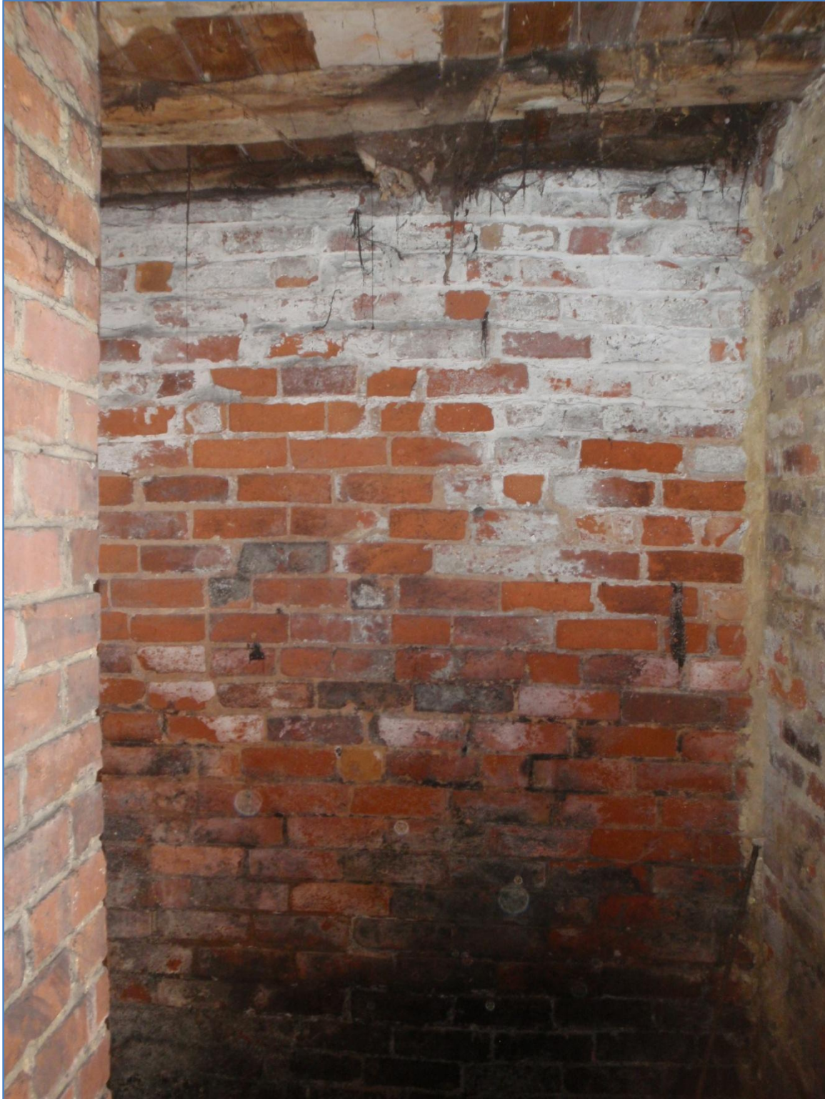
Plate 21: East wall of second ground floor room, Side Extension, from the west
