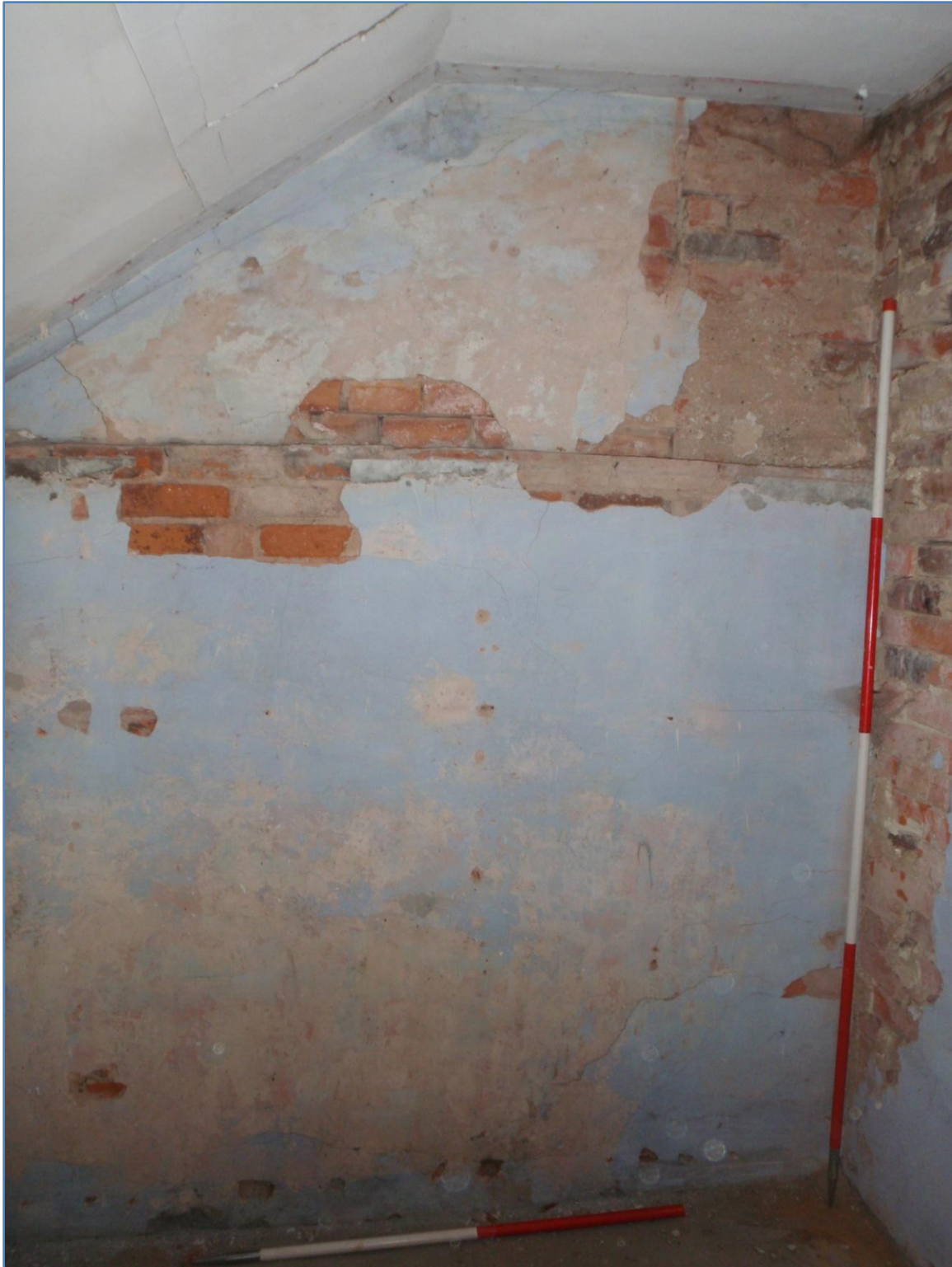
Plate 16: East wall of the first floor interior, Side Extension, from the west
