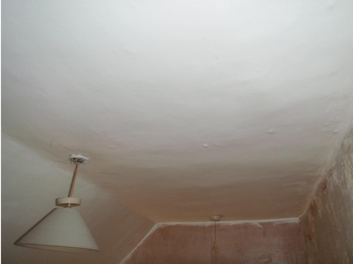
Plate 51: View of the ceiling of the first floor bathroom, from the west
