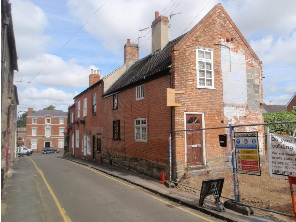
Plate 31: View of the newly exposed Side (East) Elevation and the Front (South) Elevation of 9, Apiary Gate, from the south-east
