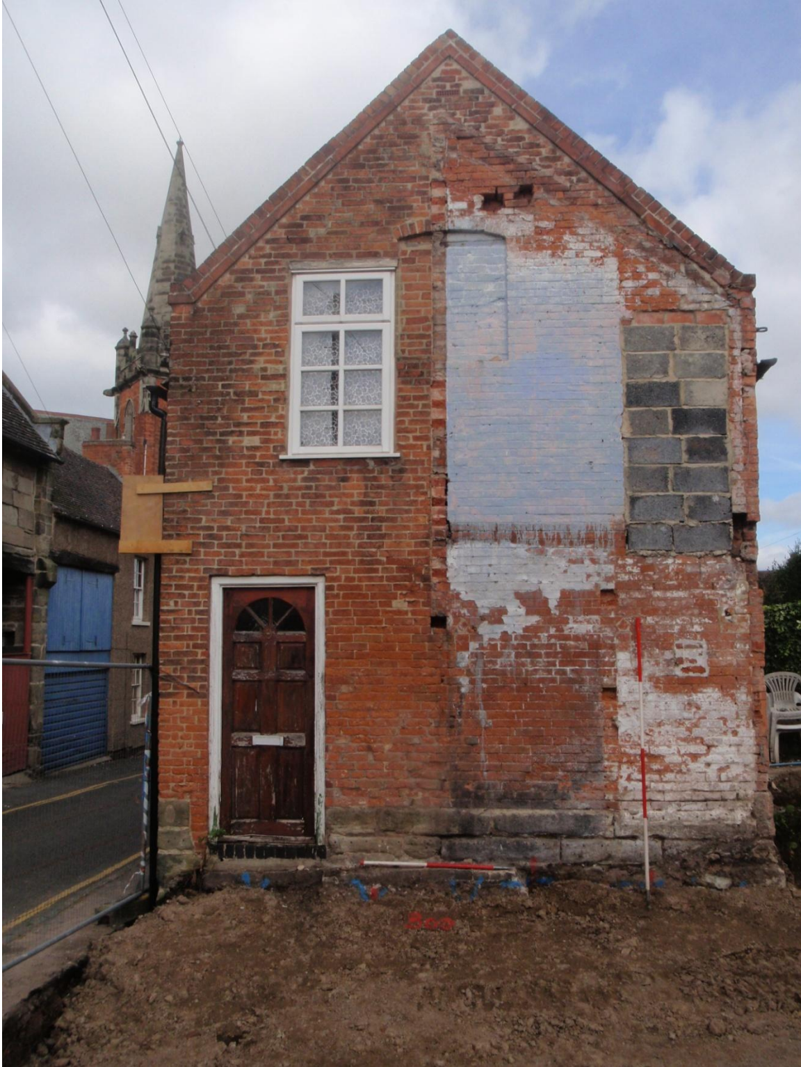
Plate 29: View of the newly and fully exposed Side (East) Elevation of 9, Apiary Gate, from the east
