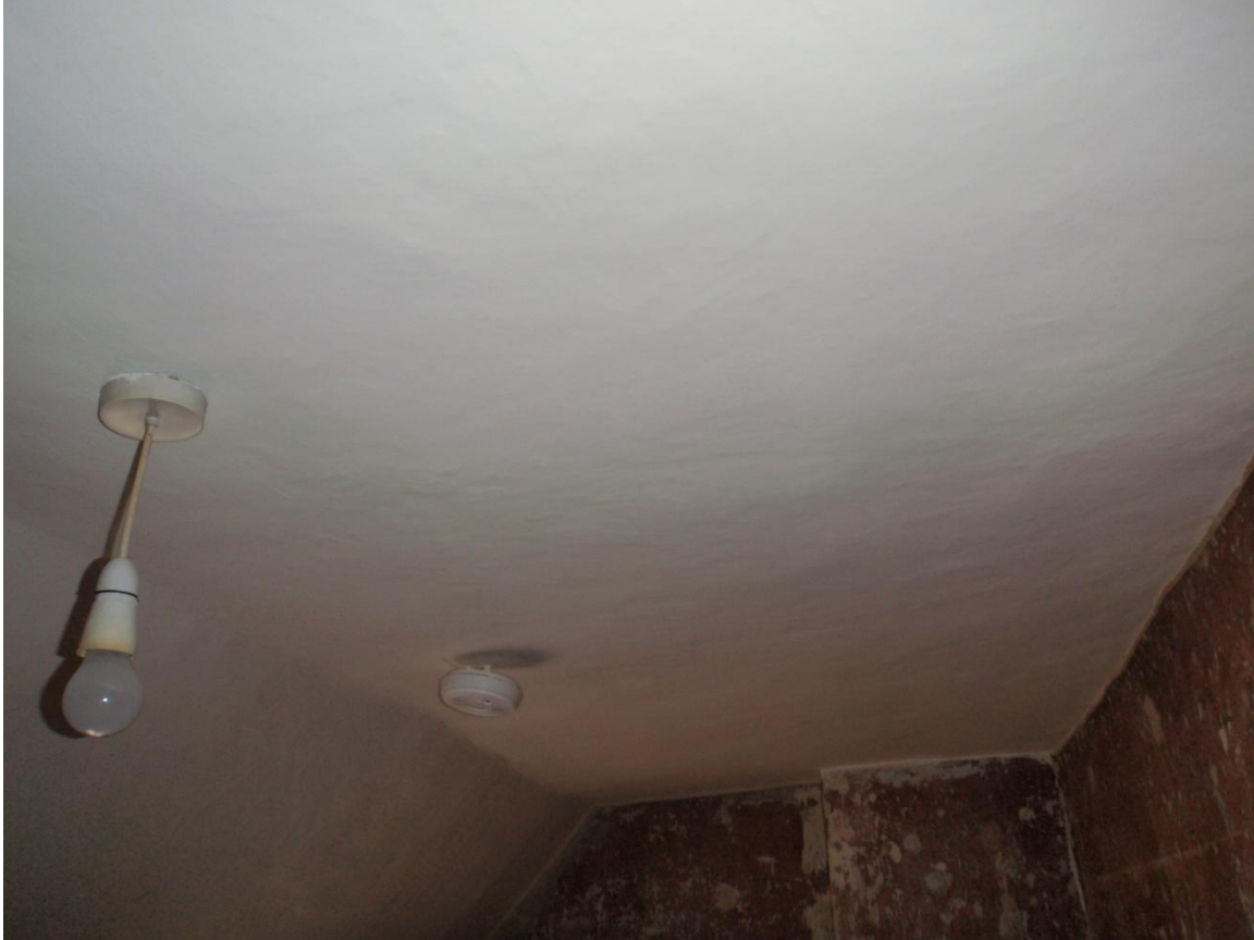
Plate 55: View of the ceiling of the first floor bedroom, from the east
