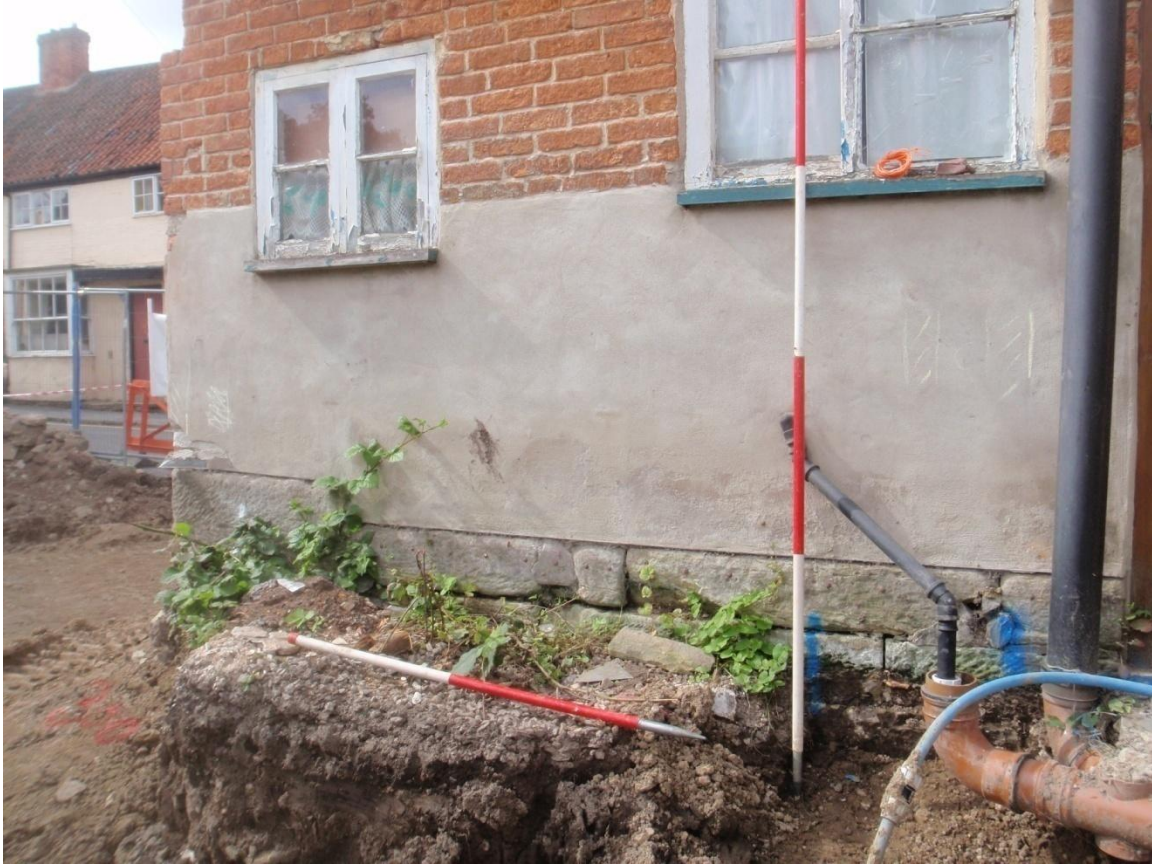
Plate 27: View of the lower levels of the Rear (North) Elevation of 9, Apiary Gate showing the sandstone ashlar foundations exposed by site groundworks, from the north
