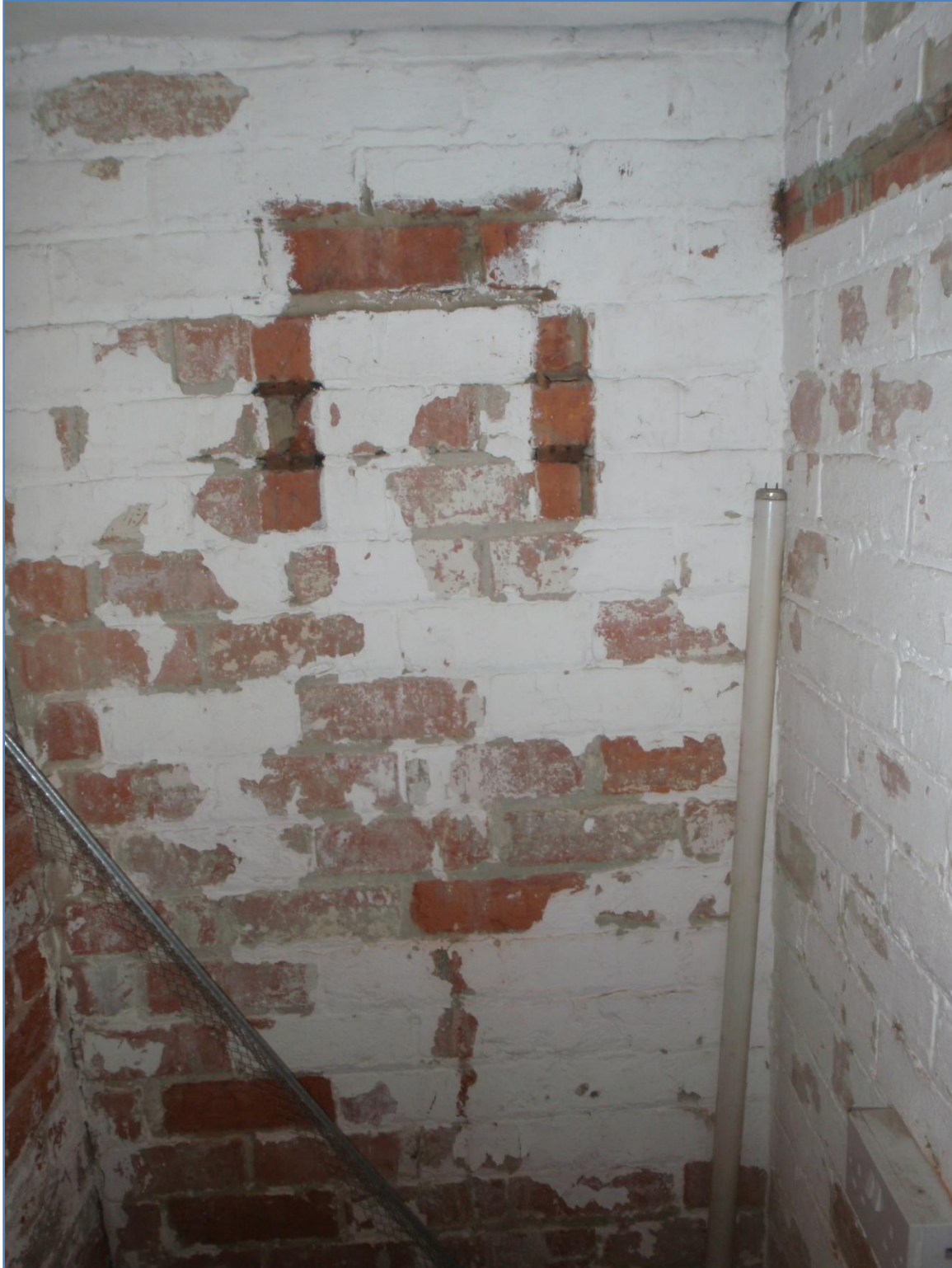
Plate 20: Walls of the first ground floor room of the Side Extension, from the west
