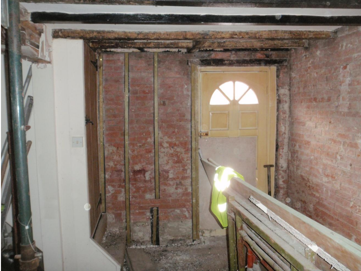
Plate 39: View of the exposed east wall of the ground floor lounge, from the west
