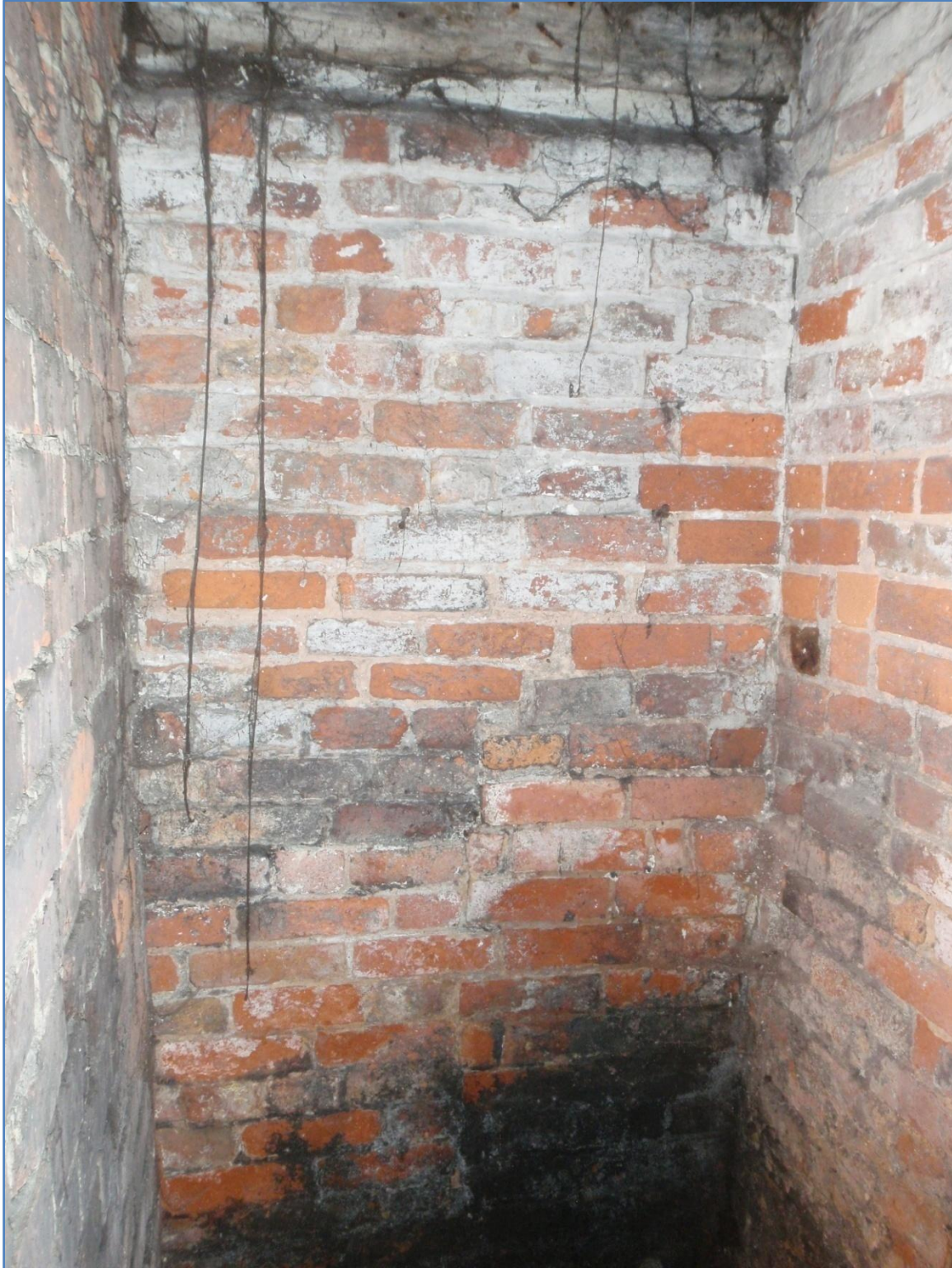
Plate 22: North wall of second ground floor room, Side Extension, from the south
