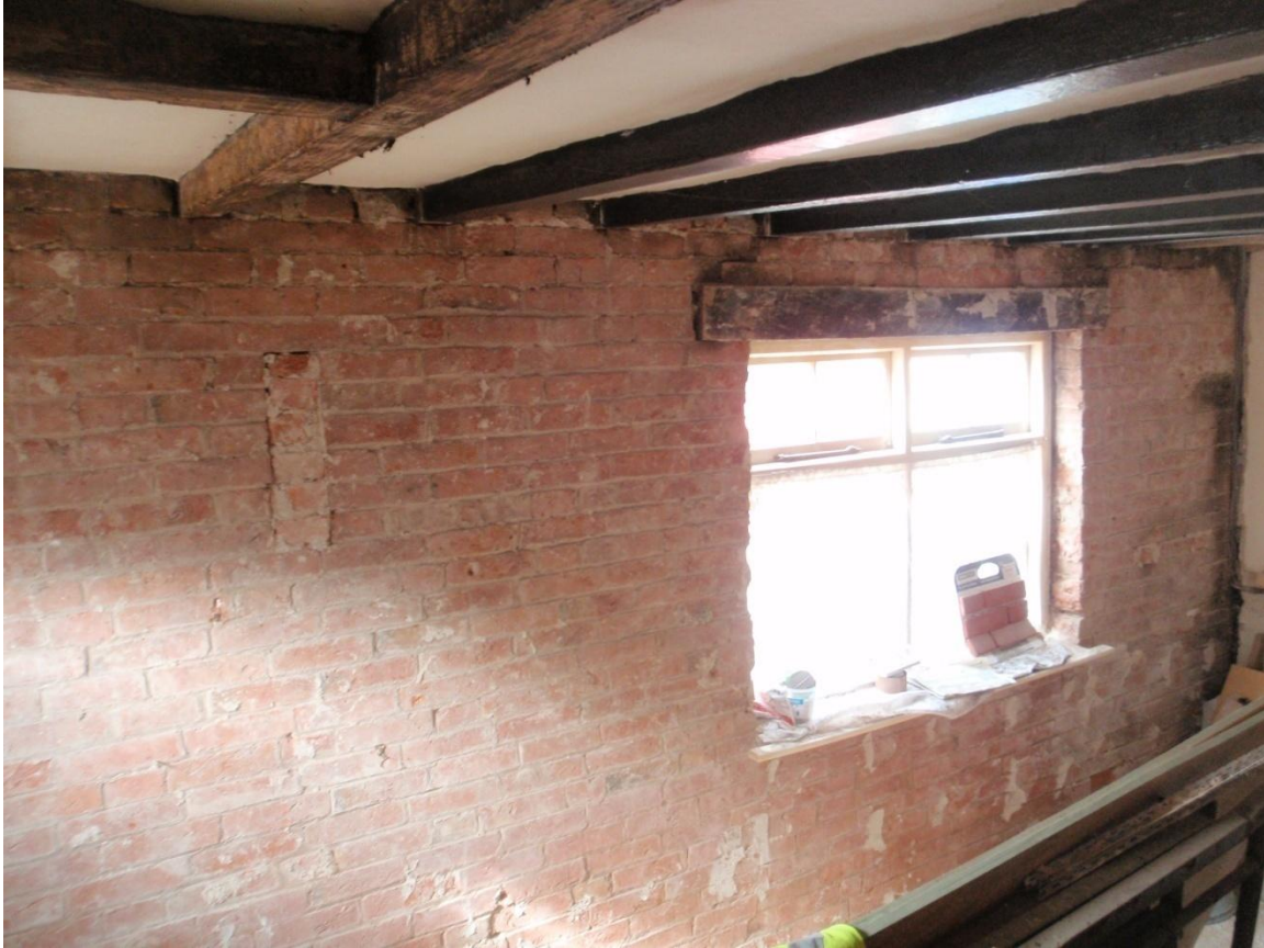
Plate 38: View of the exposed south wall of the ground floor lounge, showing the decorative 'candle' brickwork feature, from the north
