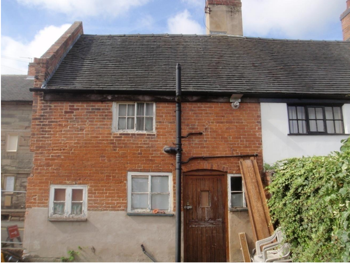
Plate 26: View of the Rear (North) Elevation of 9, Apiary Gate following the demolition of the Side Extension, from the north
