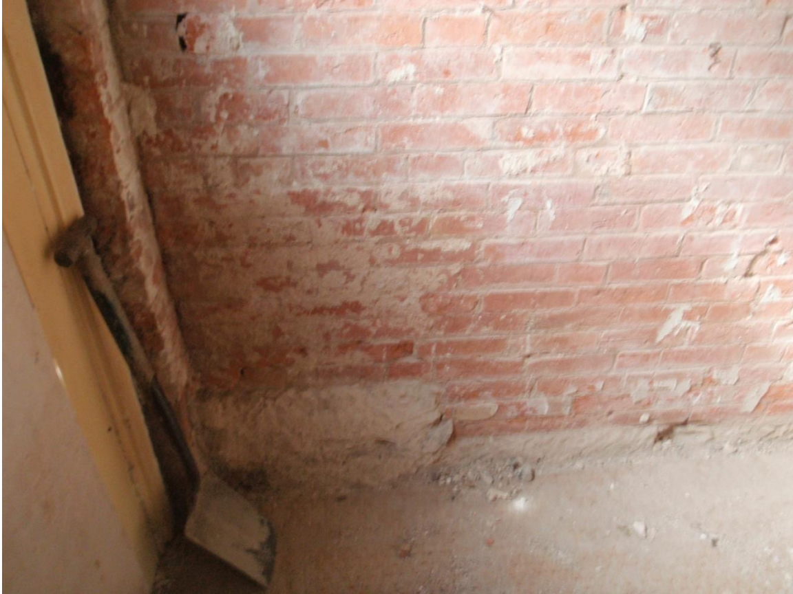
Plate 40: View of the exposed sandstone ashlar foundation in the south wall of the ground floor lounge, from the north
