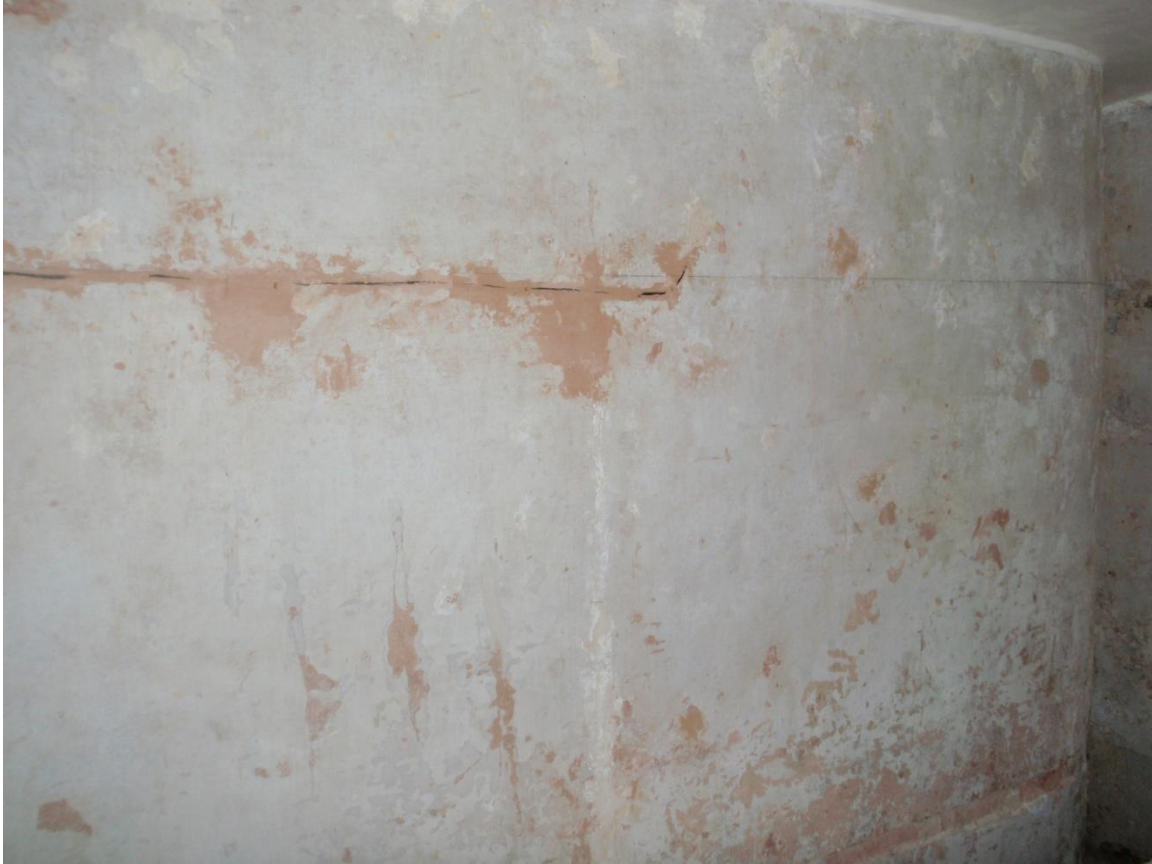
Plate 47: View of the south wall of the first floor bathroom, from the north-east
