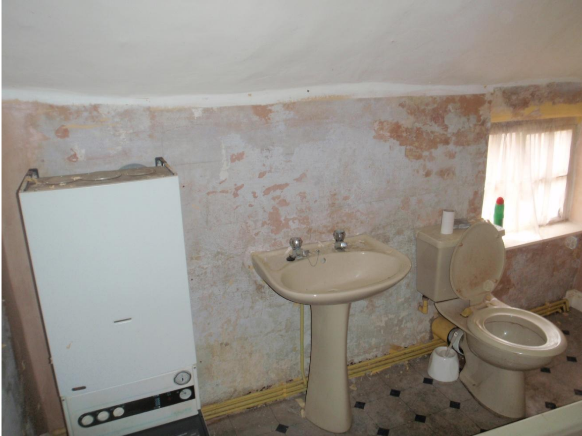
Plate 50: View of the north wall of the first floor bathroom, from the south
