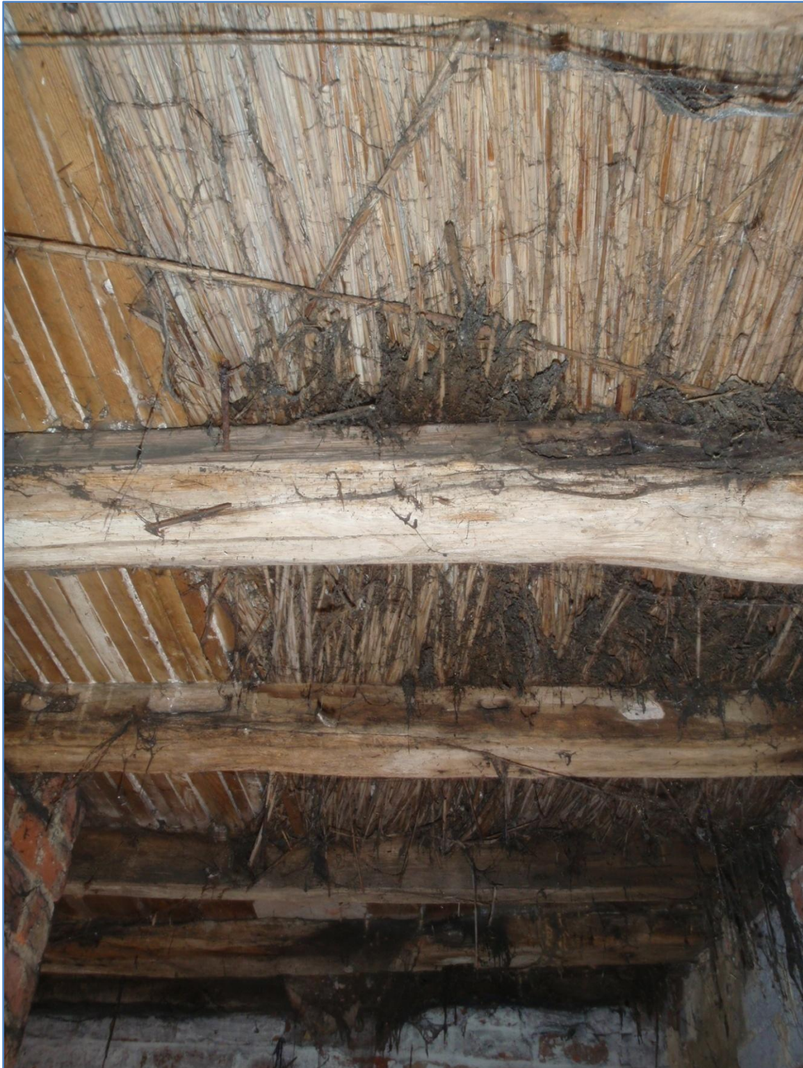
Plate 25: Ceiling of second ground floor room, Side Extension
