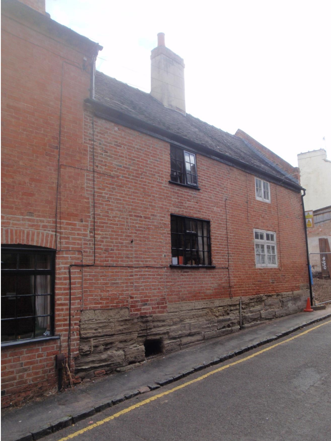
Plate 33: View of the Front (South) Elevation of 9, Apiary Gate, from the south-west
