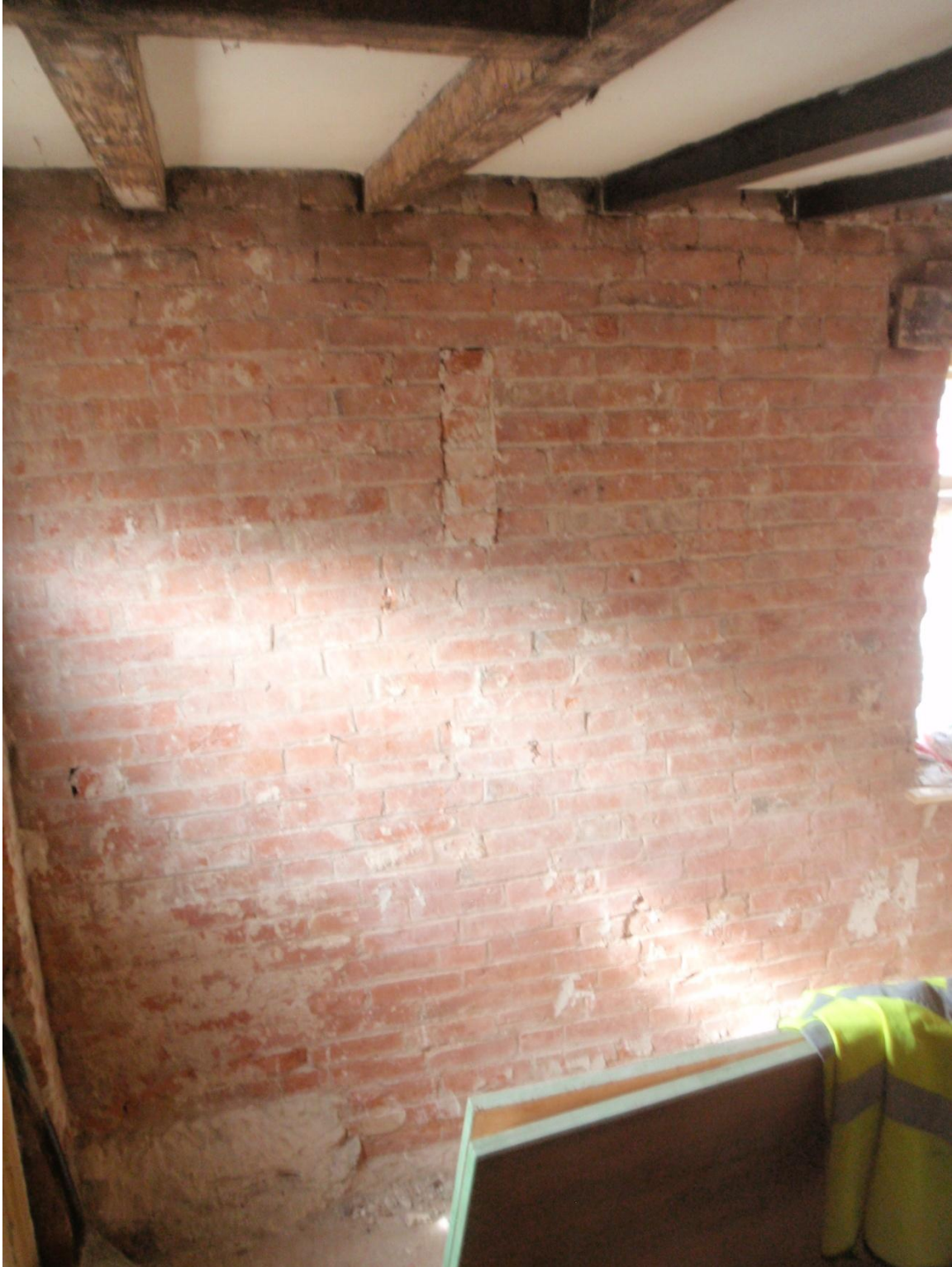
Plate 37: View of the exposed south wall of the ground floor lounge, showing the decorative 'candle' brickwork feature, from the north
