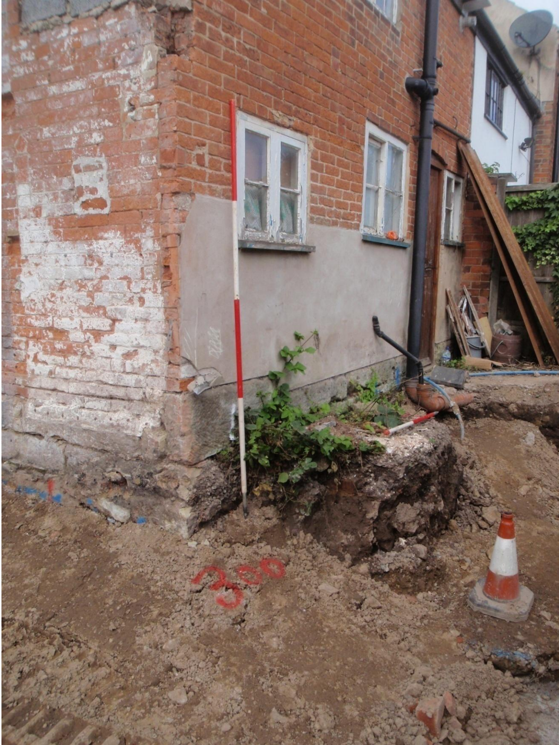
Plate 28: View of the lower levels of the Rear (North) Elevation and of the newly exposed Side (East) Elevation of 9, Apiary Gate, from the east
