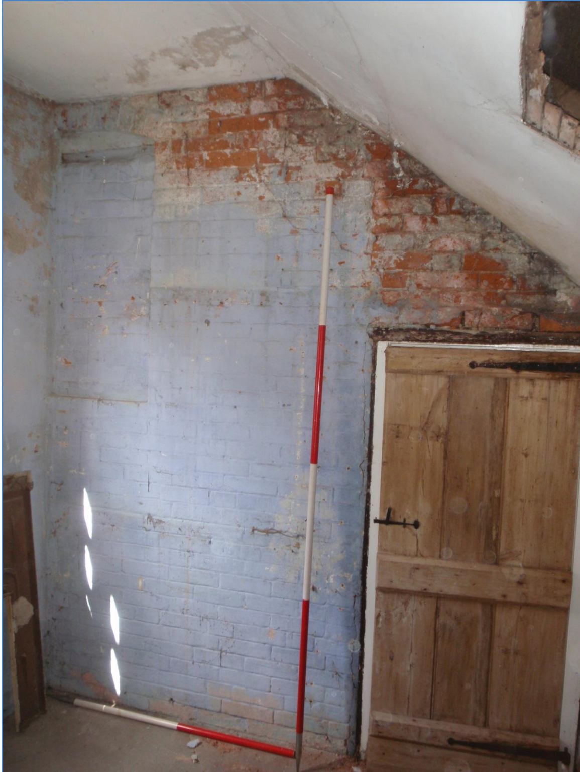
Plate 17: West wall of the first floor interior, Side Extension, from the east
