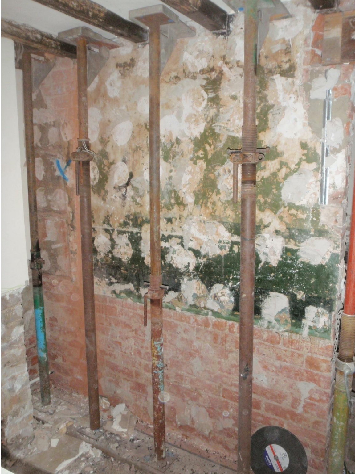
Plate 43: View of the internal partition wall between the ground floor kitchen and lounge, from the south
