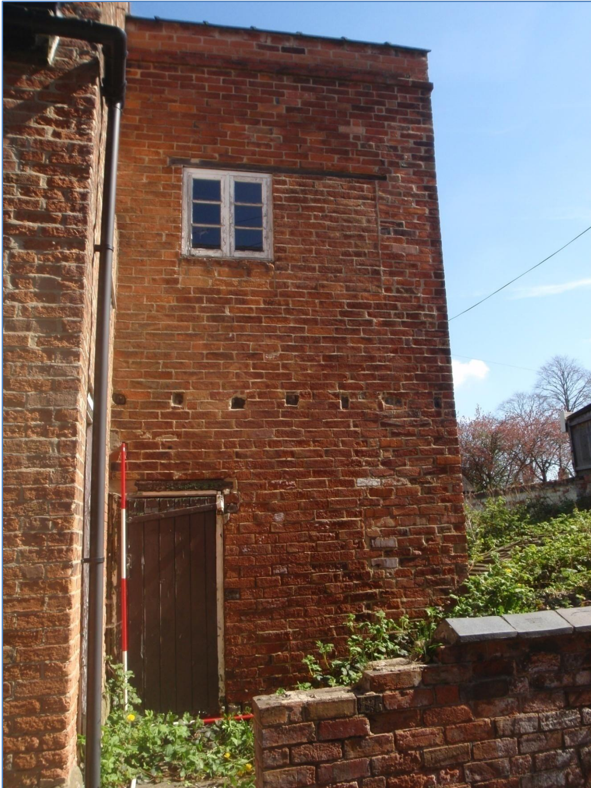
Plate 5: Front (South) Elevation of the Side Extension to 9, Apiary Gate, from the south
