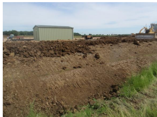
Plate 61: View of the depths of the built up ground levels & the Back-up Generator House, from the south
