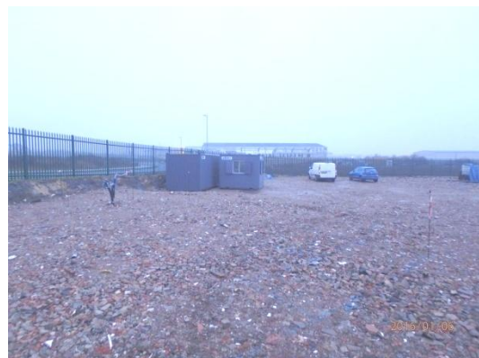
Plate 39: Compacted hardcore over the area of the development site, from the north-west
