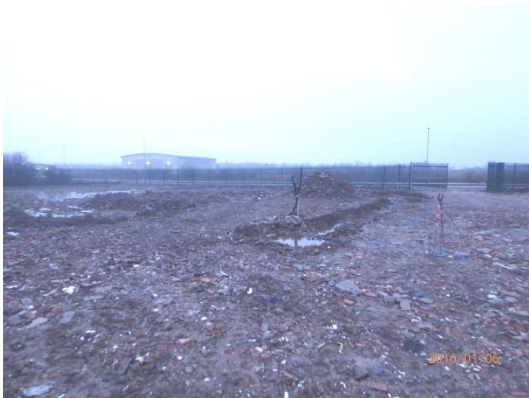
Plate 36: Compacted hardcore over the area of the development site, from the east
