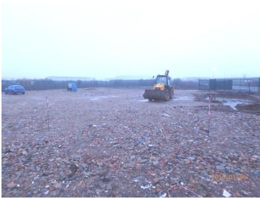
Plate 40: Compacted hardcore over the area of the development site, from the north-east
