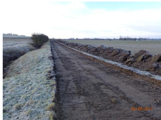
Plate 18: View of the northern end of the strip corridor looking southwards towards Tillbridge Lane, from the north
