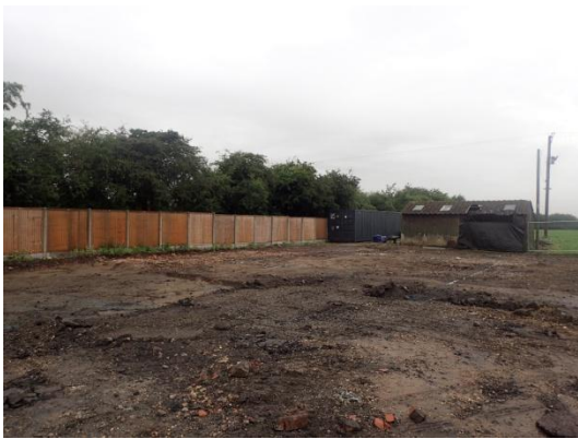
Plate 37: Set out foundations of the new house plot & garage, from the south-east
