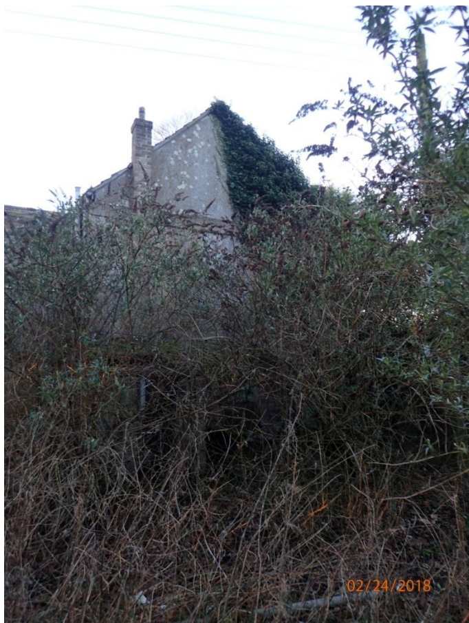
Plate 19: General view of the North Elevation of the Rear Wing of the Farmhouse, from the north
