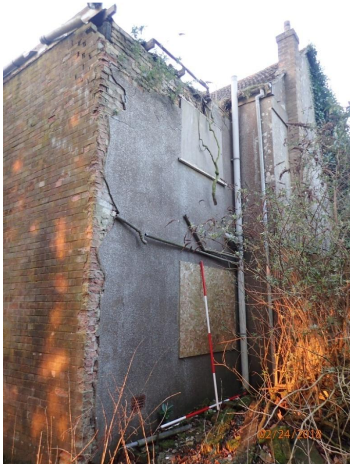
Plate 16: View of the Second North Elevation of the Modern Rear Extension of the Farmhouse, from the east
