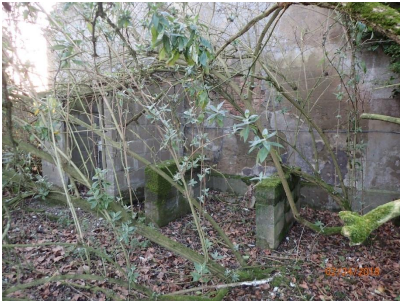
Plate 23: View of the lower levels of the North Elevation of the Farmhouse, from the north
