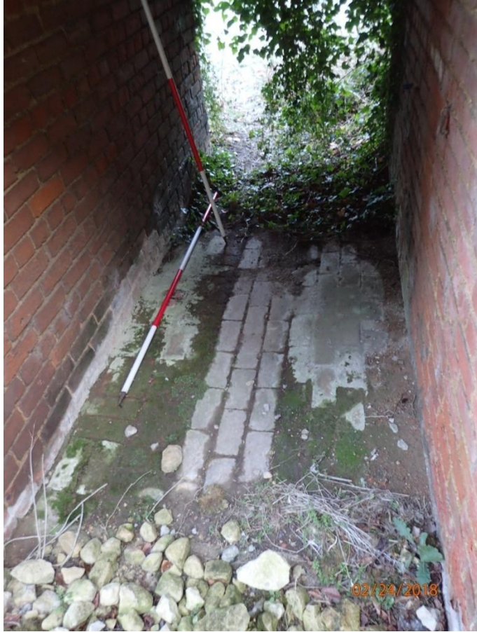
Plate 97: View of the floor of the internal passageway or Cell 6, from the south
