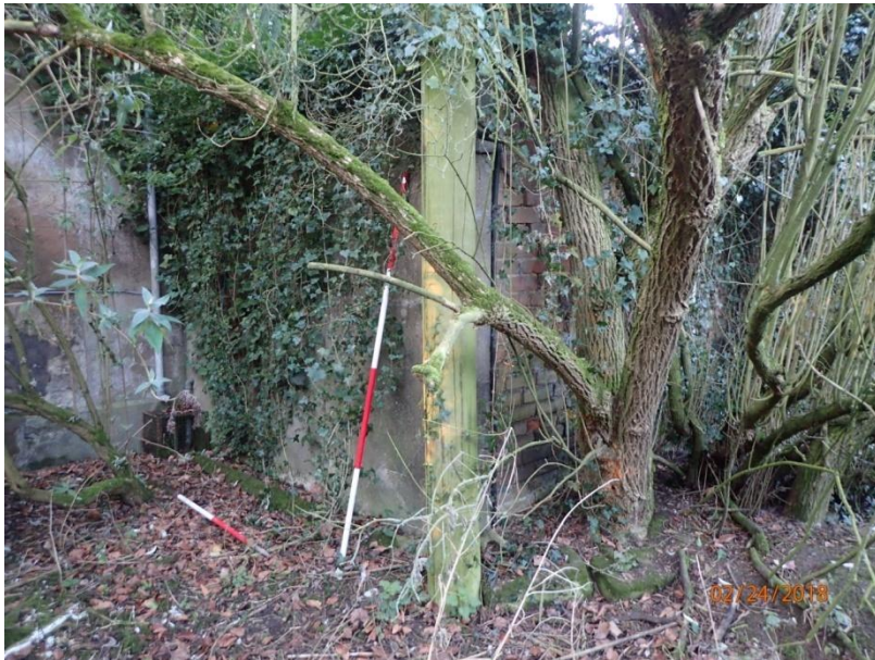
Plate 70: View of the East Elevation and part of the North Elevation of Outbuilding 3, from the north
