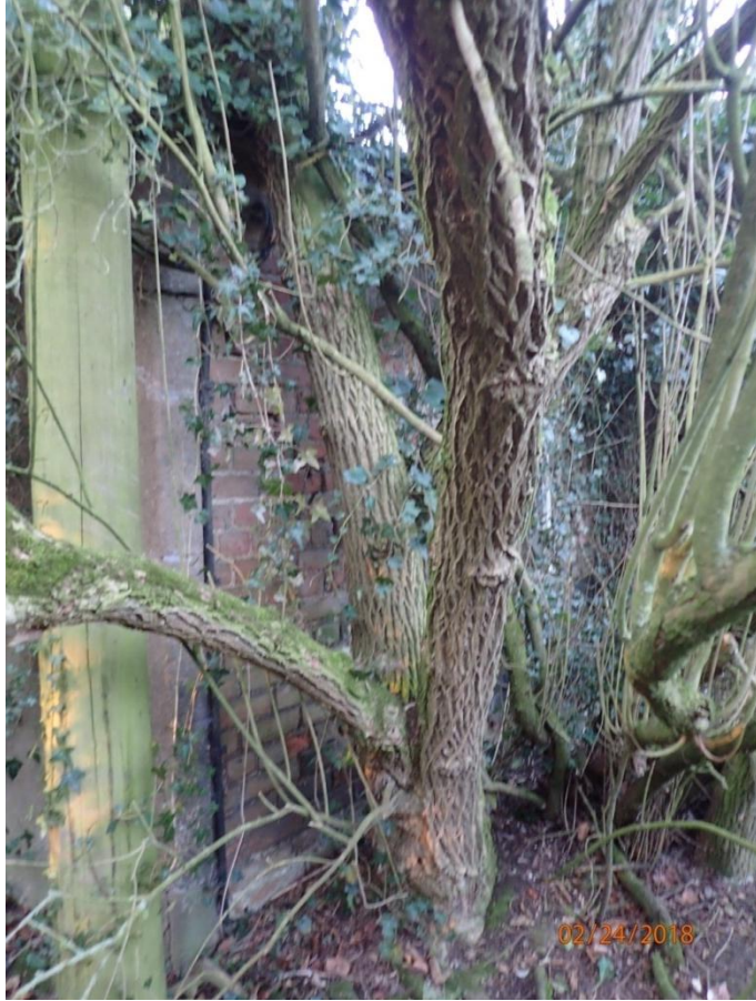
Plate 72: View of part of the North Elevation of Outbuilding 3, from the north
