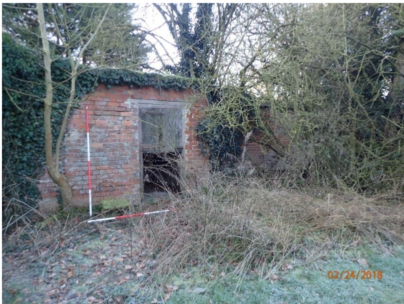
Plate 77: View of part of the North Elevation of Outbuilding 3, from the north
