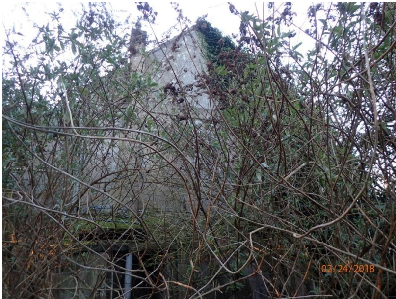
Plate 21: View of the upper levels of the North Elevation of the Farmhouse, from the north
