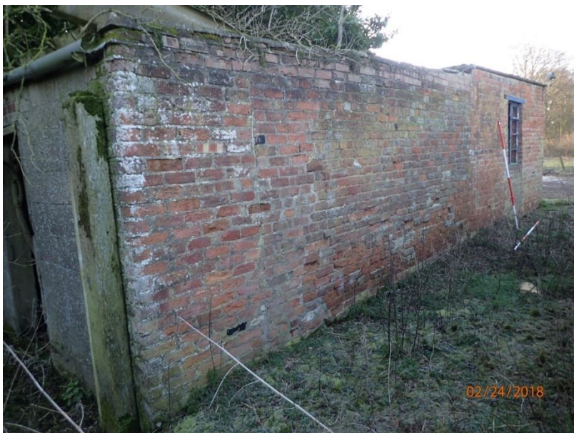
Plate 33: View of the West Elevation of Outbuilding 1, with Outbuilding 2, in the foreground, from the north
