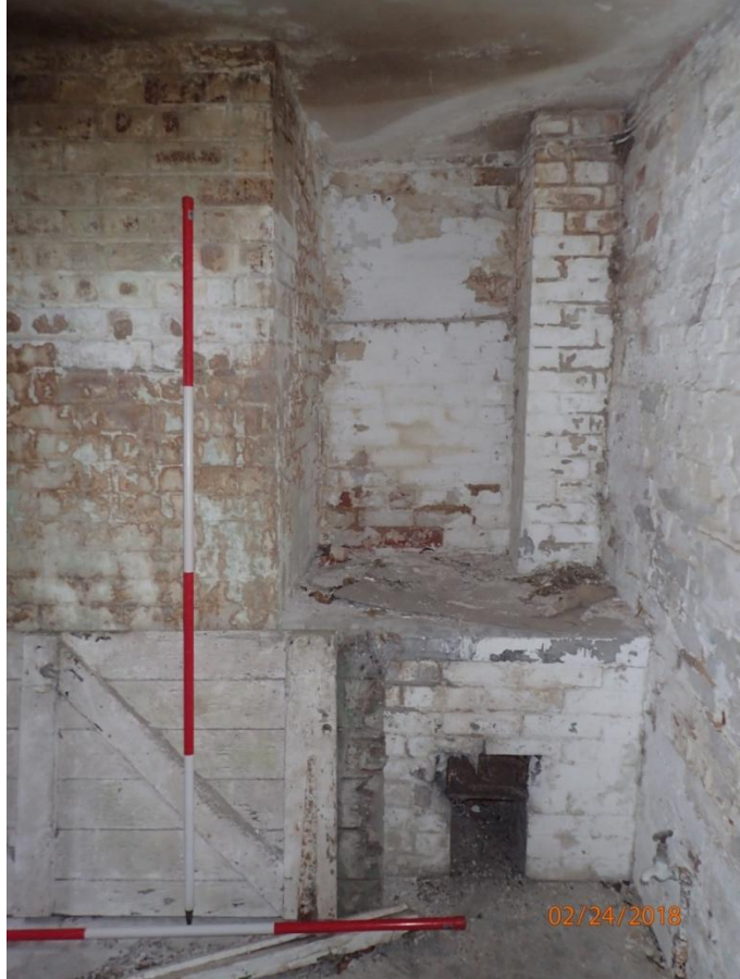
Plate 88: Detail: View of the chimney breast and fireplace in the west wall of Cell 4, from the east
