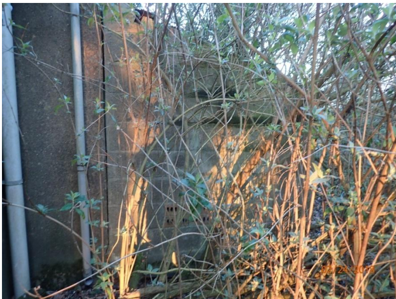
Plate 18: View of the East Elevation of a single storey rear outbuilding to the North Elevation of the Rear Wing of the Farmhouse, from the east
