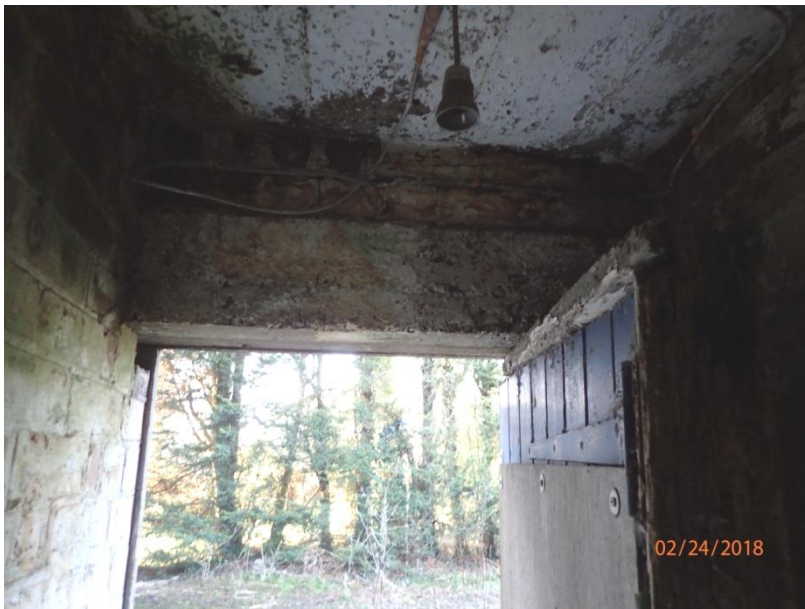
Plate 94: View of the upper levels of the south facing entrance of Cell 5, from the north
