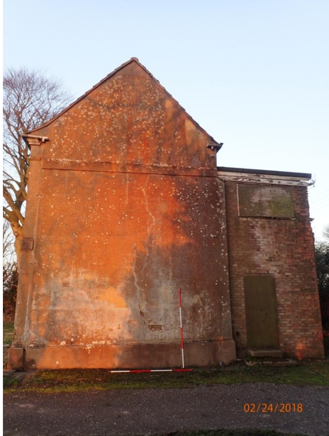
Plate 9: View of the East Elevation of the Farmhouse and adjoining Modern Rear Extension, from the east
