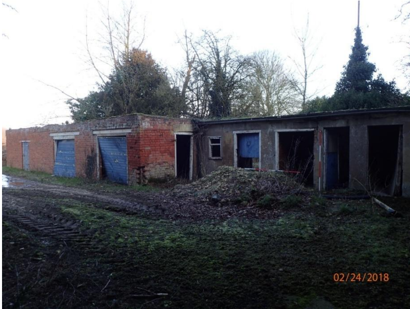
Plate 75: General view of Outbuilding 3 (to the right (east)) and Outbuilding 1 (to the left (west)), from the south
