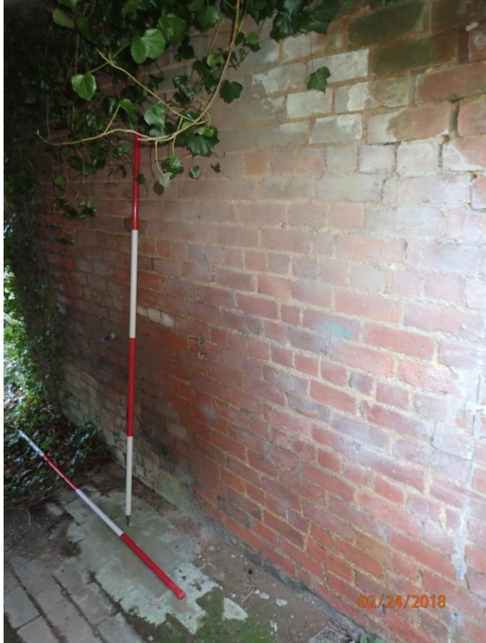
Plate 98: View of the east wall of the internal passageway or Cell 6, from the south
