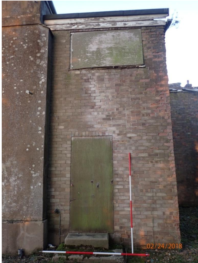
Plate 11: View of the First East Elevation of the Modern Rear Extension to the Farmhouse, from the east
