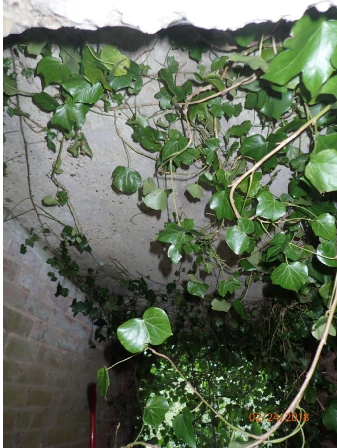
Plate 96: View of the concrete ceiling of the internal passageway or Cell 6, from the south
