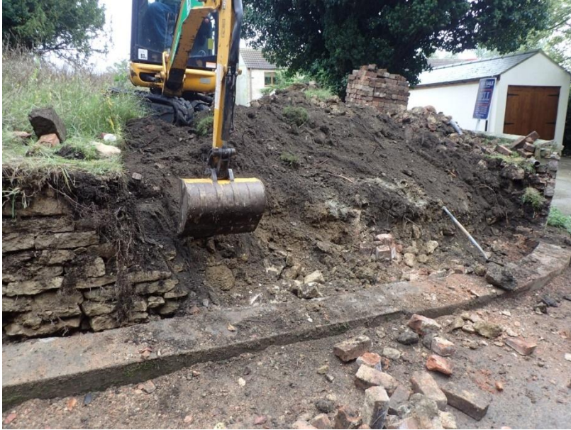
Plate 27: View of the mechanical removal of the earlier mid 19th century churchyard boundary wall, from the west
