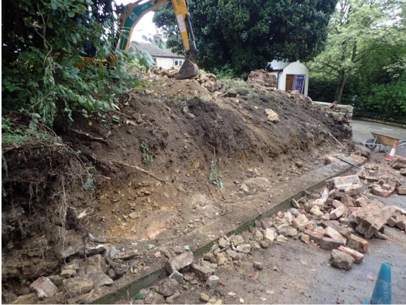
Plate 33: View of the mechanical removal of the earlier mid 19th century churchyard boundary wall, from the north-west
