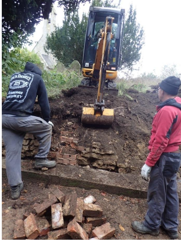
Plate 29: View of the mechanical removal of the earlier mid 19th century churchyard boundary wall, from the west
