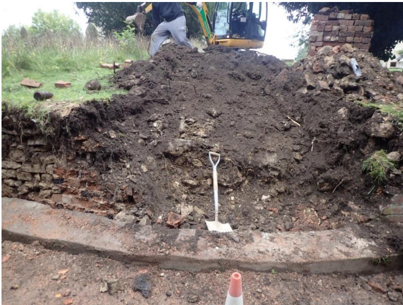
Plate 24: View of the mechanical removal of the earlier mid 19th century churchyard boundary wall, from the west
