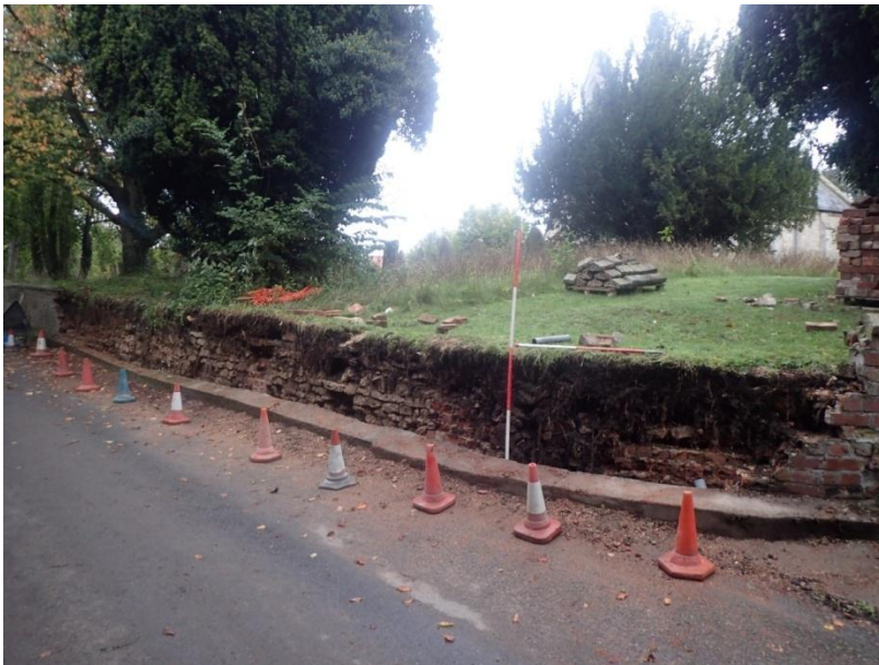
Plate 14: View of the demolished section of current churchyard boundary wall, from the south-west
