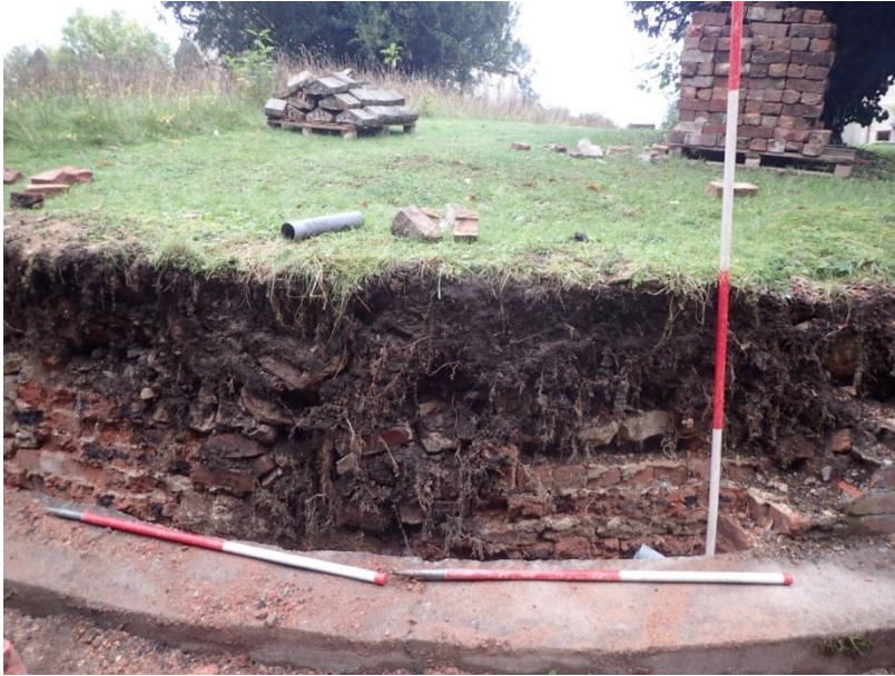
Plate 21: Detailed view of the southern demolished section of current churchyard boundary wall, from the south-west
