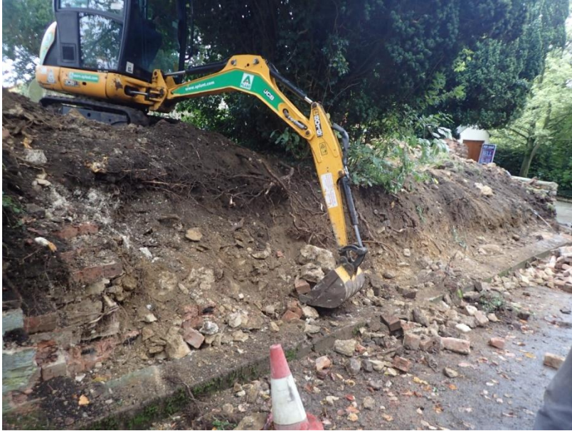
Plate 35: View of the mechanical removal of the earlier mid 19th century churchyard boundary wall, from the north-west
