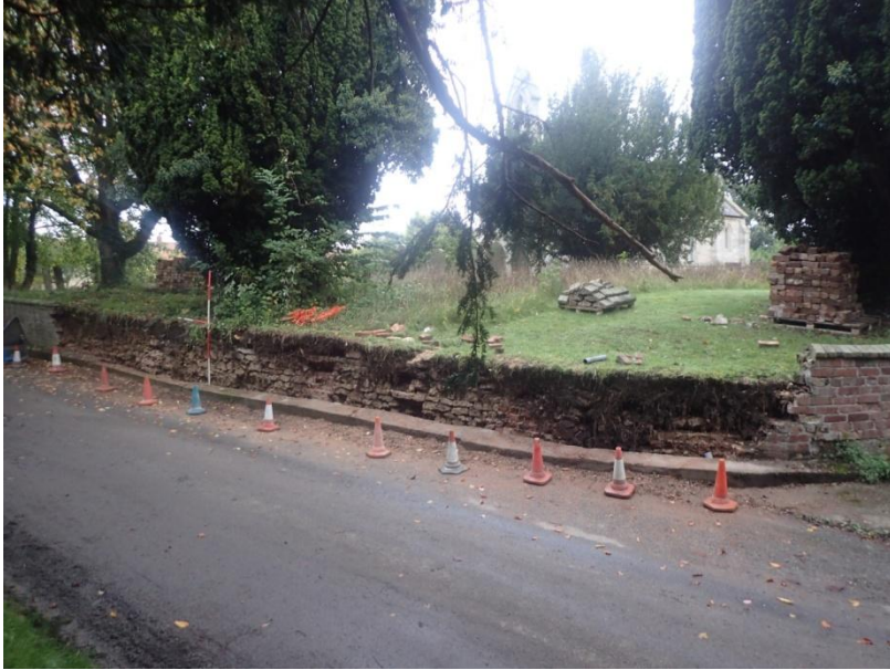
Plate 7: View of the demolished section of current churchyard boundary wall, from the south-west
