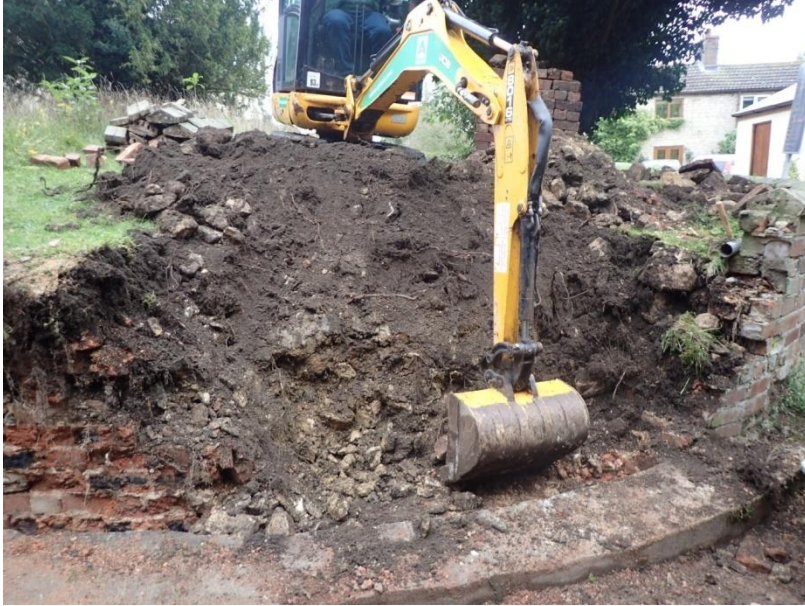
Plate 23: View of the mechanical removal of the earlier mid 19th century churchyard boundary wall, from the west
