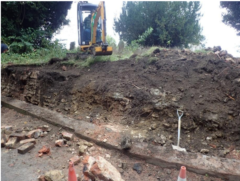
Plate 28: View of the mechanical removal of the earlier mid 19th century churchyard boundary wall, from the south-west
