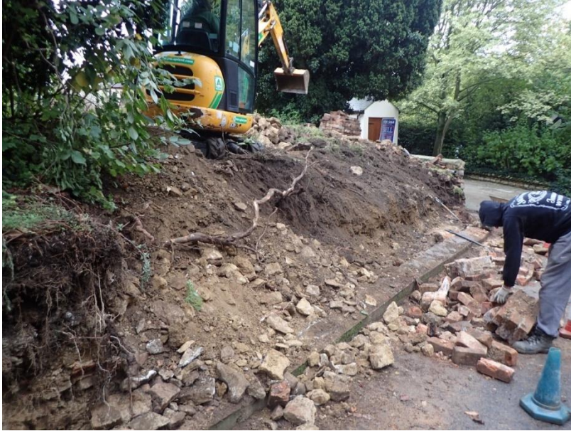
Plate 31: View of the mechanical removal of the earlier mid 19th century churchyard boundary wall, from the north-west
