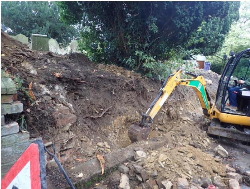
Plate 38: View of the mechanical removal of the earlier mid 19th century churchyard boundary wall, from the north-west
