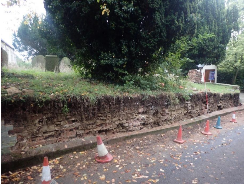
Plate 11: View of the demolished section of current churchyard boundary wall, from the north-west
