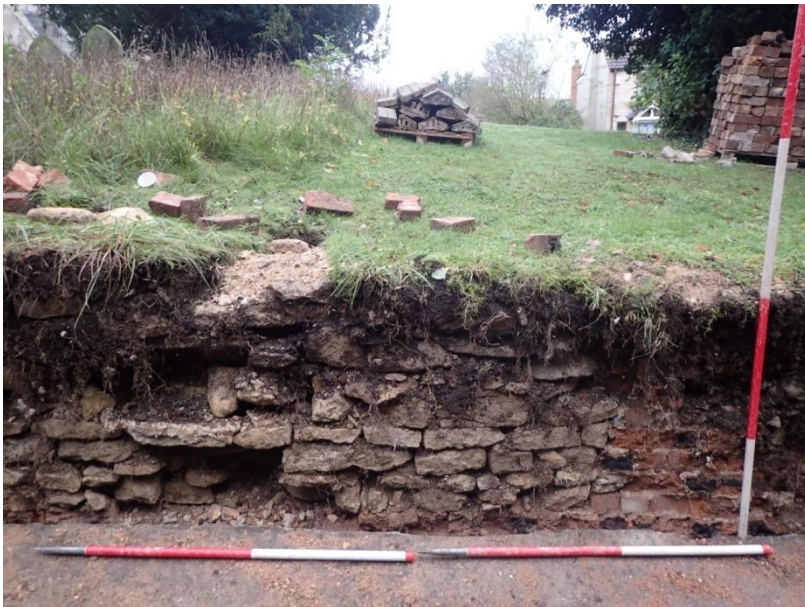
Plate 20: Detailed view of the central demolished section of current churchyard boundary wall, from the west
