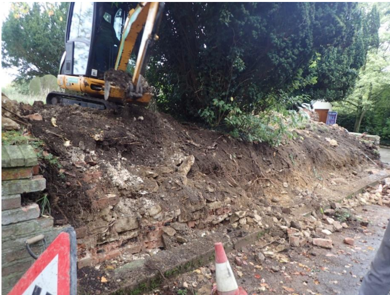
Plate 34: View of the mechanical removal of the earlier mid 19th century churchyard boundary wall, from the north-west
