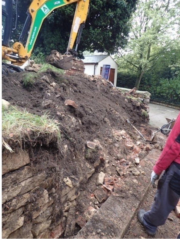
Plate 25: View of the mechanical removal of the earlier mid 19th century churchyard boundary wall, from the north
