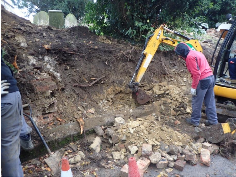
Plate 37: View of the mechanical removal of the earlier mid 19th century churchyard boundary wall, from the north-west
