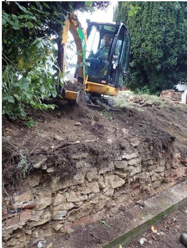
Plate 30: View of the mechanical removal of the earlier mid 19th century churchyard boundary wall, from the north-west
