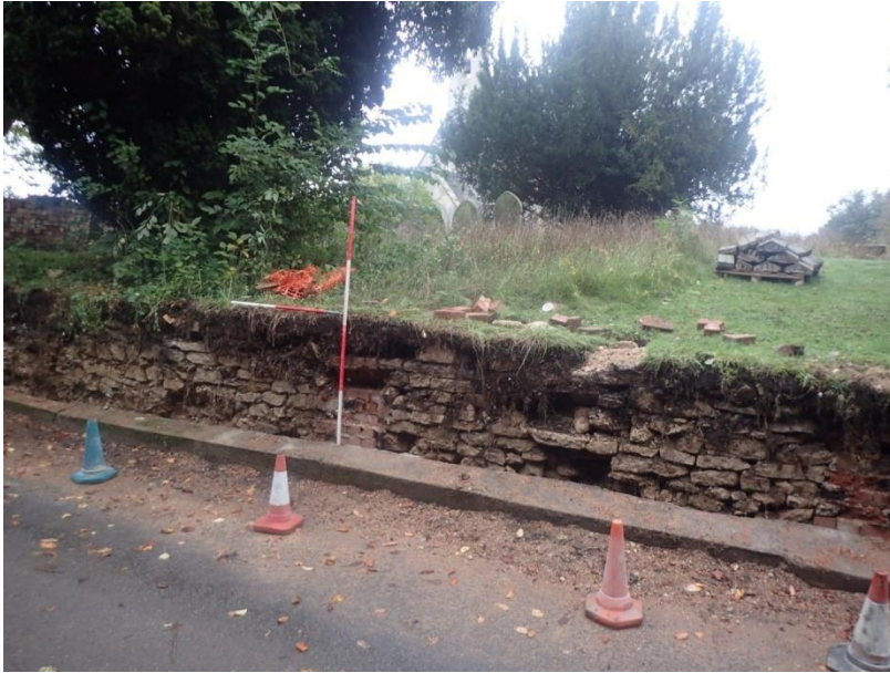
Plate 13: View of the demolished section of current churchyard boundary wall, from the south-west
