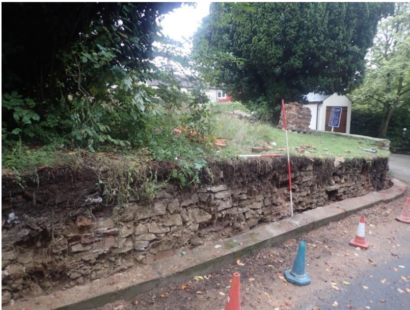
Plate 12: View of the demolished section of current churchyard boundary wall, from the north-west
