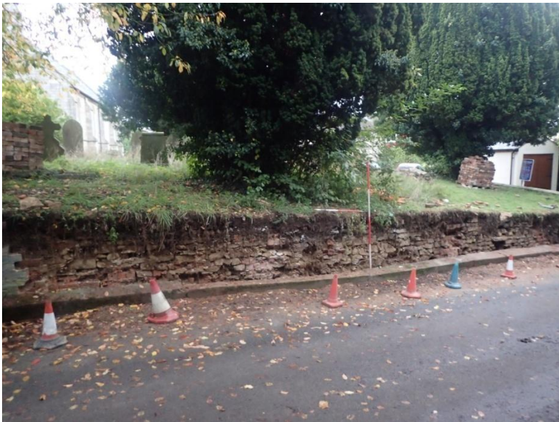
Plate 6: View of the demolished section of current churchyard boundary wall, from the west
