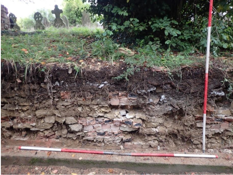
Plate 17: Detailed view of the northern demolished section of current churchyard boundary wall, from the west
