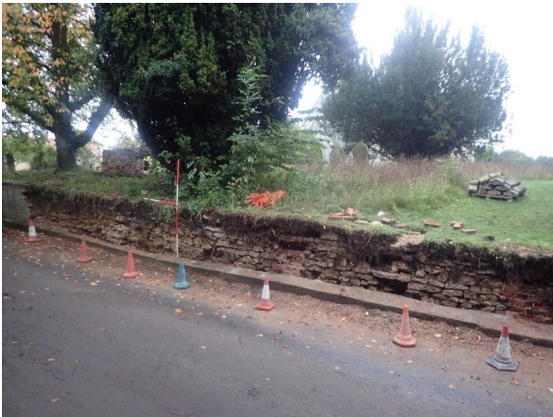
Plate 8: View of the demolished section of current churchyard boundary wall, from the south-west
