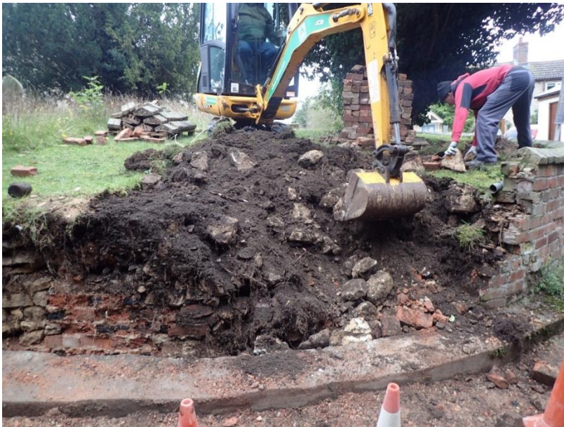
Plate 22: View of the mechanical removal of the earlier mid 19th century churchyard boundary wall, from the west
