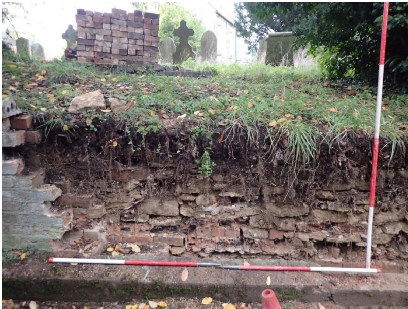
Plate 16: Detailed view of the northern demolished section of current churchyard boundary wall, from the west
