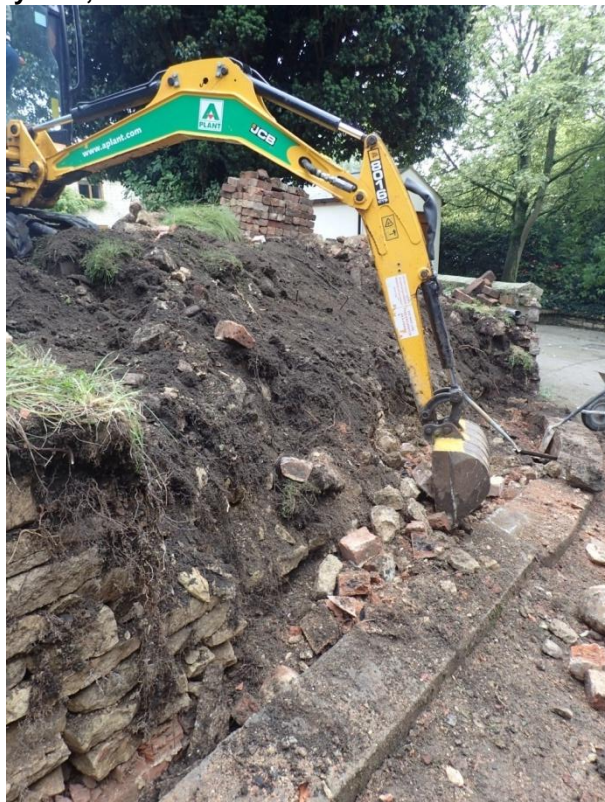
Plate 26: View of the mechanical removal of the earlier mid 19th century churchyard boundary wall, from the north
